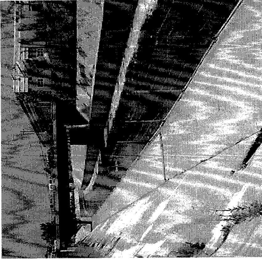
Figure 6b: "Ballona Creek to Estuary" at Duquesne Ave. Fence is meant to keep people out of the creek. Note that the channel walls have become sloped at the top and vertical at the bottom. This change occurs at the beginning of the bike path at National Blvd.
