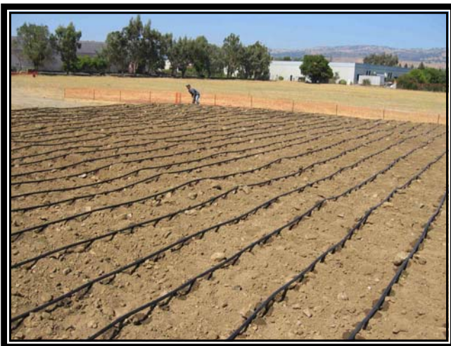
Figure 1 - Ex Situ soil pile with irrigation tubing installed and prior to installation of impermeable cover.
