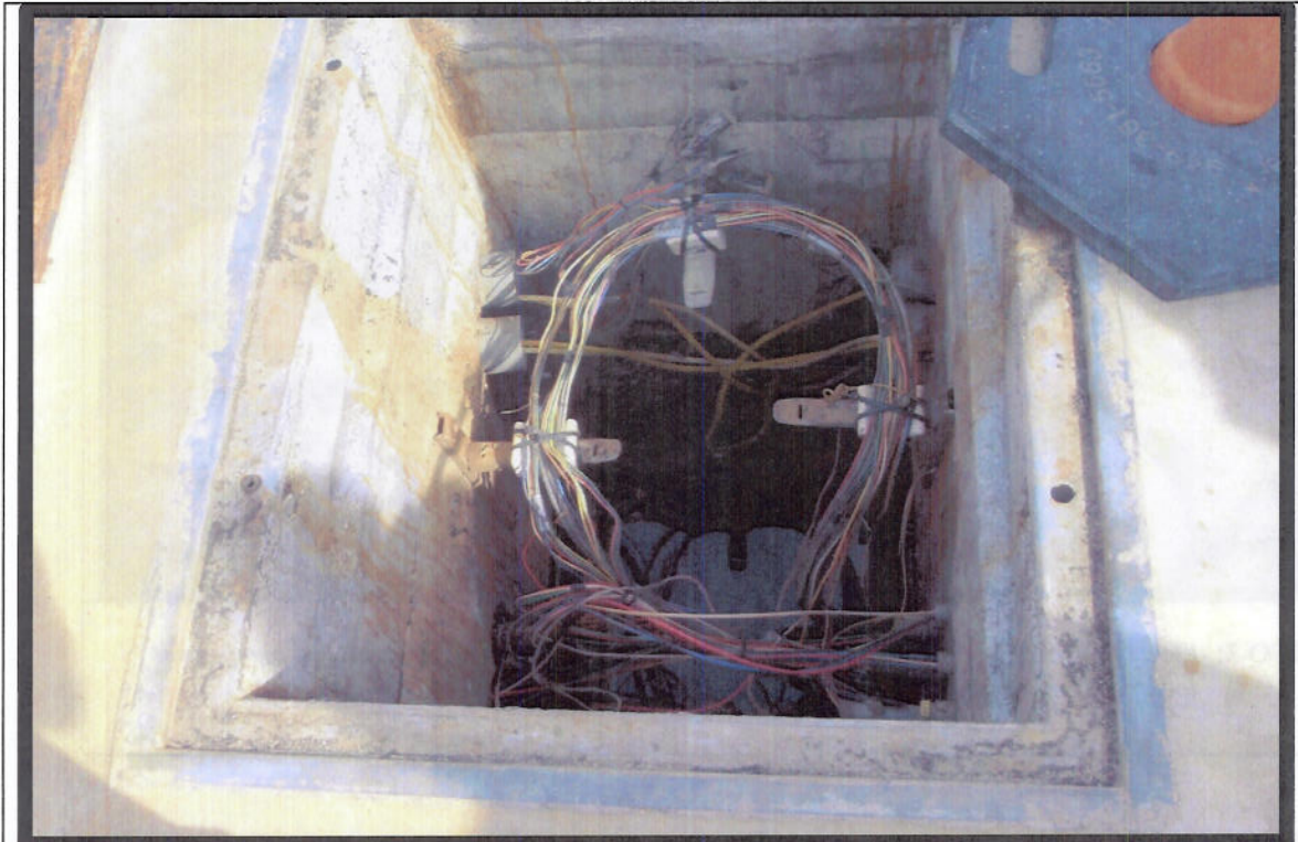
PHOTO 1: View of underground utility box which was inundated with floodwater. After entering the utility box, the floodwater then proceeded into the WWTP influent pump station through electrical conduits, causing the electrical failure and resulting sewer overflow.
