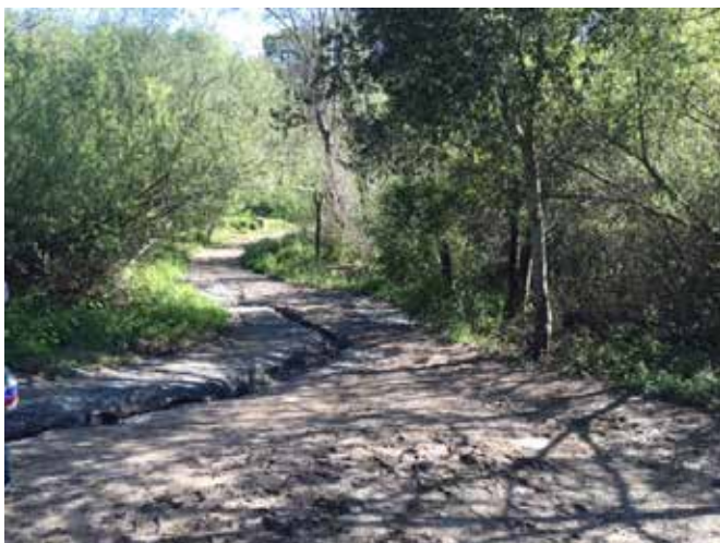
Photo 21 Downcutting observed prior to implementation, on the access road.
