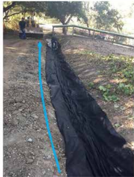
During Photo: Approximate location of 72 linear feet of drainage swale. Gully repair can be seen adjacent and to the right of the blue line. (Direction: Looking West)
