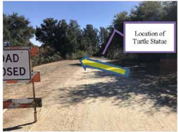
During Photo: Approximate reverse grade dip location 1 (Direction: Looking Southwest)
