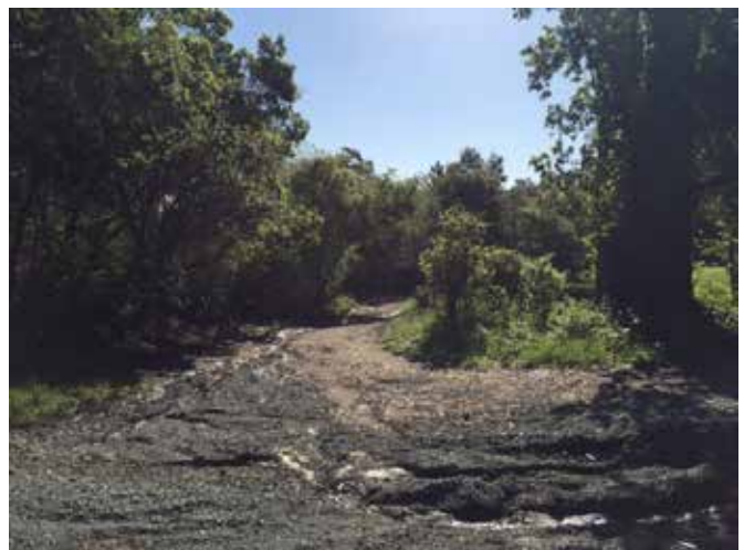
Photo 22 Downcutting and erosion farther up the road from photo 21, on the access road.
