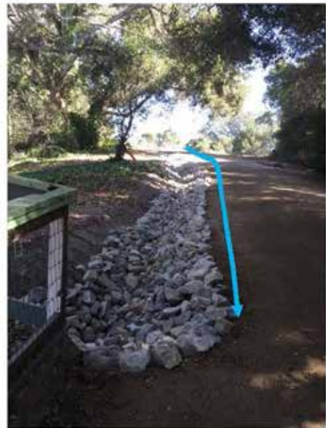
After Photo: Location of 72 linear feet of drainage swale. (Direction: Looking East)
