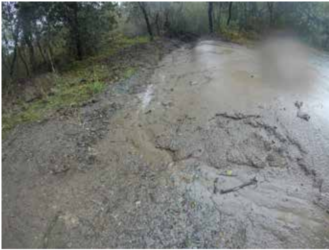
Photo 23 The implemented rolling dips in action, moving water off the access road to inhibit downcutting.
