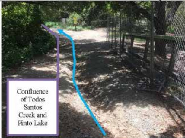
Before Photo: Erosion can be seen on bottom section of road before it drains to lake. Gully can be seen adjacent and to the right of the blue line. (Direction: Looking West)
