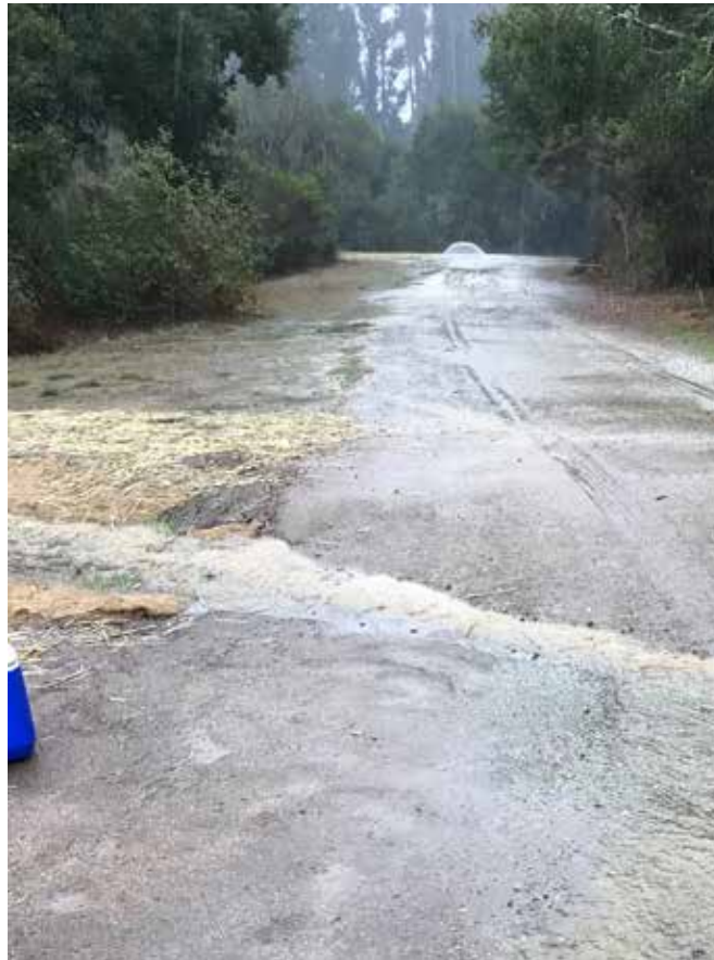
Photo 30 At the first Rolling Dip, on the Virgin Mary Road Improvement Project, during an active storm, November 16, 2017.
