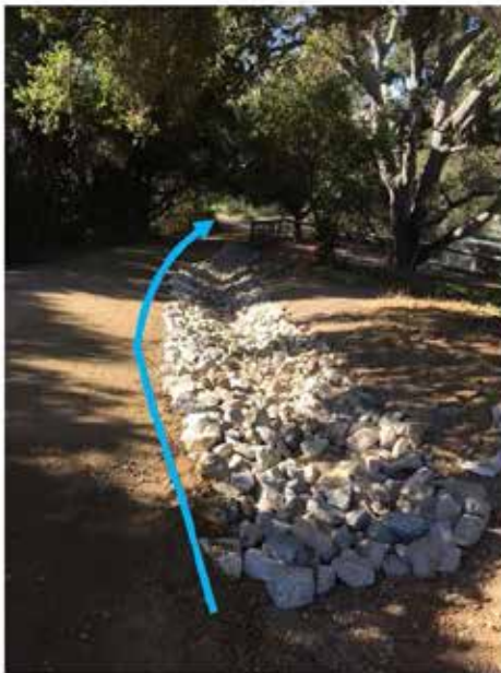
After Photo: Location of 72 linear feet of drainage swale. (Direction: Looking West)
