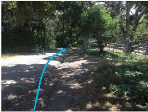
Before Photo: Approximate location of 72 linear feet of drainage swale. Gully can be seen adjacent and to the right of the blue line. (Direction: Looking West)
