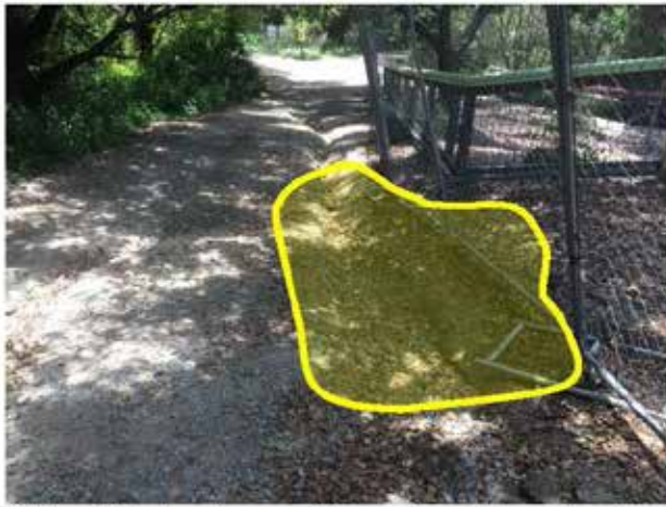
Before Photo: Approximate location of culvert inlet to transport water under the road. Gully can be seen adjacent and to the right of the blue line. (Direction: Looking West)
