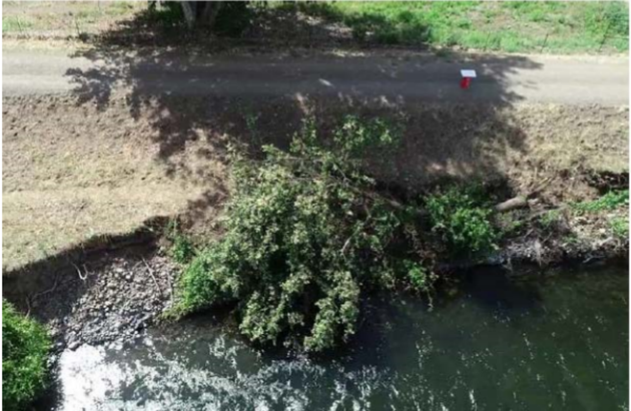
Figure 2: Extent of levee erosion at Deer Creek
