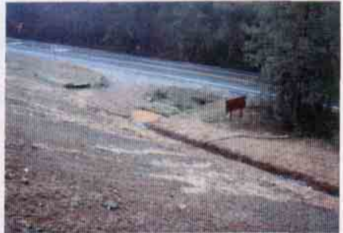
Figure 8: Partially protected slope Note: the turbid discharge leaving the site which flows directly under the roadway and into the creek
