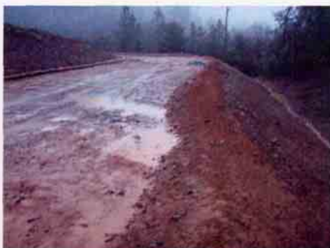
Figure 6: Lack of an effective combination of erosion and sediment control BMPs
