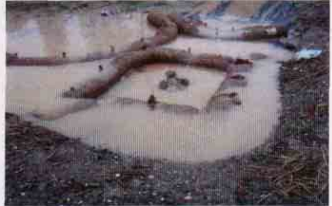
Figure 20: Pondered storm water around another drain inlet
