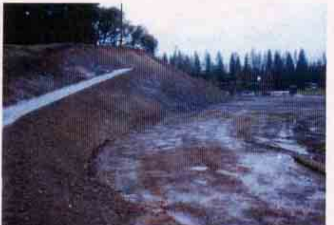
Figure 12: Lack of an effective combination of erosion and sediment control BMPs
