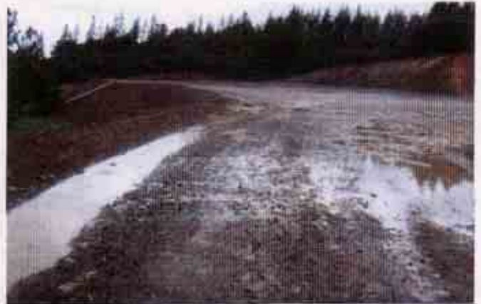
Figure 32: Lack of an effective combination of erosion and sediment control BMPs
