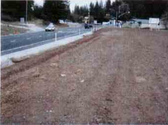
Figure 13: : Poor erosion control BMPs
