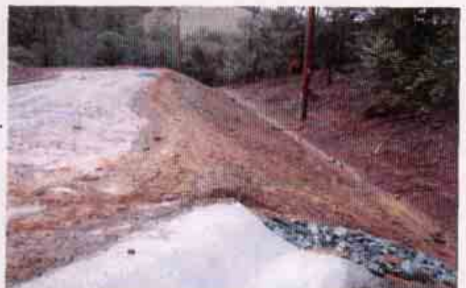
Figure 12: Area where concrete drain along the slope discharges into the area that flows down to the western discharge location. Note: the lack of BMPs other than rip-rap
