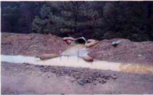
Figure 13: Inadequate BMPs at a location where storm water flows from the site into a down drain which directly flows under the roadway and into the creek
