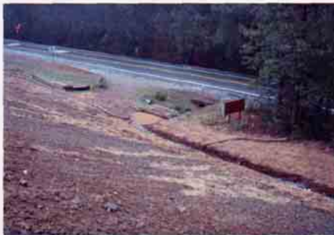
Figure 8: Partially protected slope Note: the turbid discharge leaving the site which flows directly under the roadway and into the creek
