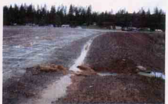
Figure 20: Lack of an effective combination of erosion and sediment control BMPs Note: the discharge into the down drain and the lack of effective BMPs prior to the down drain
