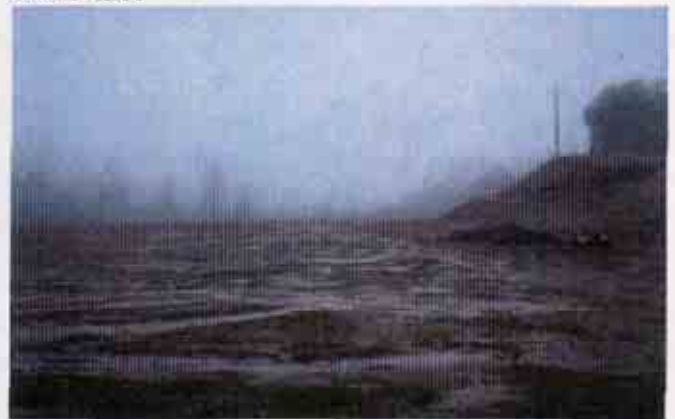
Figure 22: Lack of an effective combination of erosion and sediment control BMPs on another portion of the project
