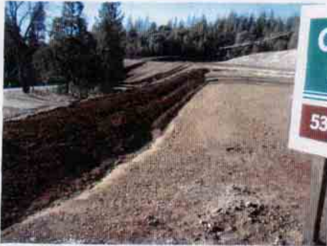
Figure 7: Lack of an effective combination of erosion and sediment control BMPs
