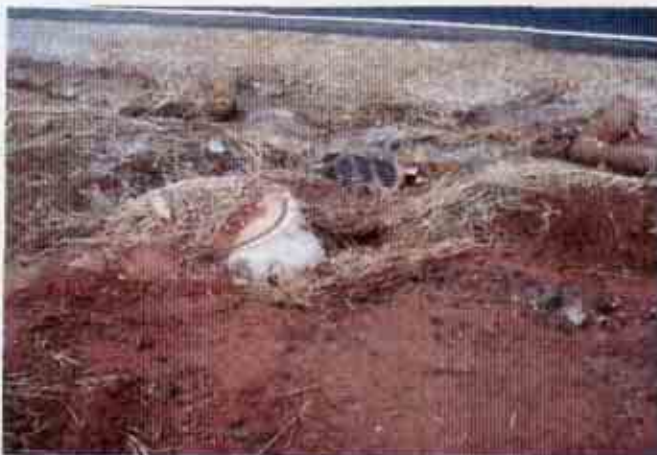
Figure 11: Another view of the protected drain inlet
