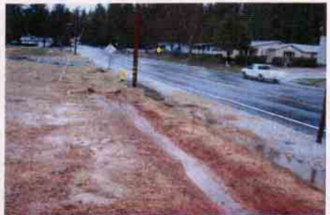
Figure 28: Sediment laden storm water flowing down to the drain inlet adjacent to Ridge Road
