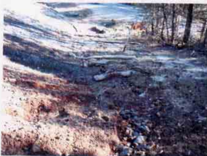
Figure 5: Poorly installed and maintained BMPs
