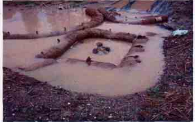
Figure 20: Pondered storm water around another drain inlet
