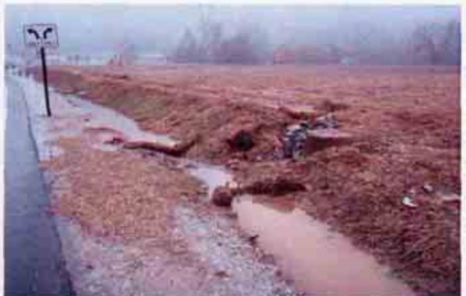
Figure 18: Another view of the poorly protected drain inlet
