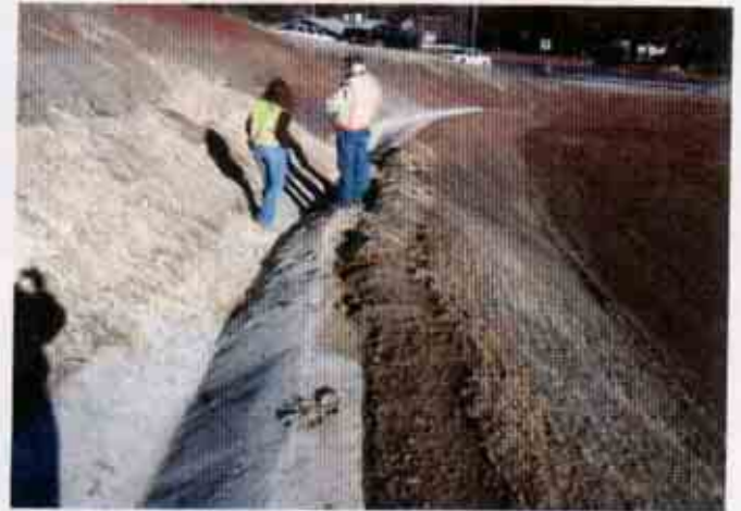
Figure 2: Erosion on the steep cut slope on the development
