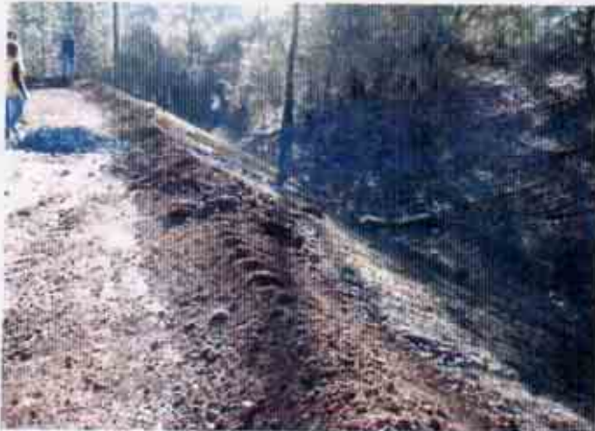
Figure 3: Another area that is poorly protected
