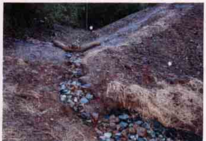
Figure 6: Area above the western discharge location where staff observed no effective storm water management BMPs
