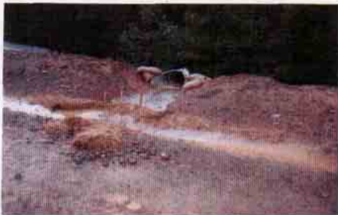
Figure 17: Fiber rolls installed prior to turbid stormwater discharge into the down drain
