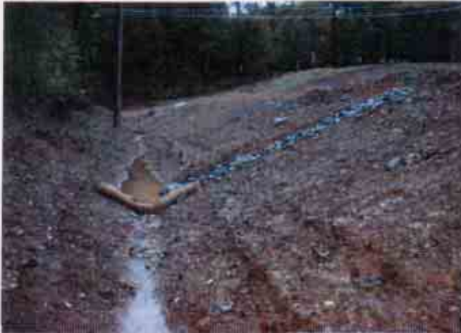
Figure 9: Area above the discharge location in Figure 8 Note: the lack of erosion control BMPs
