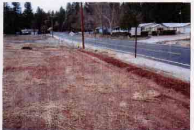
Figure 12: : Poor erosion control BMPs
