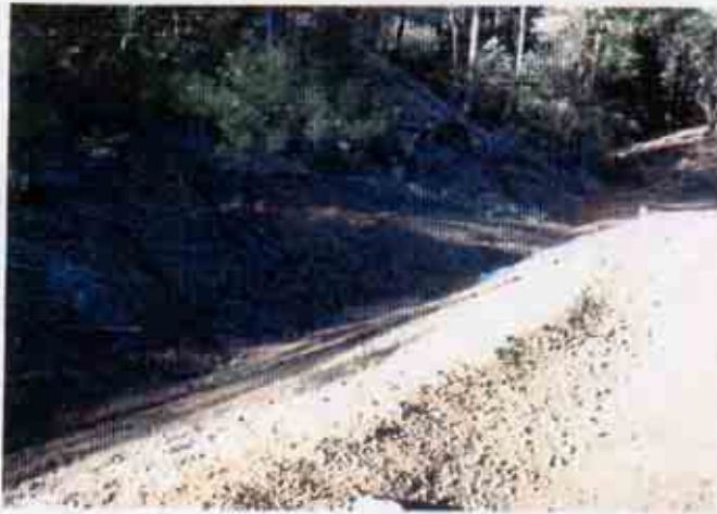
Figure 1: Area on the construction site that has not been effectively stabilized
