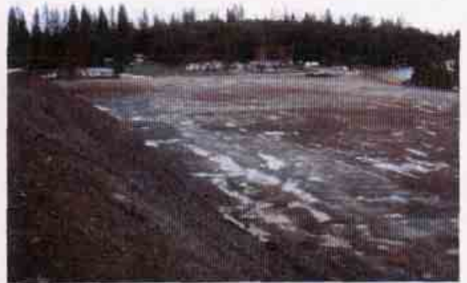
Figure 14: Lack of an effective combination of erosion and sediment control BMPs
