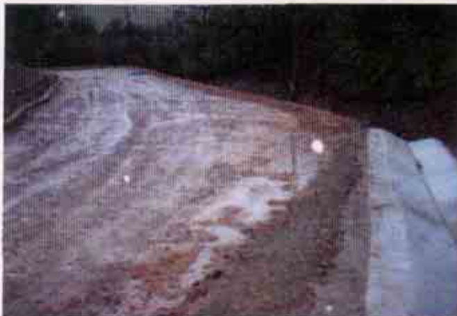
Figure 11: General lack of BMPs above the area in Figure 9
