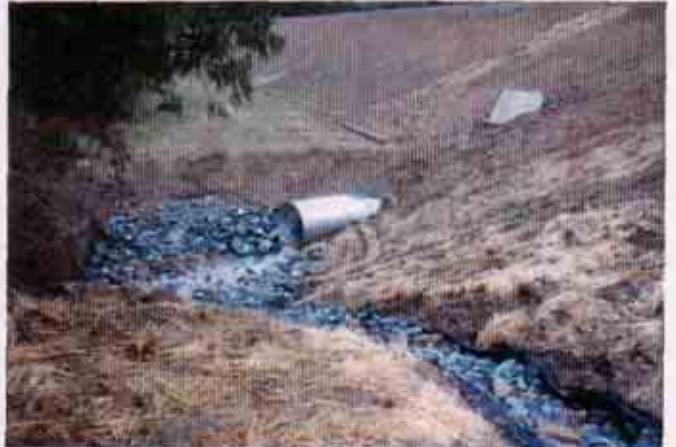
Figure 4: Turbid storm water discharging into the eastern culvert
