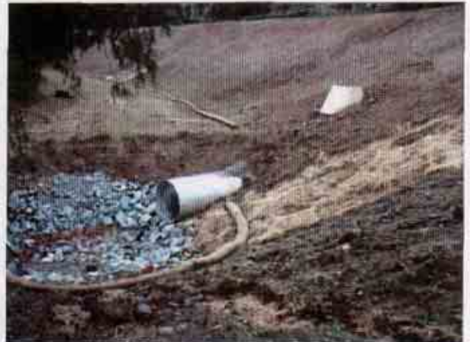
Figure 2: Poor BMPs directly around a outfall location
