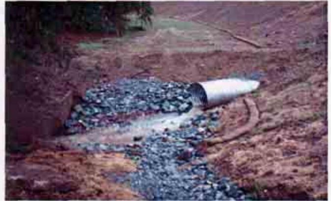
Figure 10: Turbid discharge from the project flowing from the eastern culvert.
