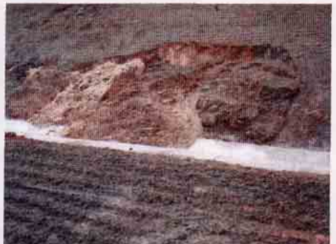
Figure 6: Slump that has deposited sediment in the concrete lined storm water conveyance system
