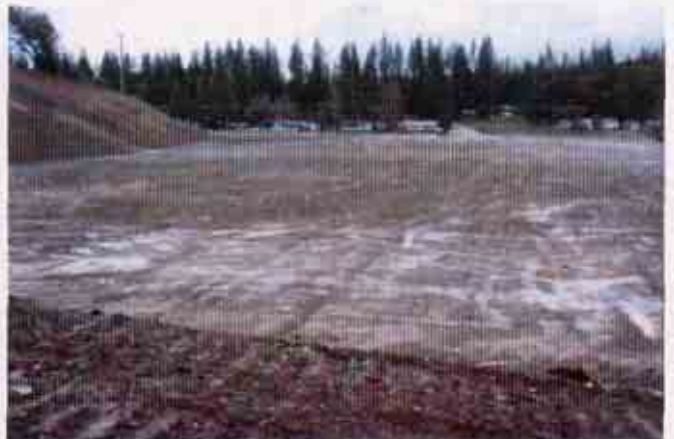
Figure 28: Lack of an effective combination of erosion and sediment control BMPs
