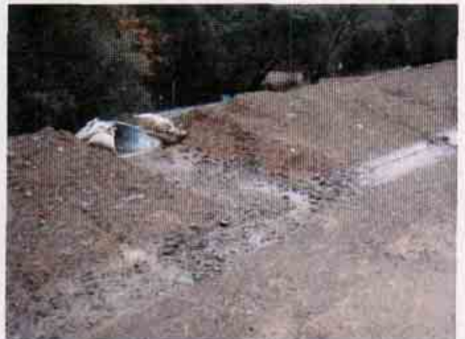
Figure 4: Poorly protected down drain inlet
