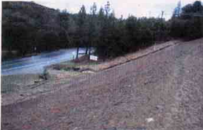
Figure 19: Poorly protected slope
