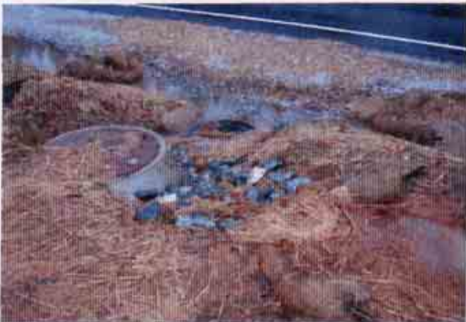
Figure 29: Turbid storm water flowing into the drain inlet along Ridge Road
