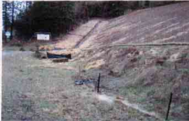
Figure 7: Storm water in the Caltrans right-of-way flowing to the western discharge location
