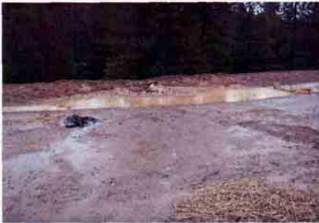
Figure 7: Turbid storm water sheet flowing to a culvert which conveys storm water down slope.
