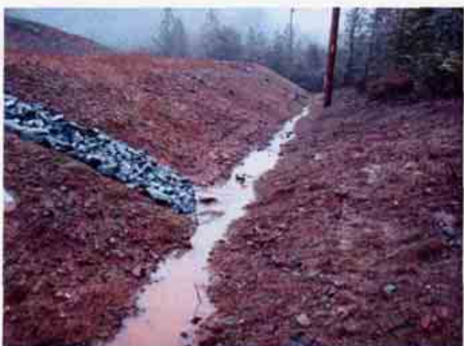
Figure 5: Lack of effective BMPs on the slopes and lack of BMPs in a defined drainage channel
