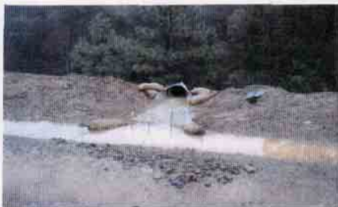
Figure 13: Inadequate BMPs at a location where storm water flows from the site into a down drain which directly flows under the roadway and into the creek
