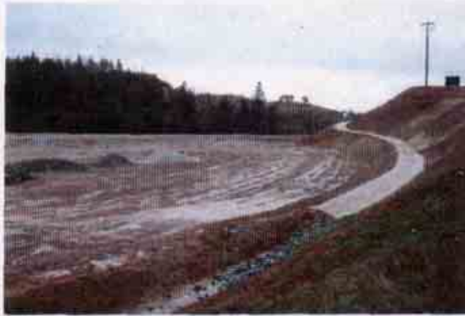
Figure 1: Lack of an effective combination of erosion and sediment control BMPs
