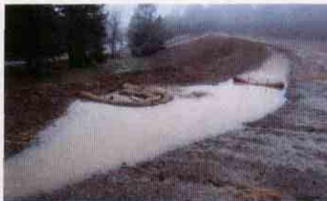
Figure 14: Inadequate BMPs at another one of the discharge areas
