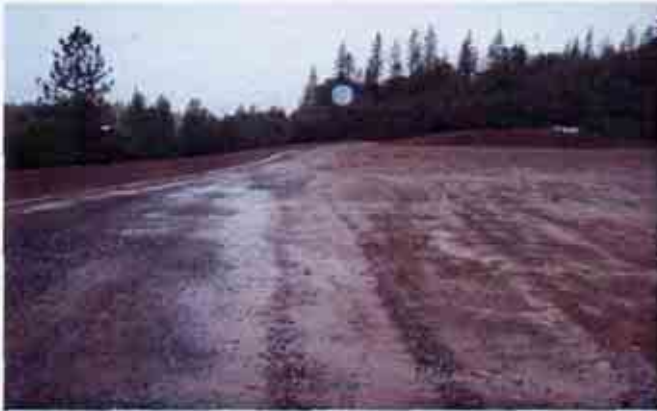
Figure 9: Another view of a portion of the flat pad without effective BMPs.
