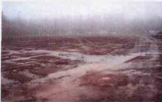
Figure 11: Lack of an effective combination of erosion and sediment control BMPs on another portion of the project
