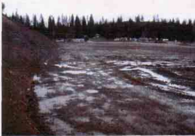
Figure 13: Lack of an effective combination of erosion and sediment control BMPs
