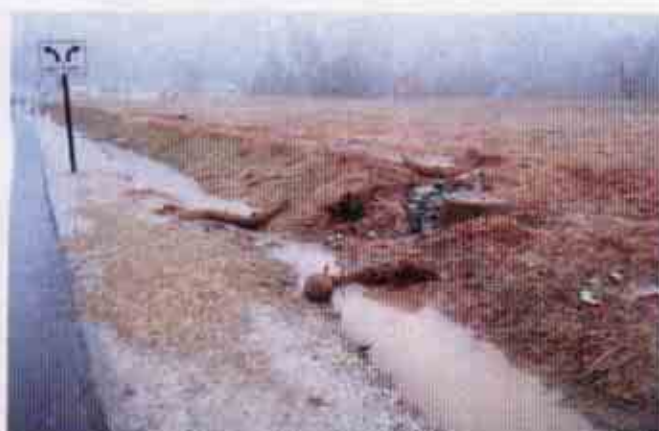
Figure 18: Another view of the poorly protected drain inlet
