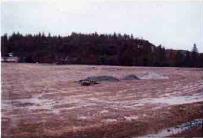
Figure 1: Overview of site, showing inadequate storm water BMPs. Storm water sheet flows to conveyance channels like that shown in Figure 2.
