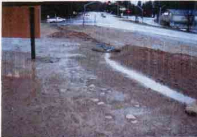
Figure 25: Lack of an effective combination of erosion and sediment control BMPs Note: the only BMP installed is a fiber roll
