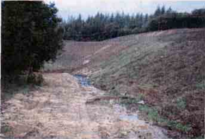
Figure 3: Storm water from the site flowing in a channel adjacent to highway 88 right-of-way
