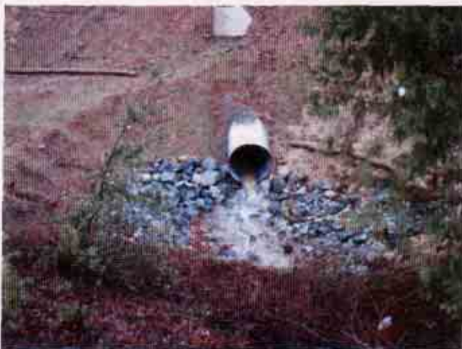
Figure 5: Another view of turbid storm water discharging into the eastern culvert which flows into Jackson Creek
