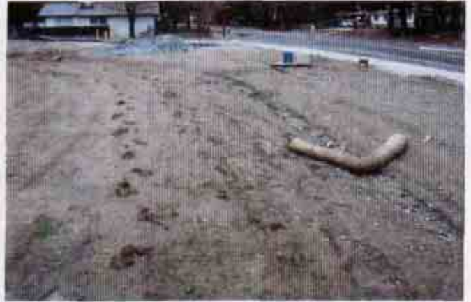
Figure 8: Another view of a portion of the project which requires additional BMPs
