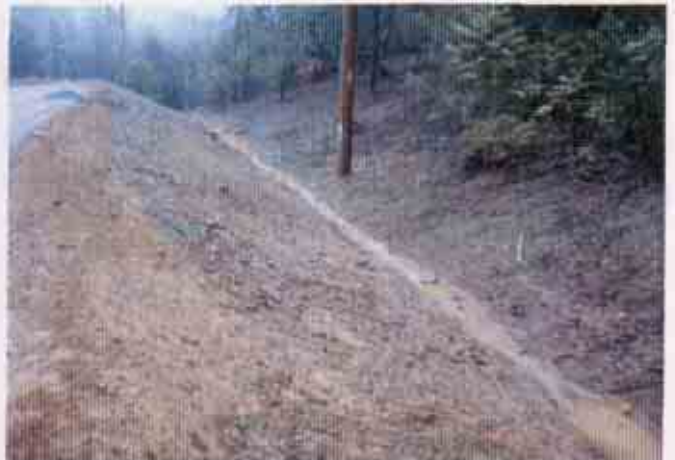
Figure 4: Lack of an effective combination of erosion and sediment control BMPs
