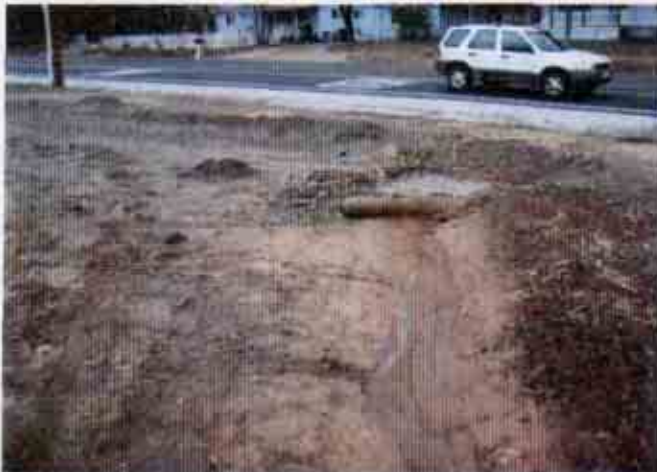
Figure 9: Poorly protected drain inlet
