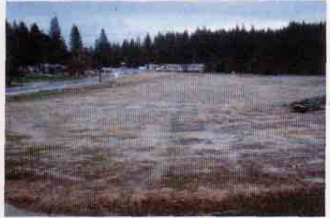
Figure 2: Lack of an effective combination of erosion and sediment control BMPs
