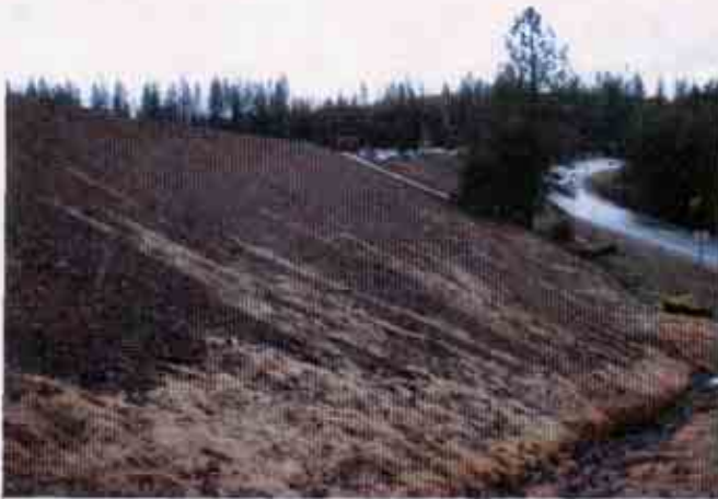
Figure 9: Lack of an effective combination of erosion and sediment control BMPs on the slope adjacent to Highway 88
