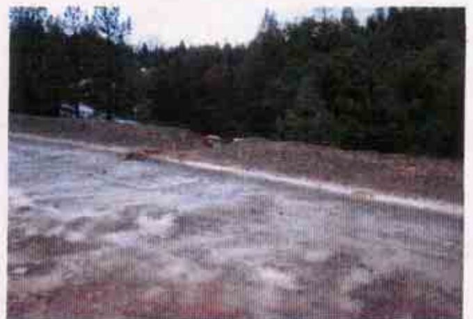
Figure 16: Lack of an effective combination of erosion and sediment control BMPs prior to one of the discharge locations
