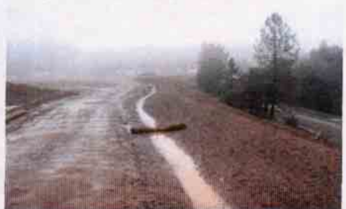
Figure 10: Lack of an effective combination of erosion and sediment control BMPs on a portion of the project
