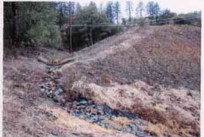
Figure 10: Lack of effective BMPs upslope of the western discharge location. Note: the large rill that is forming at the top of the slope
