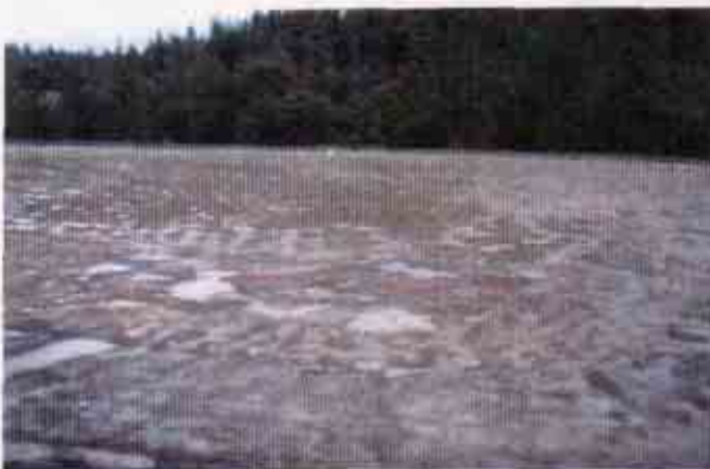
Figure 15: Lack of an effective combination of erosion and sediment control BMPs
