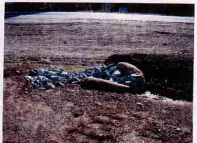
Figure 6: Another poorly installed and maintained BMP
