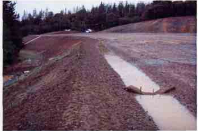
Figure 2: One of the channels directing storm water to a culvert that discharges under Highway 88, directly into Jackson Creek.
