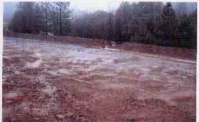
Figure 12: Lack of an effective combination of erosion and sediment control BMPs on still another portion of the project
