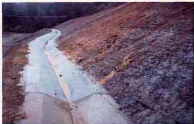
Figure 1: One of the many areas where soil is slumping on the steep slopes on the northern side of the project
