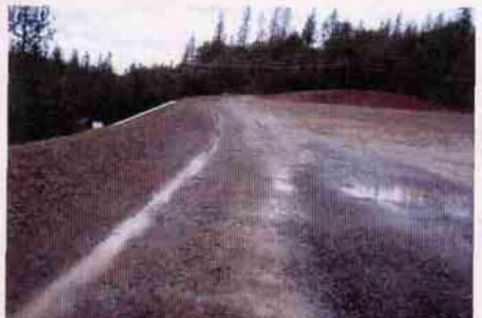
Figure 24: Lack of an effective combination of erosion and sediment control BMPs
