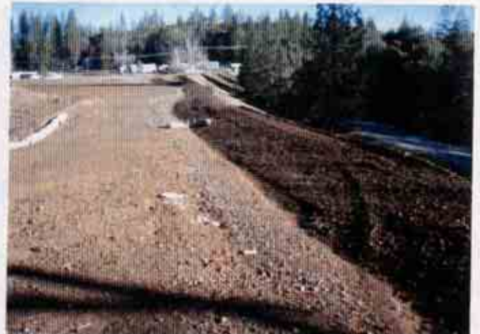
Figure 4: Lack of an effective combination of erosion and sediment control BMPs
