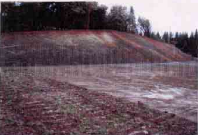
Figure 29: Lack of an effective combination of erosion and sediment control BMPs
