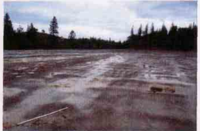
Figure 20: Lack of an effective combination of erosion and sediment control BMPs
