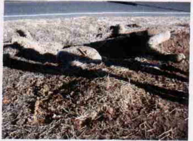
Figure 8: Poorly protected drain inlet
