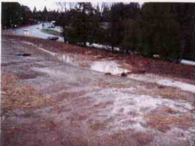
Figure 23: Another view of the same area Note: the general lack of erosion control BMPs
