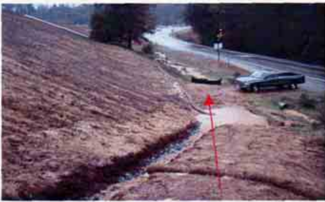
Figure 15: Turbid storm water from the project flowing down to the discharge location.
