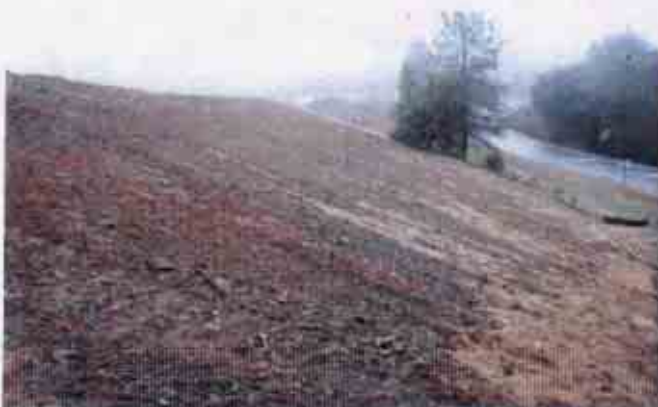
Figure 9: Poorly protected slopes
