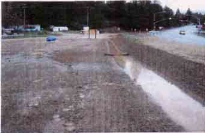
Figure 31: Lack of an effective combination of erosion and sediment control BMPs
