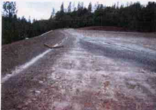
Figure 21: Lack of an effective combination of erosion and sediment control BMPs
