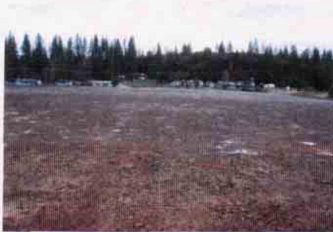
Figure 15: Lack of an effective combination of erosion and sediment control BMPs
