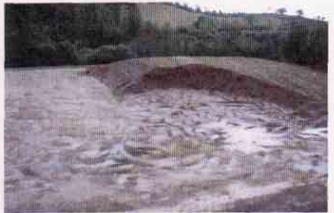
Figure 16: Lack of an effective combination of erosion and sediment control BMPs Note: the poorly stabilized stockpile
