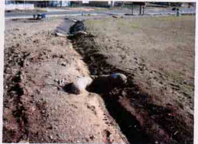
Figure 10: Poorly installed and maintained BMPs
