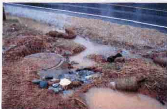
Figure 17: Poorly protected drain inlet along Ridge Road
