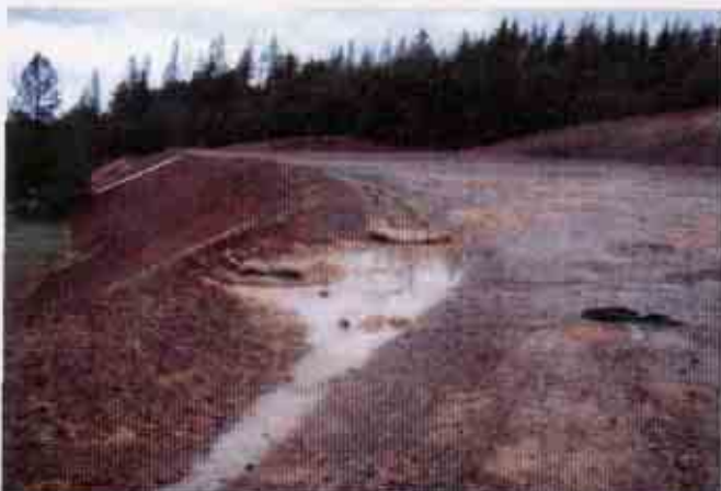
Figure 23: Turbid storm water ponded onsite just prior to discharge into the eastern culvert
