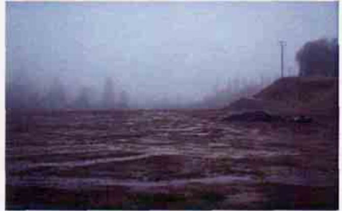
Figure 22: Lack of an effective combination of erosion and sediment control BMPs on another portion of the project
