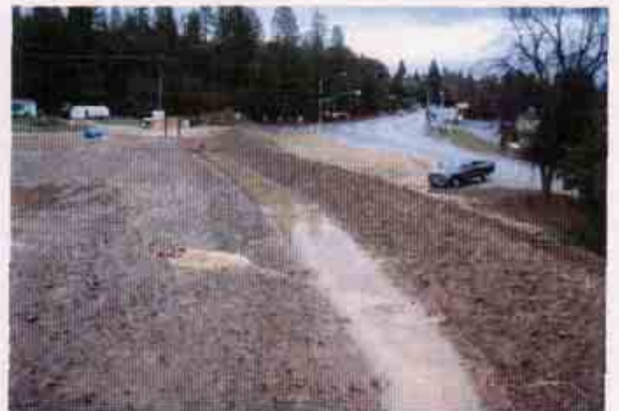
Figure 22: Turbid storm water flowing on the site Note: the lack of effective storm water management BMPs
