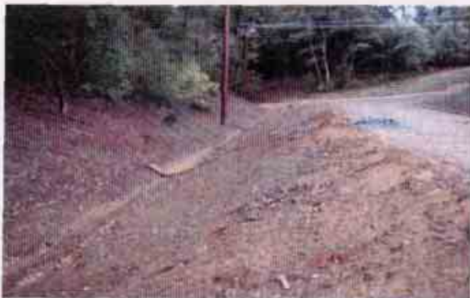
Figure 11: Lack of effective BMPs on top of the slope above the western discharge location
