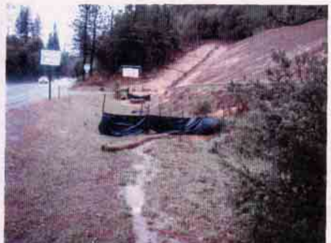
Figure 6: Looking at the western discharge location in the distance
