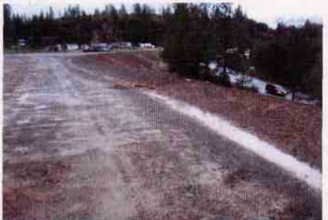
Figure 30: Lack of an effective combination of erosion and sediment control BMPs
