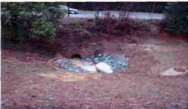
Figure 15: Storm water discharge from the site entering the culvert which flows under the highway and directly into the creek
