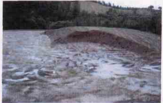
Figure 14: Poorly stabilized stockpile
