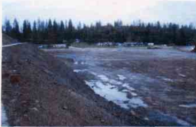
Figure 13: Lack of an effective combination of erosion and sediment control BMPs
