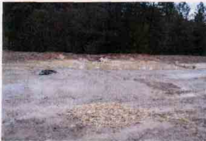
Figure 21: Lack of an effective combination of erosion and sediment control BMPs Note: the turbid storm water ponded adjacent to one of the discharge locations
