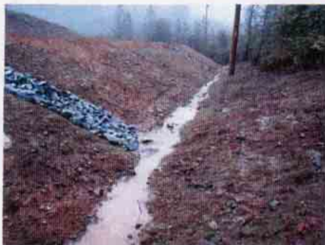
Figure 5: Lack of effective BMPs on the slopes and lack of BMPs in a defined drainage channel
