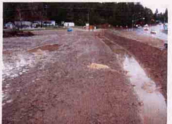
Figure 24: Lack of an effective combination of erosion and sediment control BMPs
