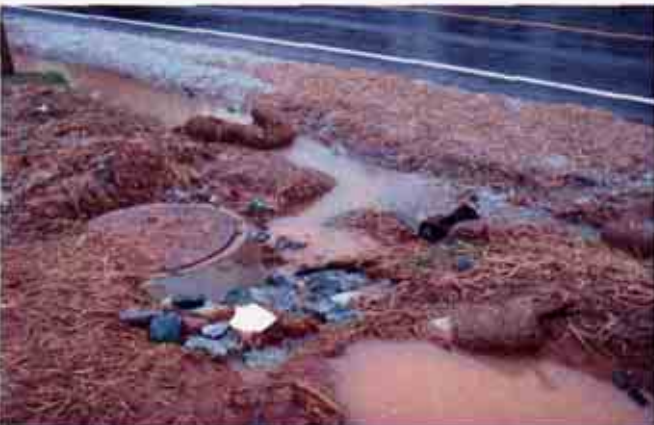
Figure 17: Poorly protected drain inlet along Ridge Road
