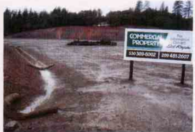
Figure 26: Another view of the same area Note: the lack of erosion control BMPs
