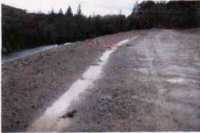
Figure 25: Lack of an effective combination of erosion and sediment control BMPs Note: the only BMPs observed were a few small fiber rolls
