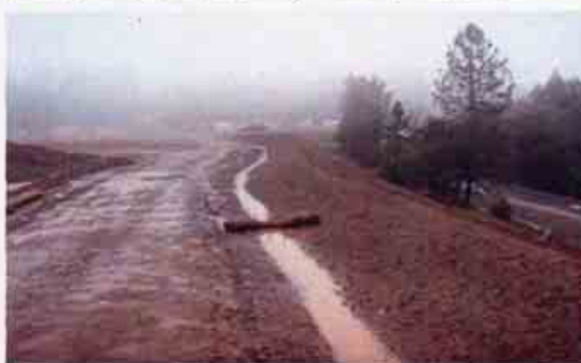
Figure 10: Lack of an effective combination of erosion and sediment control BMPs on a portion of the project
