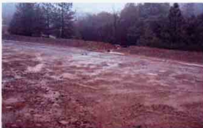
Figure 12: Lack of an effective combination of erosion and sediment control BMPs on still another portion of the project
