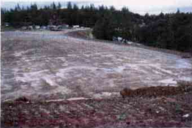
Figure 27: Lack of an effective combination of erosion and sediment control BMPs
