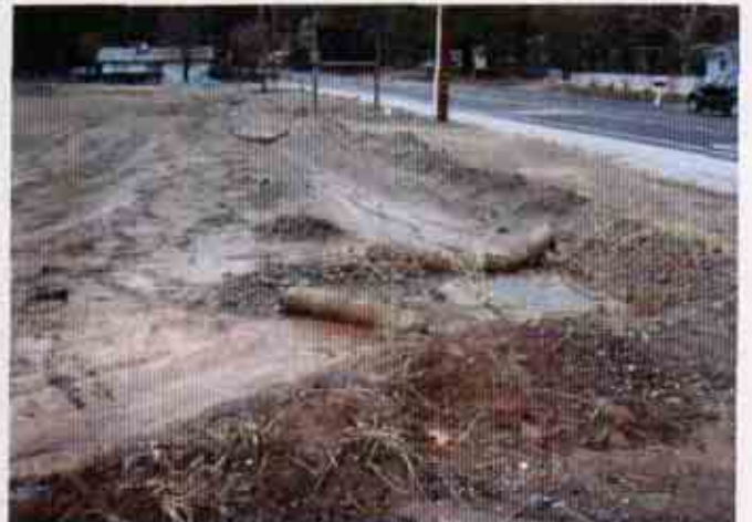
Figure 10: Another view of the protected drain inlet
