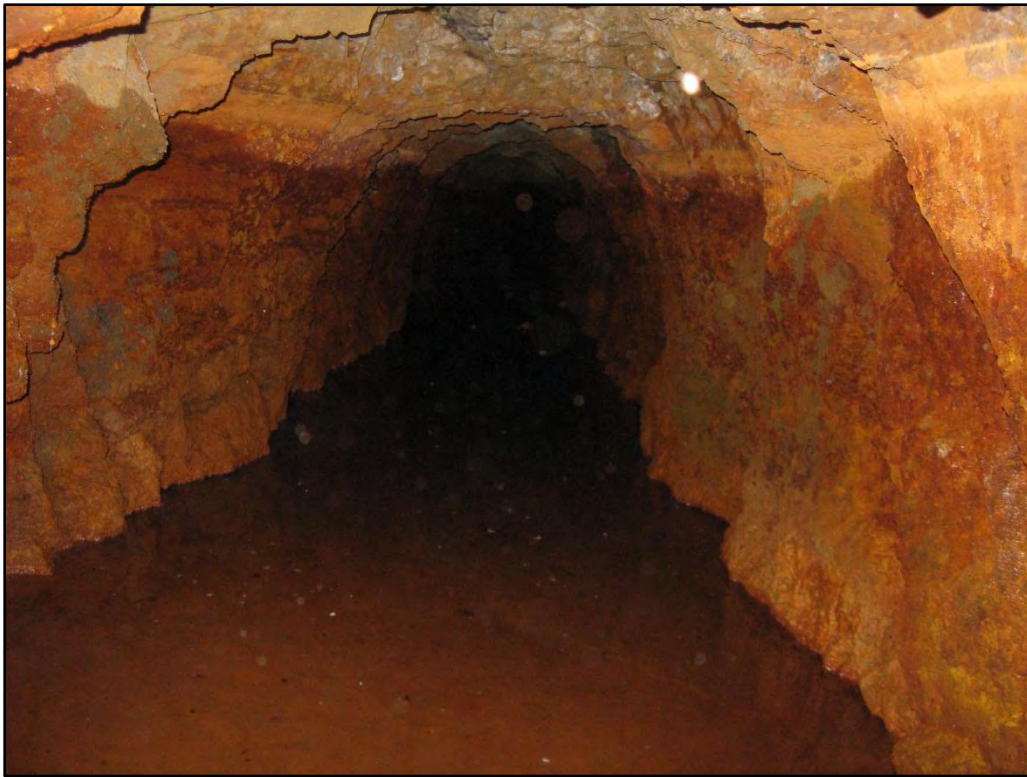
Figure 11. Entrance to Corona Mine Boiler House Portal showing the bulkhead and drain pipe (top) and the interior (bottom) showing standing water.
