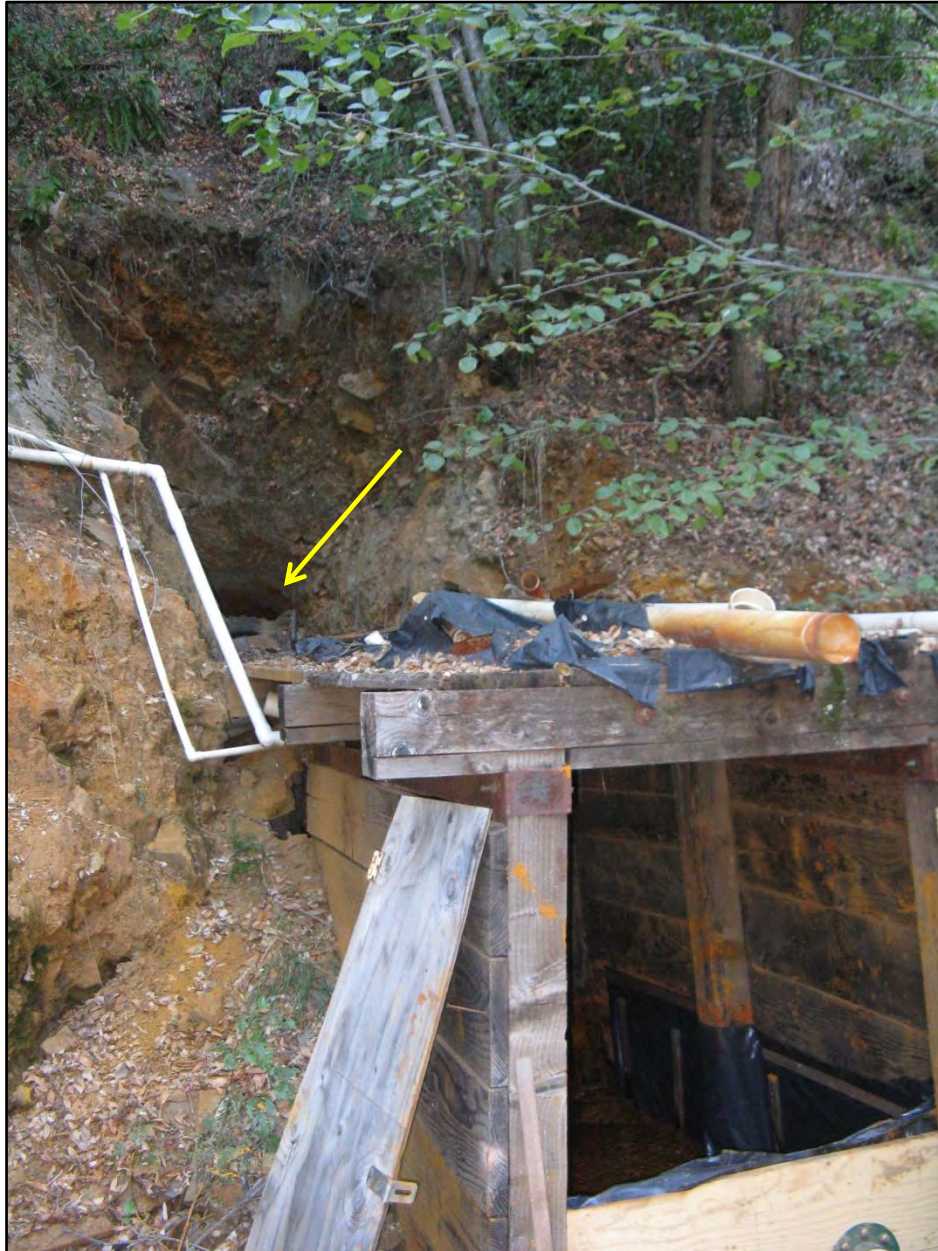
Figure 9. Entrance to Corona Mine drain portal. Arrow shows restricted potential bat flight passage area largely filled with debris.
