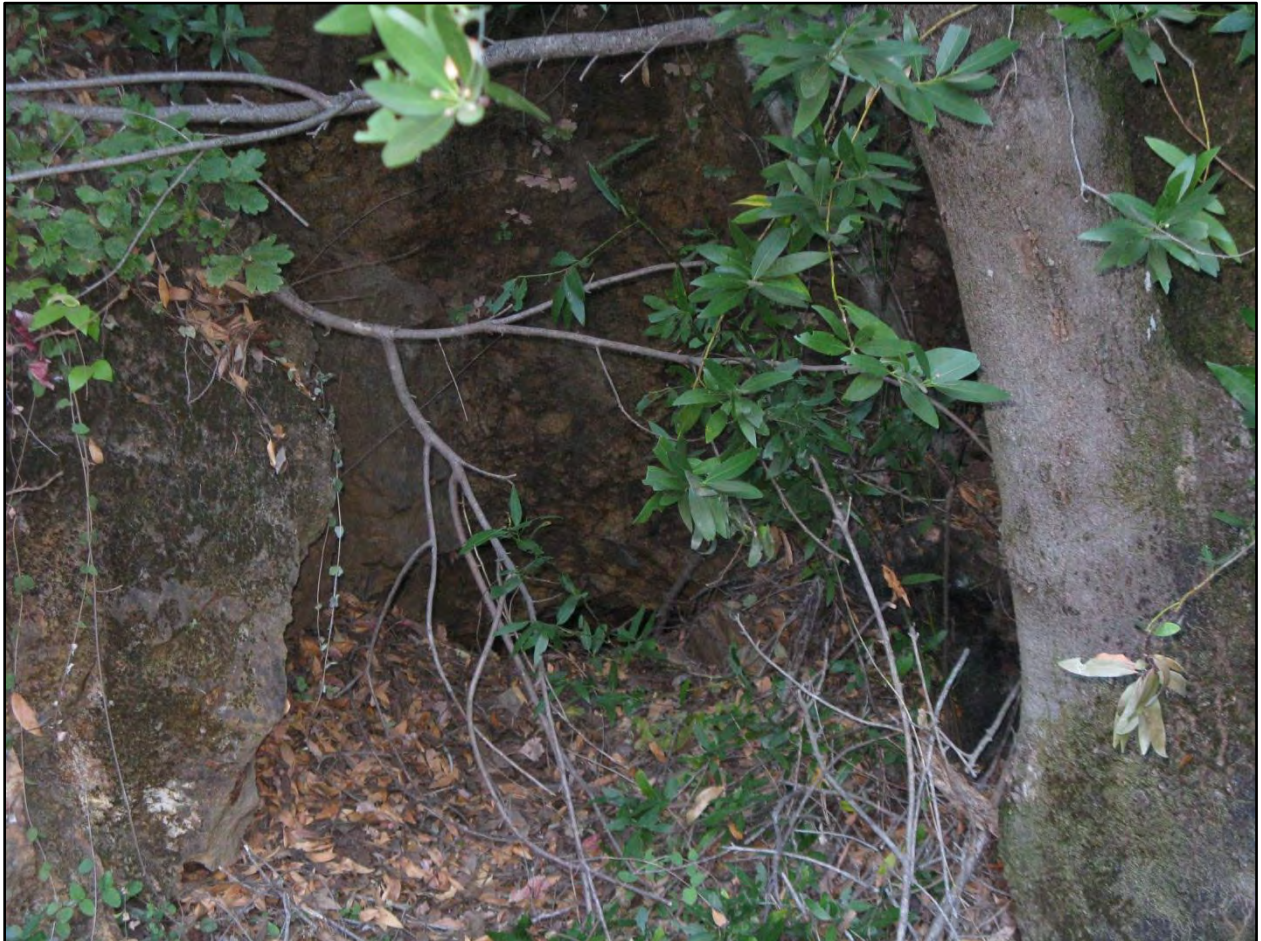
Figure 14. Entrance to Twin Peaks Mine Adit 2 showing dense vegetation blocking the opening.
