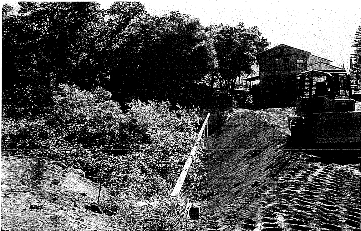
Figure 2. View of illegal impoundment on south side of drainage.
