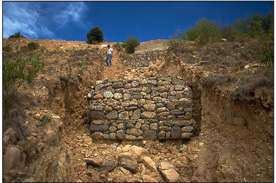
Photo 14.3 An expensive but failed gabion gully control structure that was not properly keyed into the banks of the gully. Further, the flow was not kept over the protected middle of the structure.
