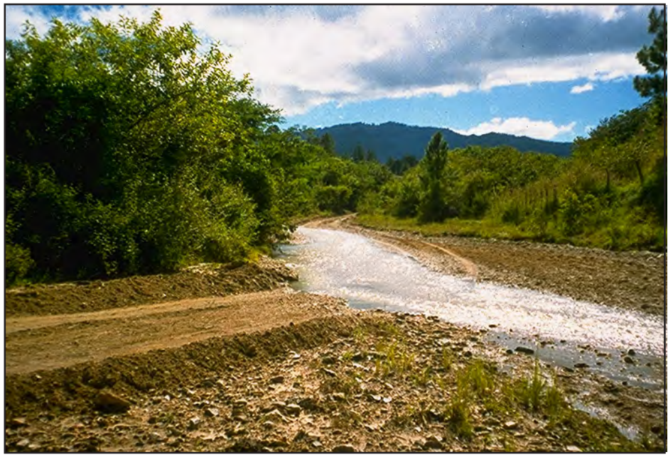
Photo 7.8 Avoid natural drainage crossings that are broad and that are not perpendicular to the drainage. Stay out of the stream! This broad channel is a good site for a vented ford.
