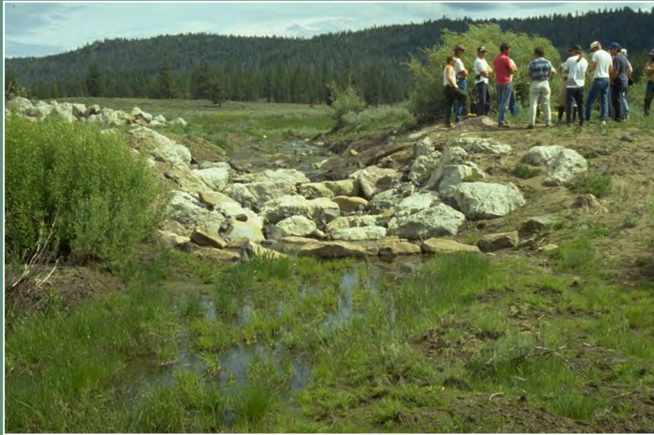
Depicted above is a loose rock gully control structure being used to stop headcutting up into the meadow. Note that the rock structure is well keyed into the banks and channel bottom.
