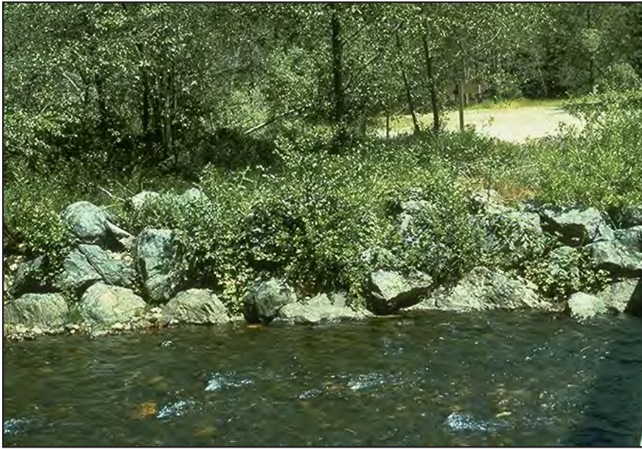
Photo 6.2 Riprap used for stream bank slope protection to prevent scour at the entrance of a structure. Note the use of willows for additional “biotechnical” root strength.
