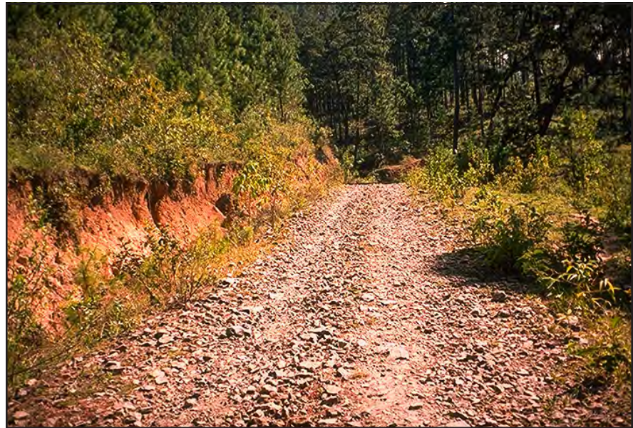
Photo 12.2 Stabilize the roadway surface with crushed rock (or other surfacing) on steep grades, in areas of soft soil, or in erosive soils.
