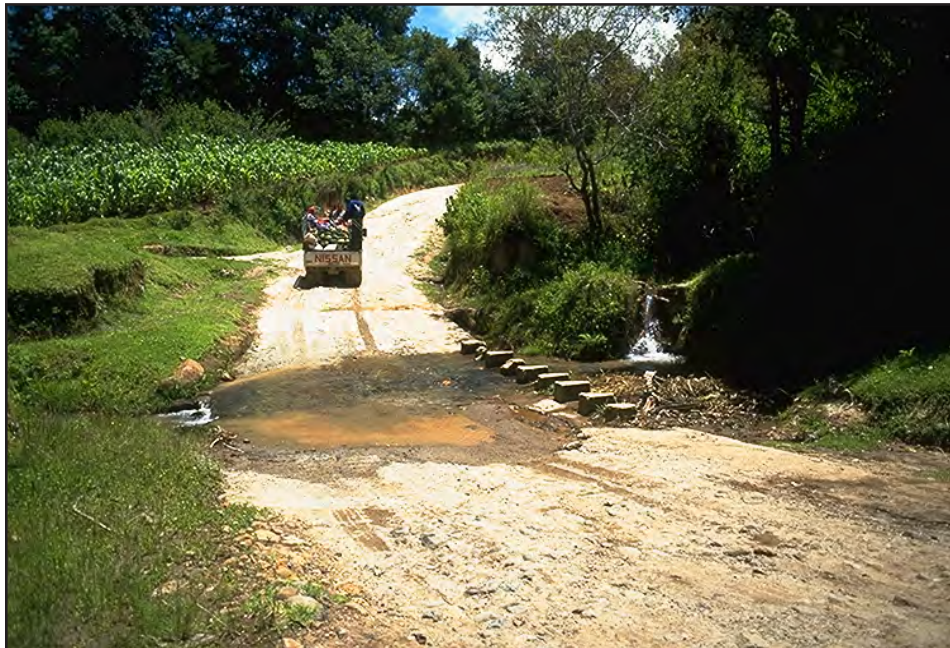
Photo 9.1 Use armored low-water crossings, fords, or drifts as often as possible to cross low flows in broad, shallow natural drainages, thus avoiding the use of pipes. Note that part of this reinforced driving surface needs repair.
