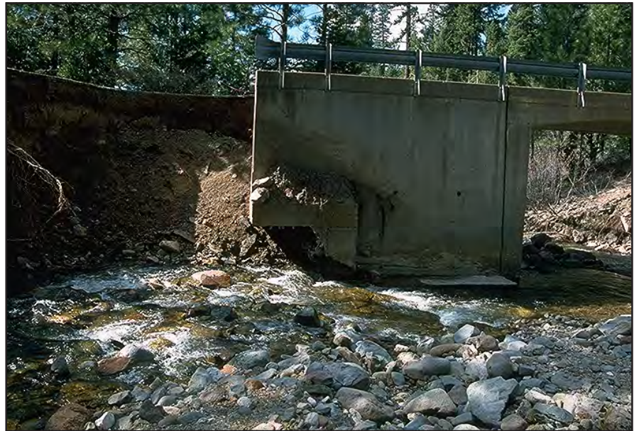
Photo 10.3 Scour is one of the most common causes of bridge failure. Use an opening wide enough to minimize constriction of the natural channel. Locate the bridge foundation on bedrock when possible, or below the depth of scour, and use stream bank protection measures such as riprap.
