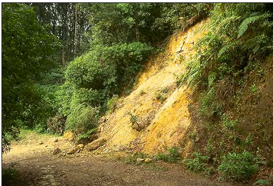
Photo 11.1 Over-steep slopes, wet areas, or existing slide areas can cause instability problems for a road and increase repair and maintenance costs, as well as sediment production.
