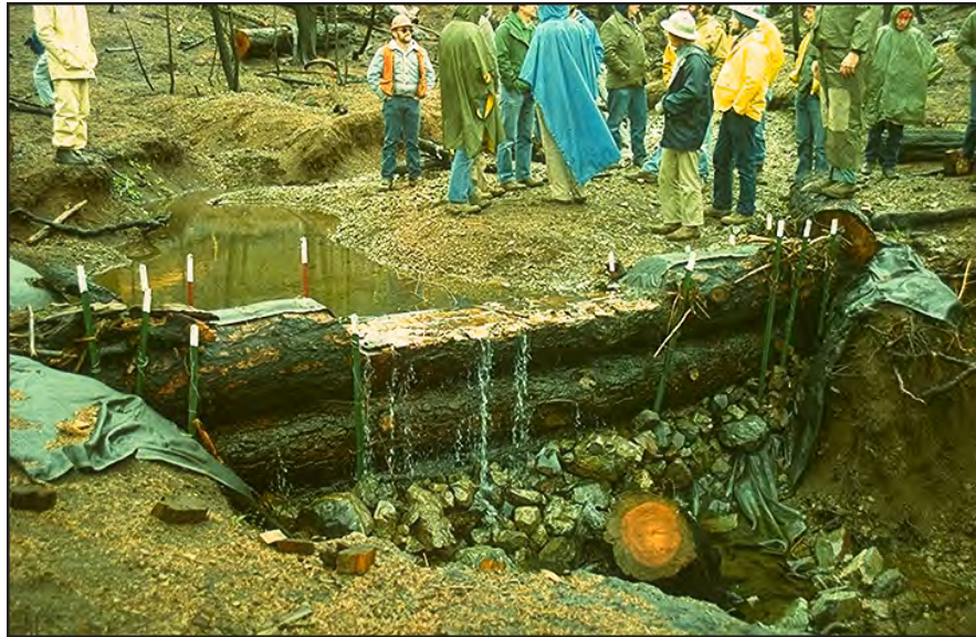
Photo 14.2 Logs being used to build gully stabilization structures in a fire damaged area. Physical or vegetative dams (dikes or debris retention structures) may be used to control sediment and stabilize gullies. Prevent water concentration before gullies form.
