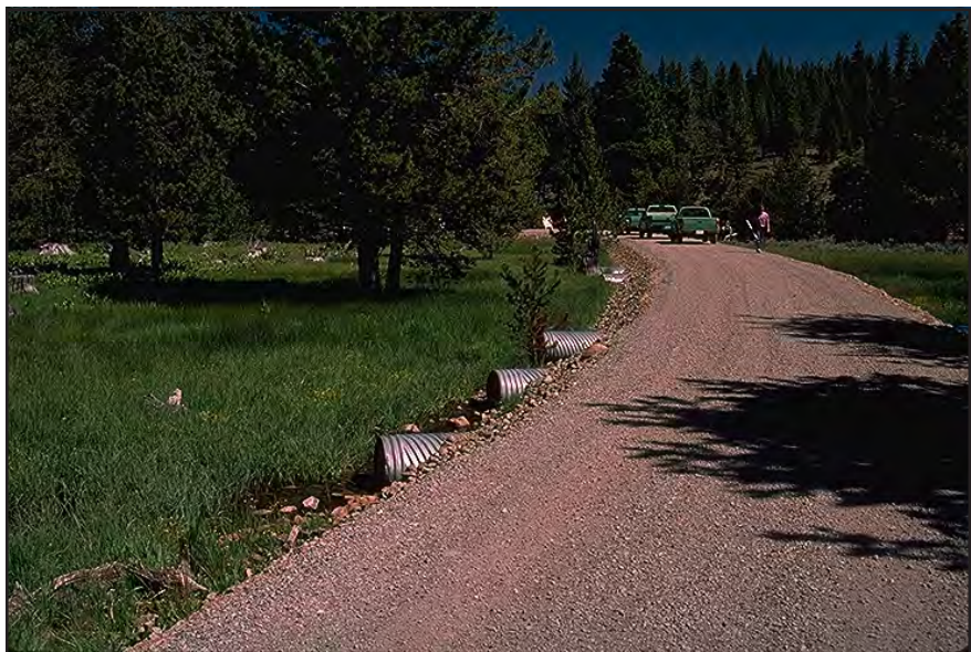
Photo 7.9 Avoid crossing wet meadow areas. When necessary to cross, use multiple drainage pipes to keep water flow dispersed across the meadow.
