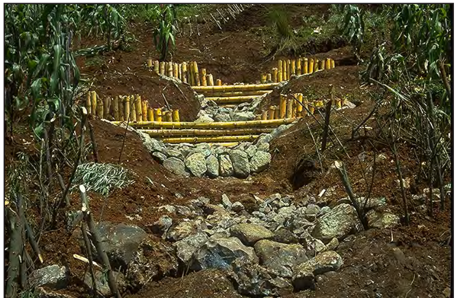
Photo 14.4 Construct debris retention and gully control structures with a notched wier to keep flow over the middle of the structure, add scour protection at the outlet of each structure, and key the structures into the firm soil banks.
