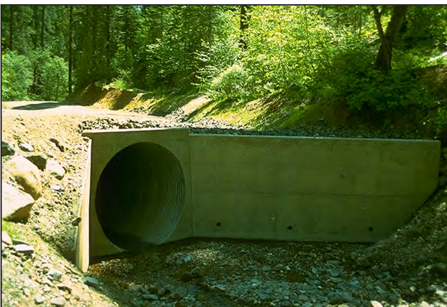
Photo 8.8 Install culverts with adequate capacity. Use headwalls to improve culvert capacity, protect the roadway fill, resist overtopping damage, and prevent bank scour, particularly at a bend in the channel.
