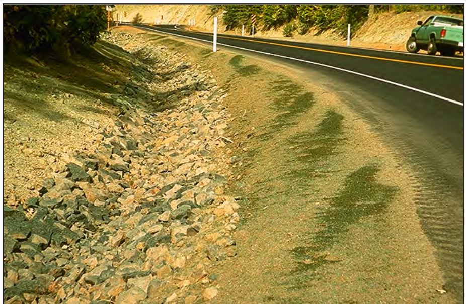
Photo 3.5 Maintain roads and drainage features to withstand major storm events with minimum erosion, such as with armored ditches that are kept clean.
