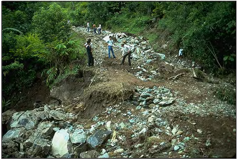
Photo 3.4 A road that has been heavily damaged during a storm because of an undersized, plugged culvert pipe and no overflow protection.
