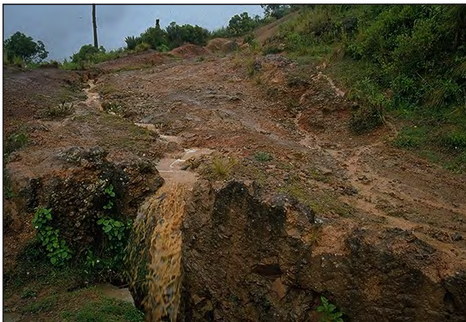
Photo 13.1 Do not leave disturbed or barren areas exposed to raindrops and runoff. Use erosion control measures to protect the area and protect water quality.
