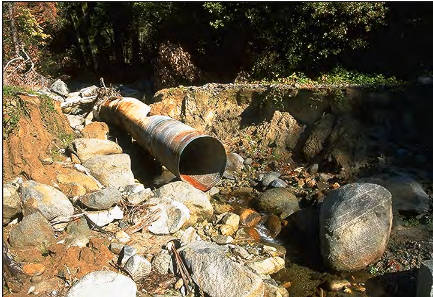
Photo 8.2 A culvert failure caused by insufficient flow capacity or inadequate pipe size to pass the debris (boulders) moving through the drainage.
