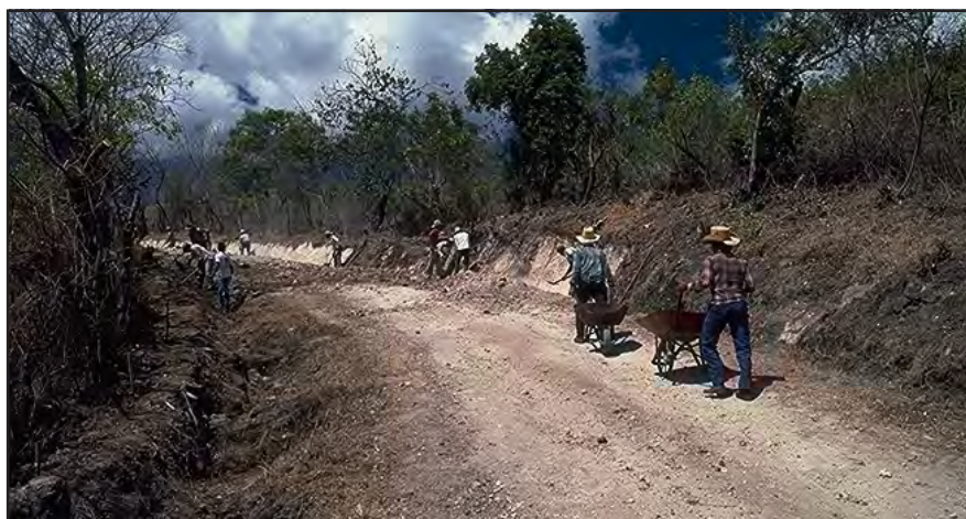
Photo 4.7 Use the road construction techniques that are most appropriate and cost-effective for the job and geographic area. Hand labor versus equipment depends on labor costs, equipment availability, and production rates.
