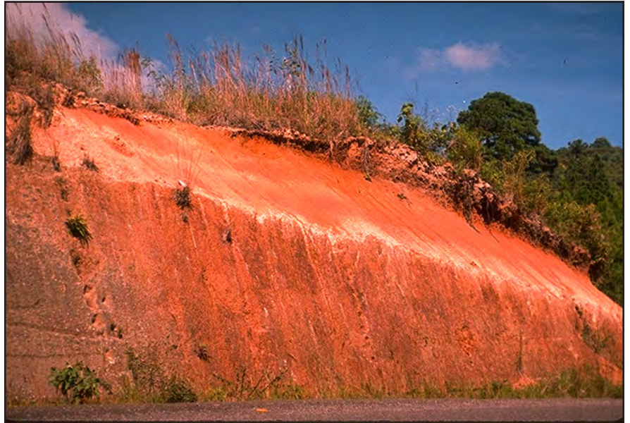
Photo 11.2 Construct cut slopes at a 3/4:1 or flatter slope in most soils for long-term stability. In well-cemented soils and rock, a 1/4:1 cut clope will usually be stable.
