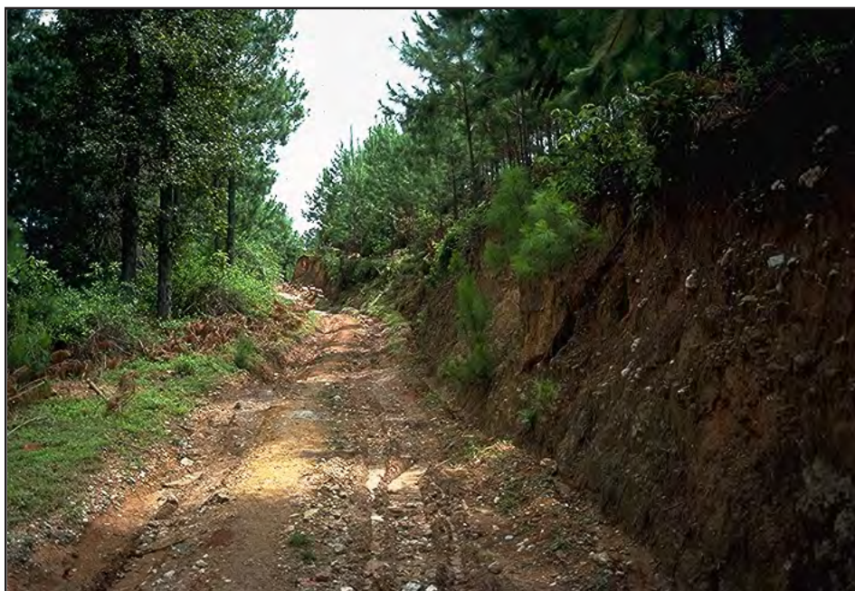
Photo 12.1 A rutting road caused either by soft subgrade soil or inadequate road drainage (or both).
