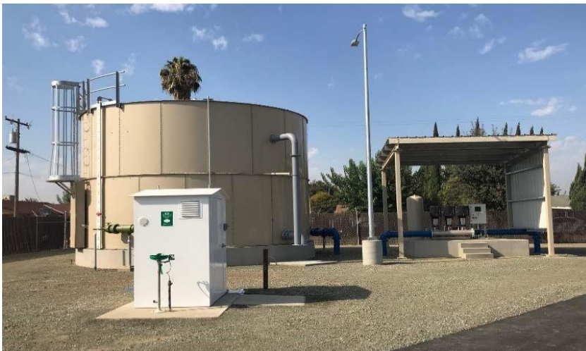
Photo 1: New booster station and storage tank.
