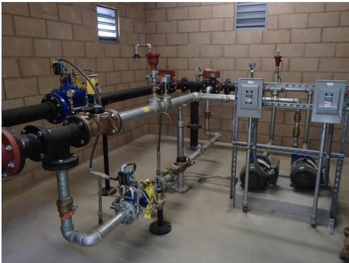
Photo 1: Drought emergency intertie and pump station
