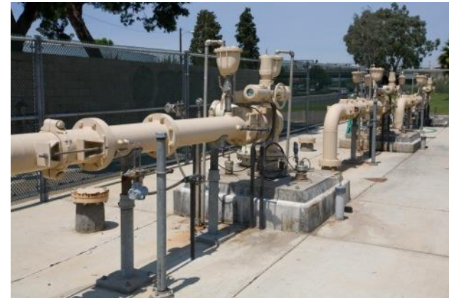
Typical injection well - OCWD
