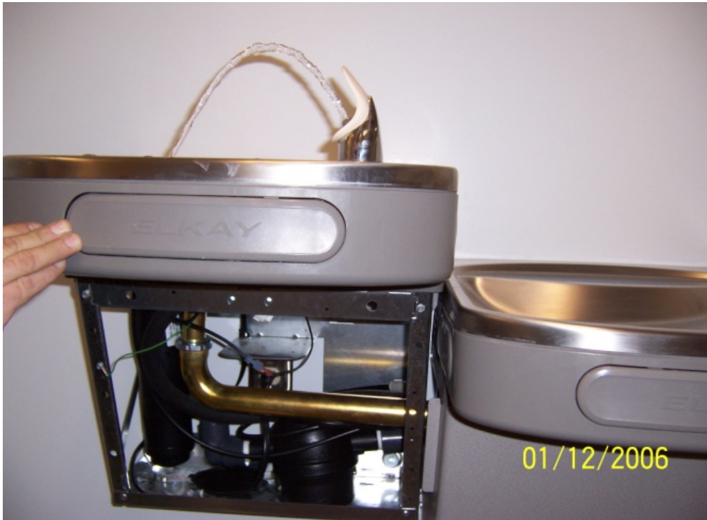
Figure 4-4. POU AM Units Installed Under a Sink (top) and Inside a Drinking Water Fountain (bottom)
