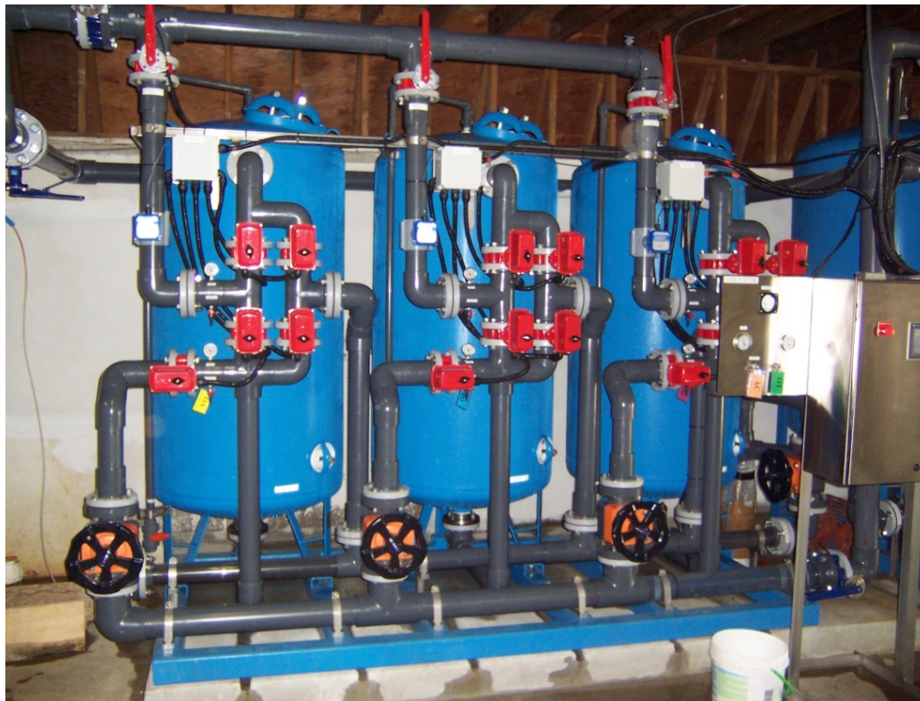
Figure 3-1D. 250-gpm AD26/E33 Filtration System by AdEdge
