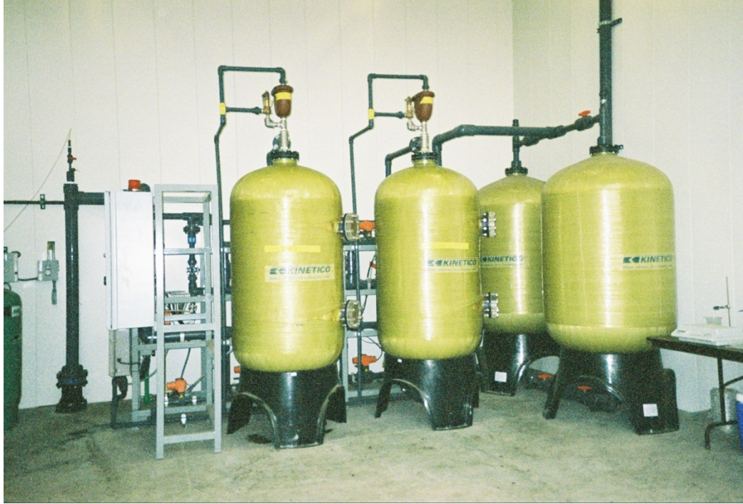
Figure 3-1C. 140-gpm Macrolite® Pressure Filtration System by Kinetico (Clockwise from Left: Control Panel, Macrolite® Filters, and Contact Tanks)
