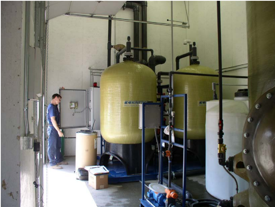
Figure 4-1. Photograph of IX-248-As/N System at Fruitland, ID
