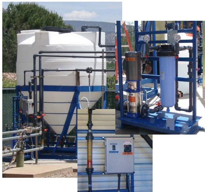
Figure 2-6. Backwash Recycling System at VV (Clockwise from Left: 1,800-gal Holding Tank; Recycle Pump and Bag Filter; and Backwash Flowrate Indicator and Pump Box)
