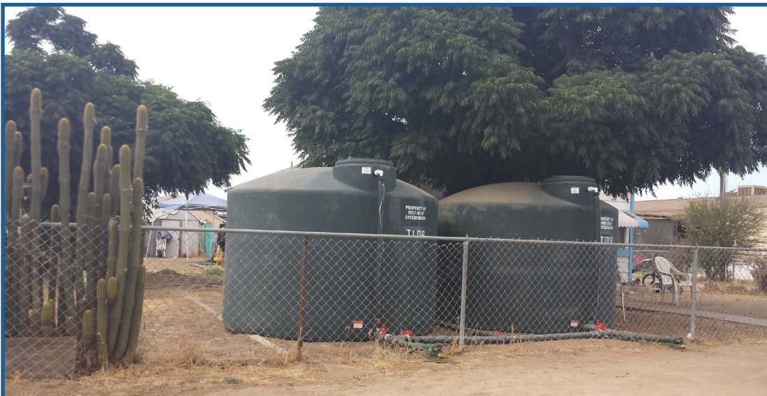
LEFA Project - Okieville - 2 Tanks as 2 Owners Occupied Homes on Property Where Wells Were Dry
