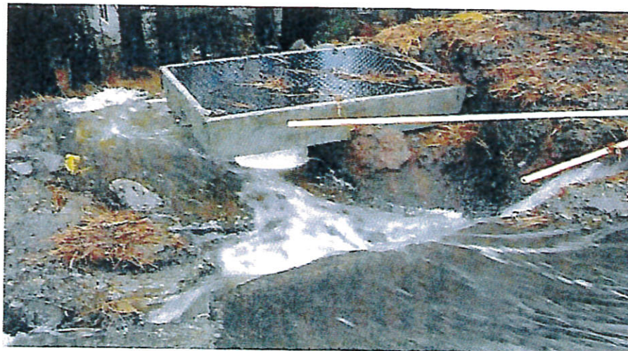
Photo 13. Eroded water utilities on West Reed Avenue.
