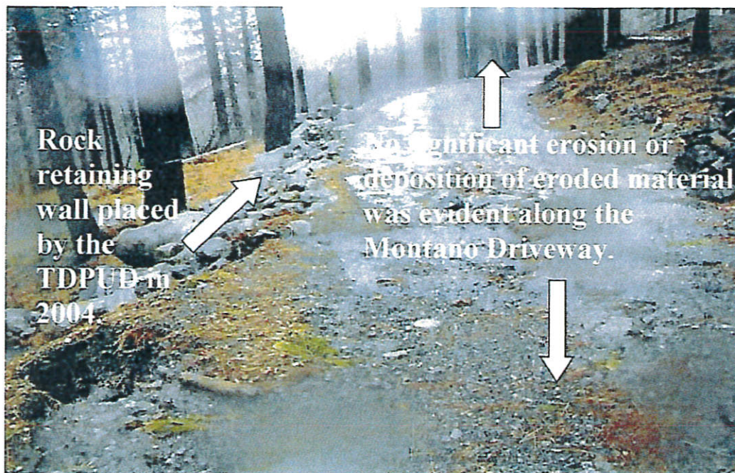
Photo 26. The west end of the TDPUD’s Cedar Point pipeline alignment through the Robert Montano property that is planned for asphalt paving. Photo taken December 31, 2005.
