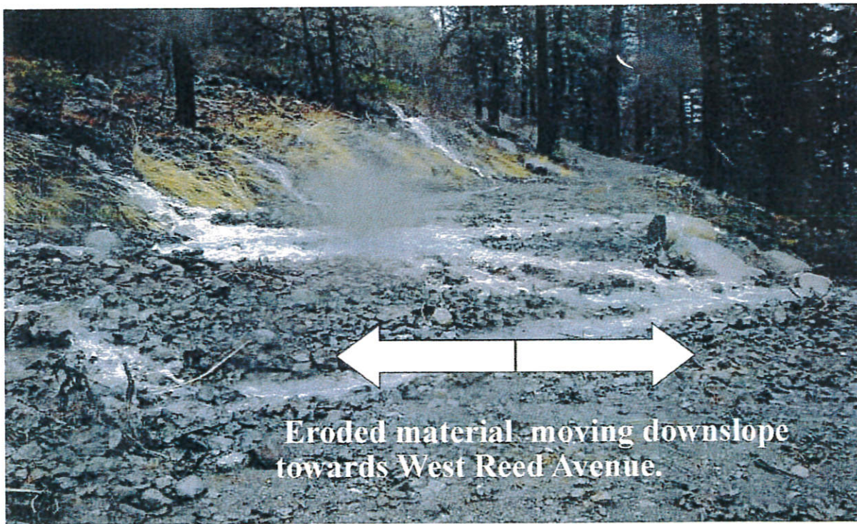
Photos 3 and 4. High velocity runoff outside Caltrans culvert and eroded material being transported downslope. Photo taken December 31, 2005.
