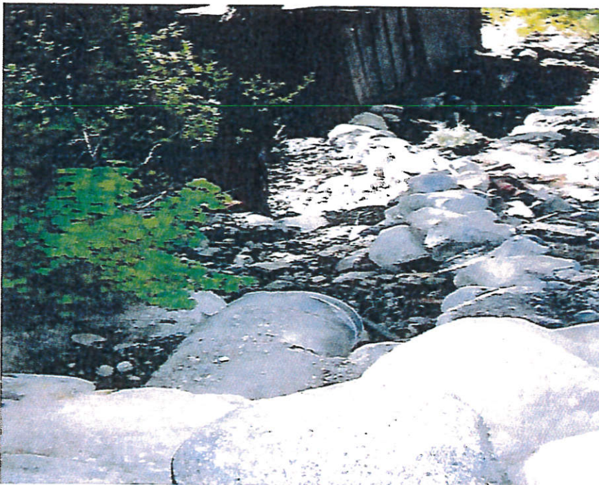
Photo 10. A culvert outfall on the south side of West Reed Avenue does not convey runoff effectively as debris clogs the inlet on the north side of the road. Photo taken May 29, 2006.
