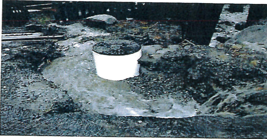
Photo 11. Eroded water utilities on West Reed Avenue.
