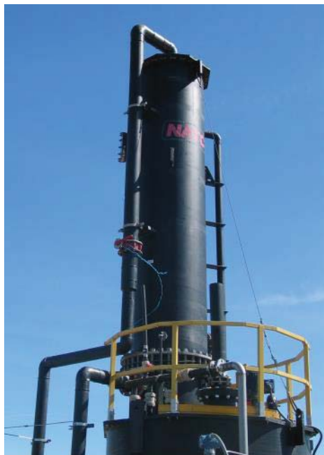
Dairy gas cleanup system (gas scrubber)
