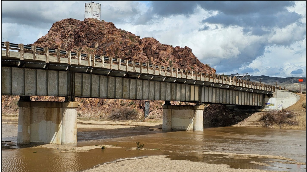
Figure 3.1 - Barstow First Street from east side of the First Street Bridge on 03/15/2023. USGS Barstow stream gage measured discharge is 133 cubic feet per second
