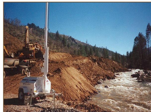
This photo of the American River shows a mass failure that temporarily blocked the river. This slide was believed to be the result of lack of vegetation from a previous fire, defoliation efforts, and water associated with a 100-year precipitation event (1997).
