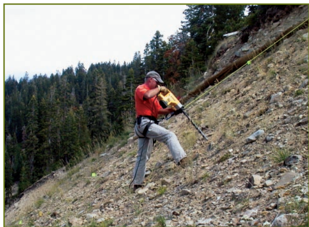
Drilling holes using hammer drill to increase infiltration on extremely dense cut slope in Squaw Valley.
