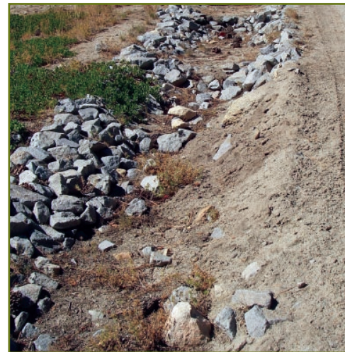
Deposited sediment in unmaintained rock-lined ditch.
