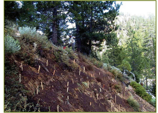
3- Wooden stakes were hammered into slope to increase infiltration and provide anchors to hold compost in place.
