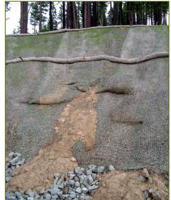
Clear evidence of significant erosion occurring underneath erosion control blankets.
