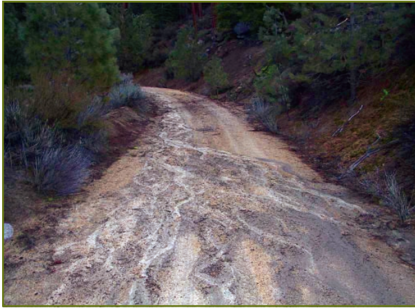
Erosion on dirt road.
