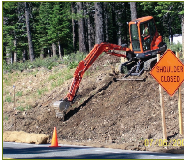
Responding to slope failures using subsurface “scallop” and temporary irrigation – Summer 2006.
