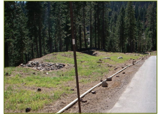
Infiltration areas off Highlands View Drive at Northstar-at-Tahoe. Full soil-vegetation treatment was implemented to maximize infiltration over the entire roadside. In addition, berms were constructed every 50 feet to direct high flows to stable, rock-armored outfall areas.
