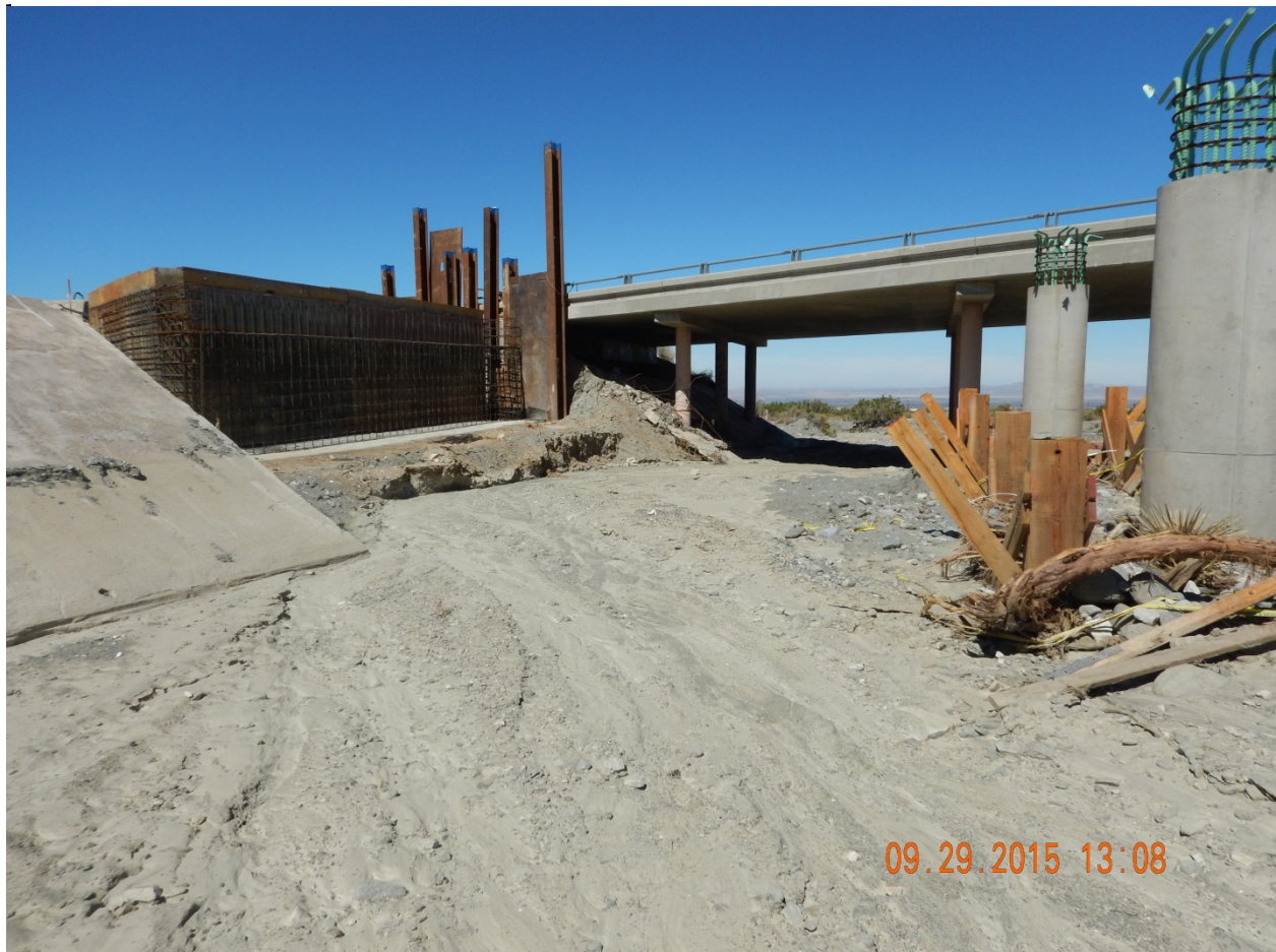
Picture 26: View North within Sheep Creek. Note lack of BMPs on creek banks and debris accumulation upstream of footings from last storm event.
