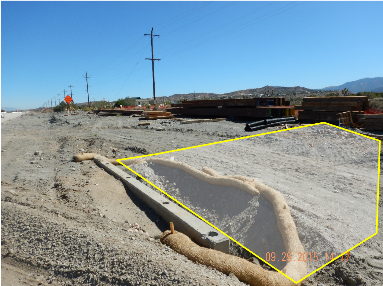
Picture 4: View South East of unpermitted temporary impact at Drainage ID 54. Note fill from access road in the stream channel (rough outline of area in yellow).
