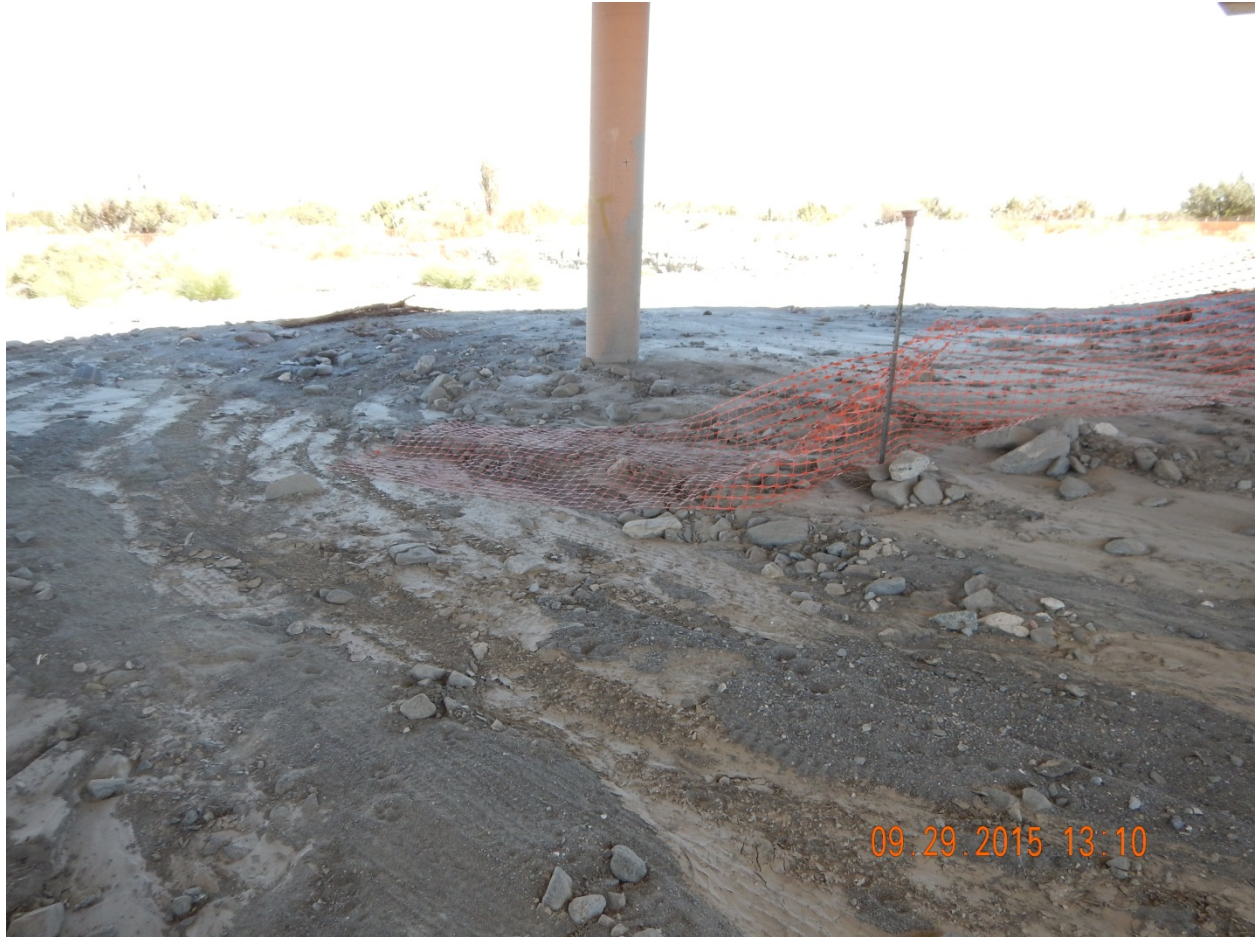
Picture 22: Beneath the Sheep Creek Bridge. Note damaged construction fencing left in the creek.
