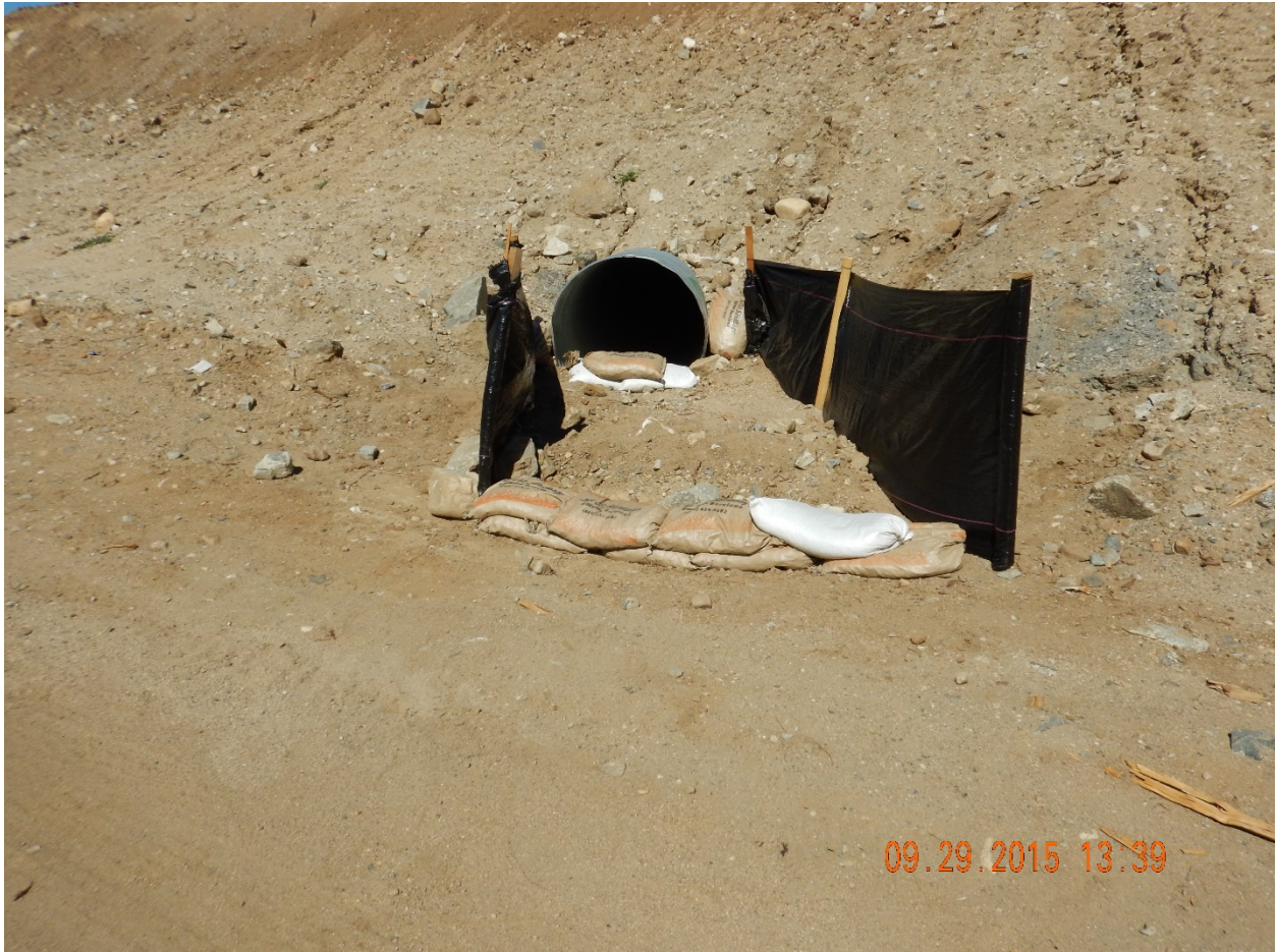
Picture 7: View North of Drainage ID 55. Note the inadequate BMPs and unconsolidated sediment and sandbags in the stream channel.
