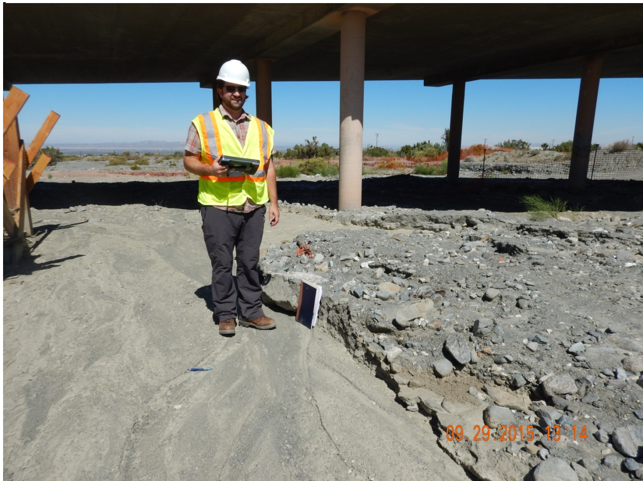
Picture 25: View North within Sheep Creek. Note approximately 10 inches of unconsolidated sediment washed out from this location during last storm event.
