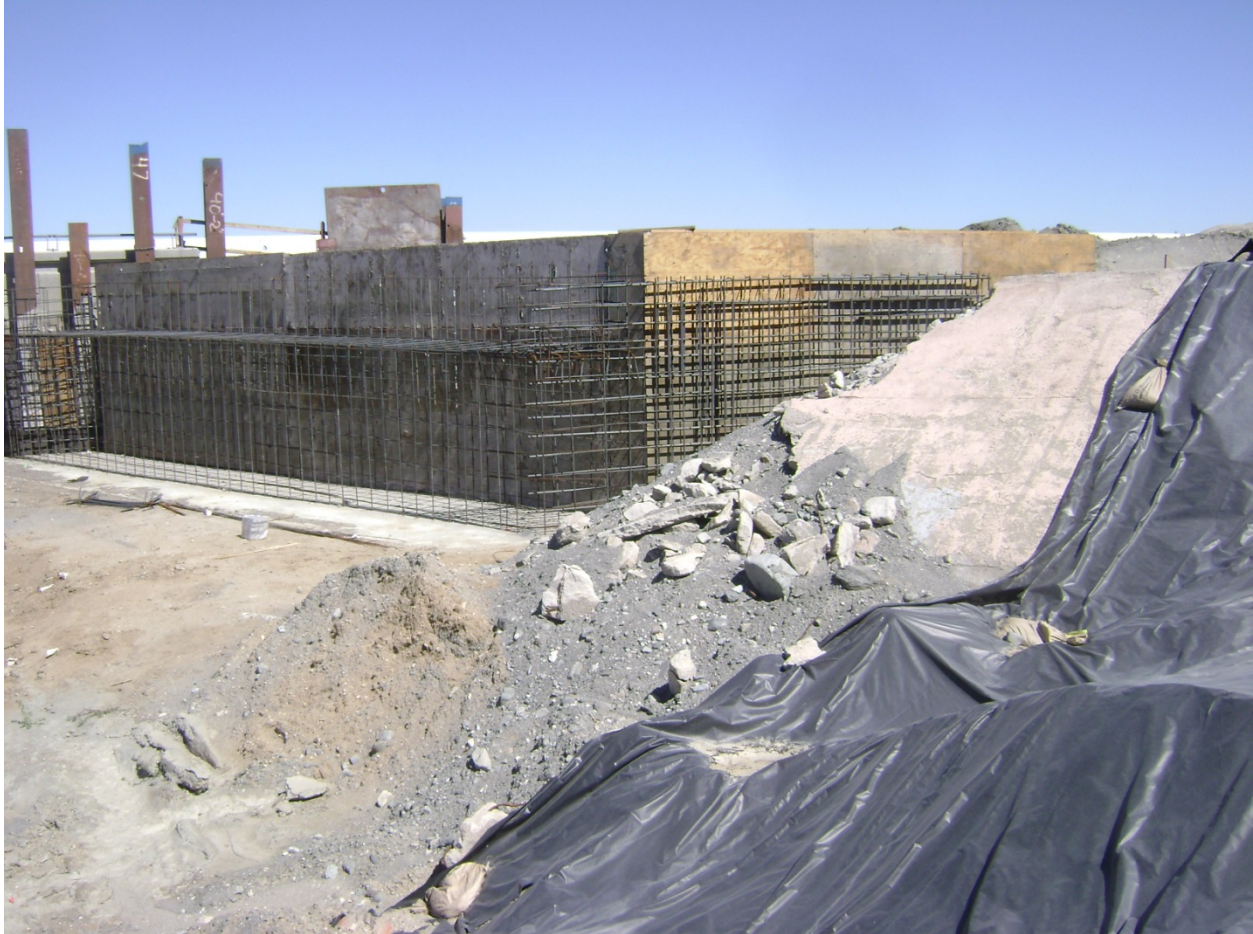
Picture 20: View North Within Sheep Creek. Note Inadequate BMPs.
