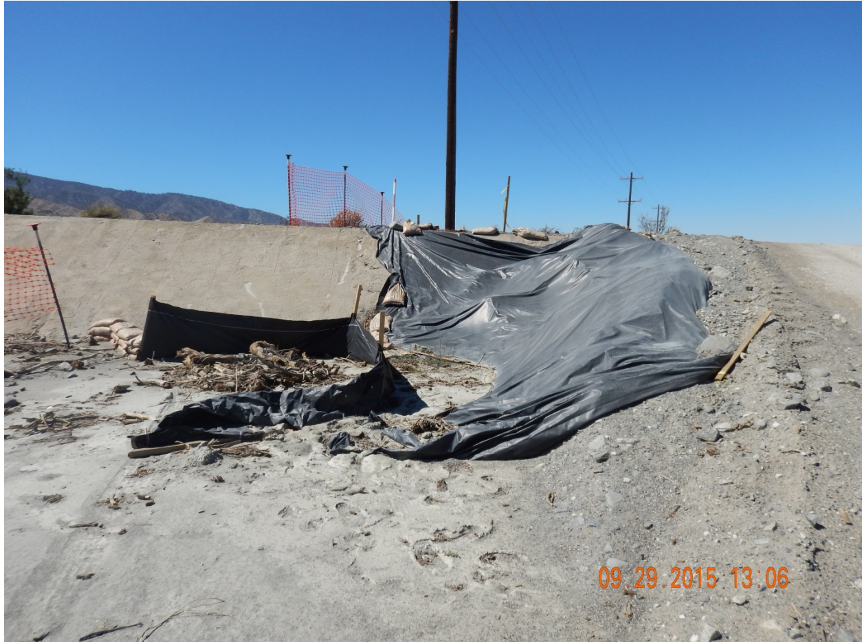
Picture 28: View West from within Sheep Creek. Note inadequate BMPs and failing improperly installed silt fencing.
