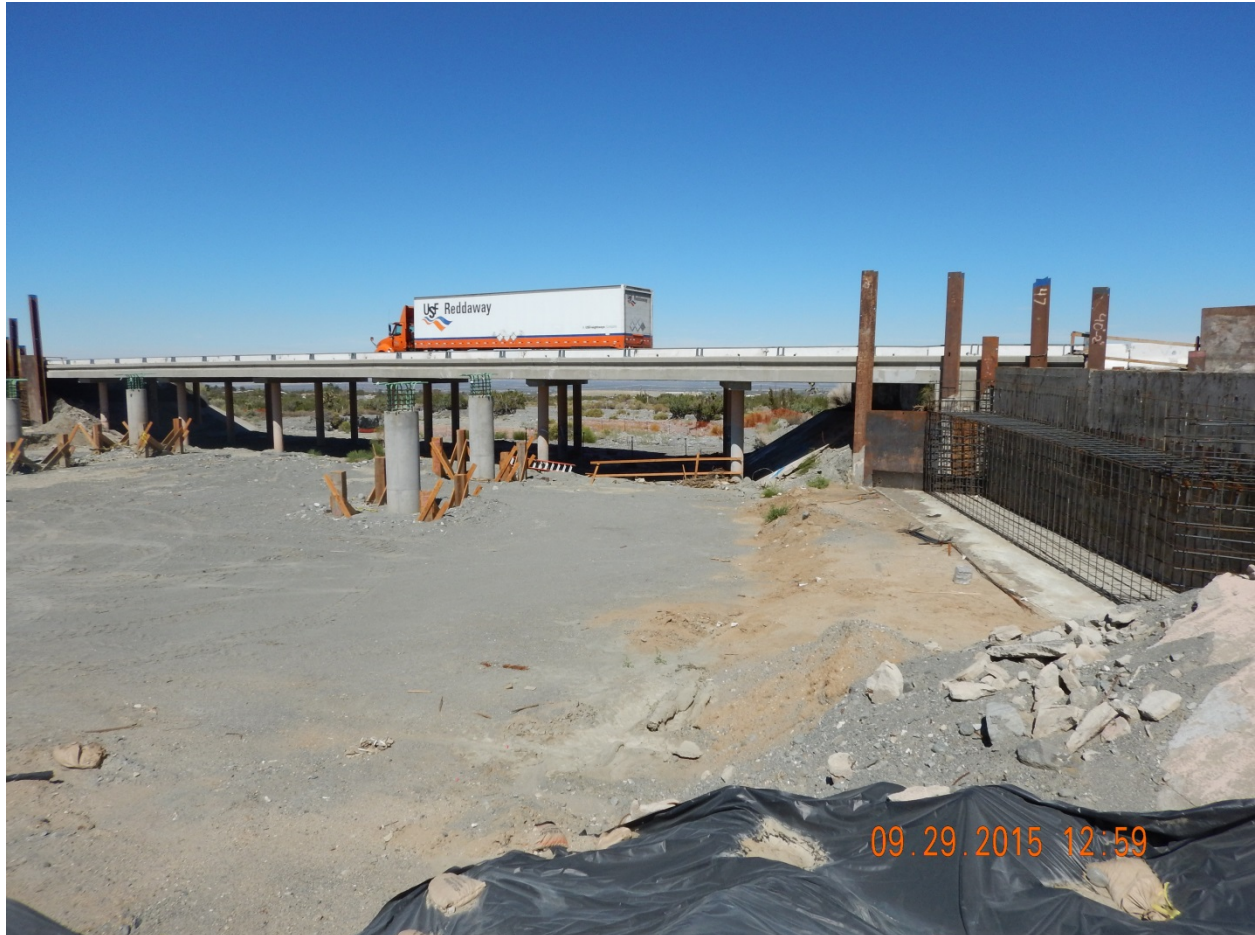
Picture 19: View North Within Sheep Creek. Note Extensive in-channel work and inadequate BMPs.
