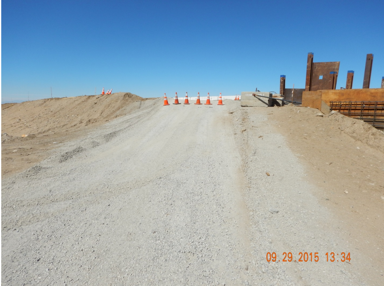
Picture 31: View facing north along construction access road (west of Sheep Creek) to active paving activity along the SR 138 alignment.
