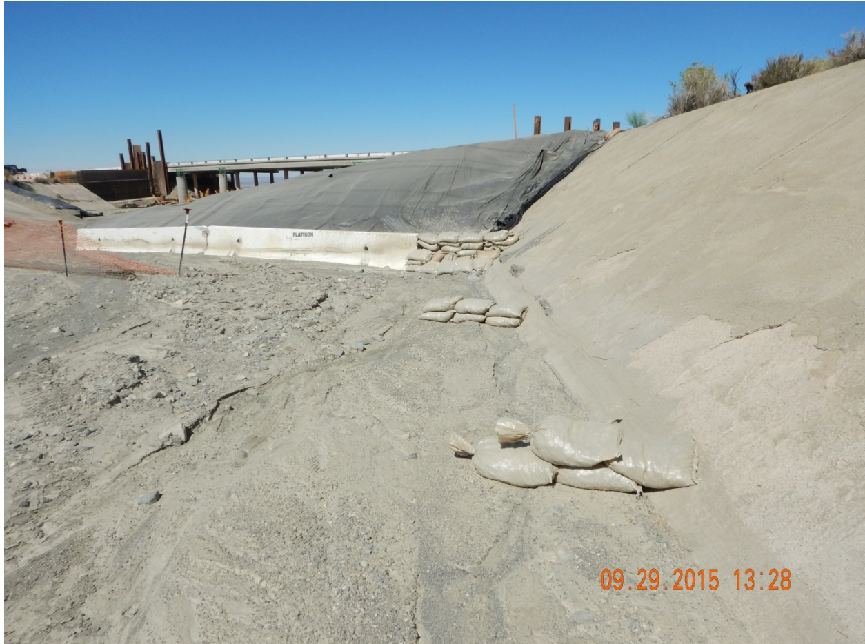
Picture 29: View North from within Sheep Creek. Note that the k-rail does not extend far enough to the west to protect the toe of the access road.
