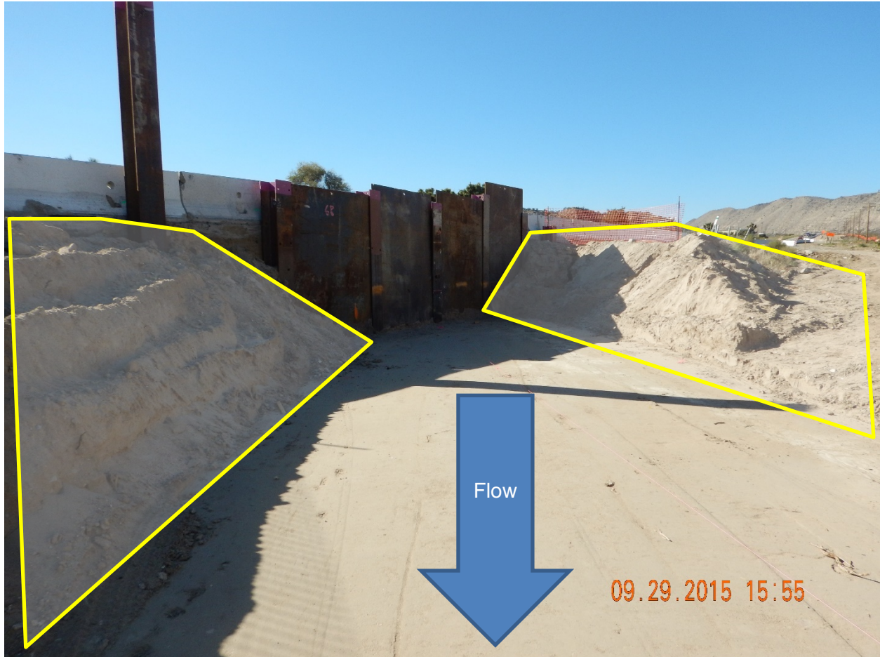
Picture 9: View West at Drainage ID 16. Note the un-stabilized stream banks and absence of erosion and sediment controls (approximate areas in yellow boxes). Additionally the stream has been completely disconnected from upstream flow with metal sheet pilings.
