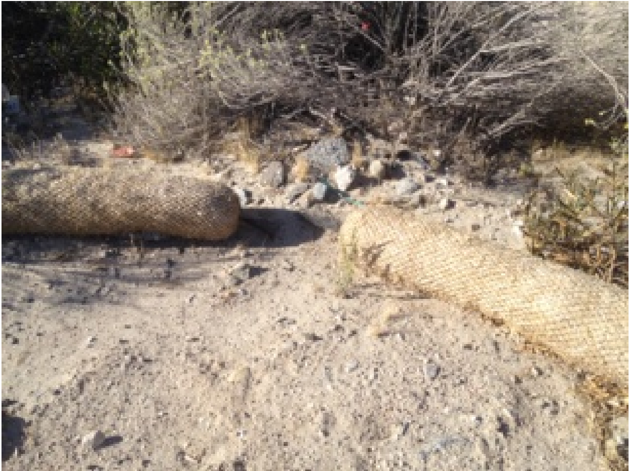
Picture 12: View of gap in wattles adjacent to Drainage ID 1b.
