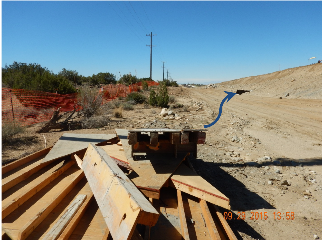
Picture 6: View West of unpermitted temporary impact at Drainage ID 55. Note the access road parallel to road construction and fill within the stream channel. Flow path and direction shown with arrow.
