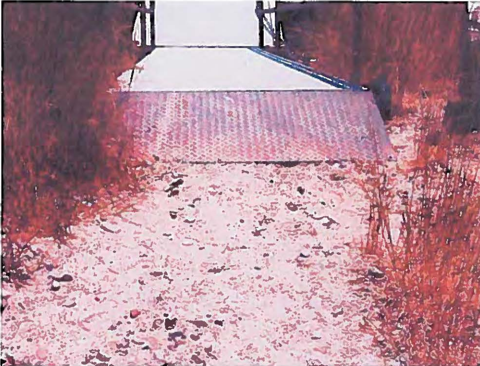
Picture 2: The walkway is downward sloping from the parking lot to the gangways. Potential for rill or gully erosion into the marina surface waters is possible.
