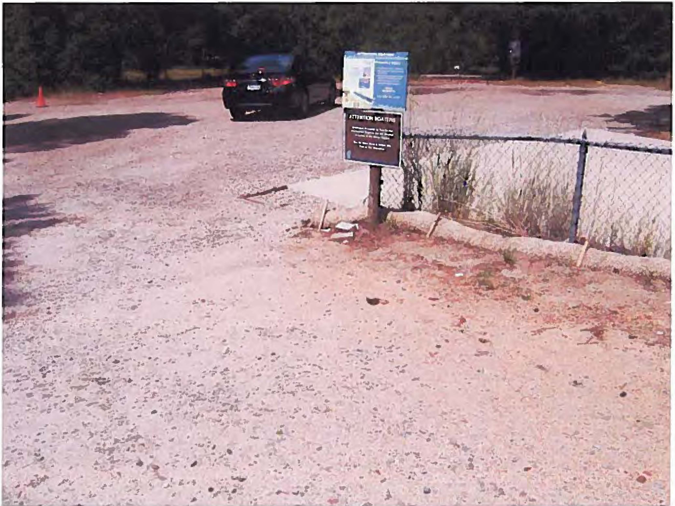
Photograph 04 - Looking East, Northeast at fiber roll. The fiber roll is not J-Hooked at its end which is also installed perpendicular to the grade lower than the rest of the fiber roll, and not parallel to the grade. Any runoff that flows toward the fiber will flow along it toward the downgradient end and, eventually, down the boat ramp and into the marina.
