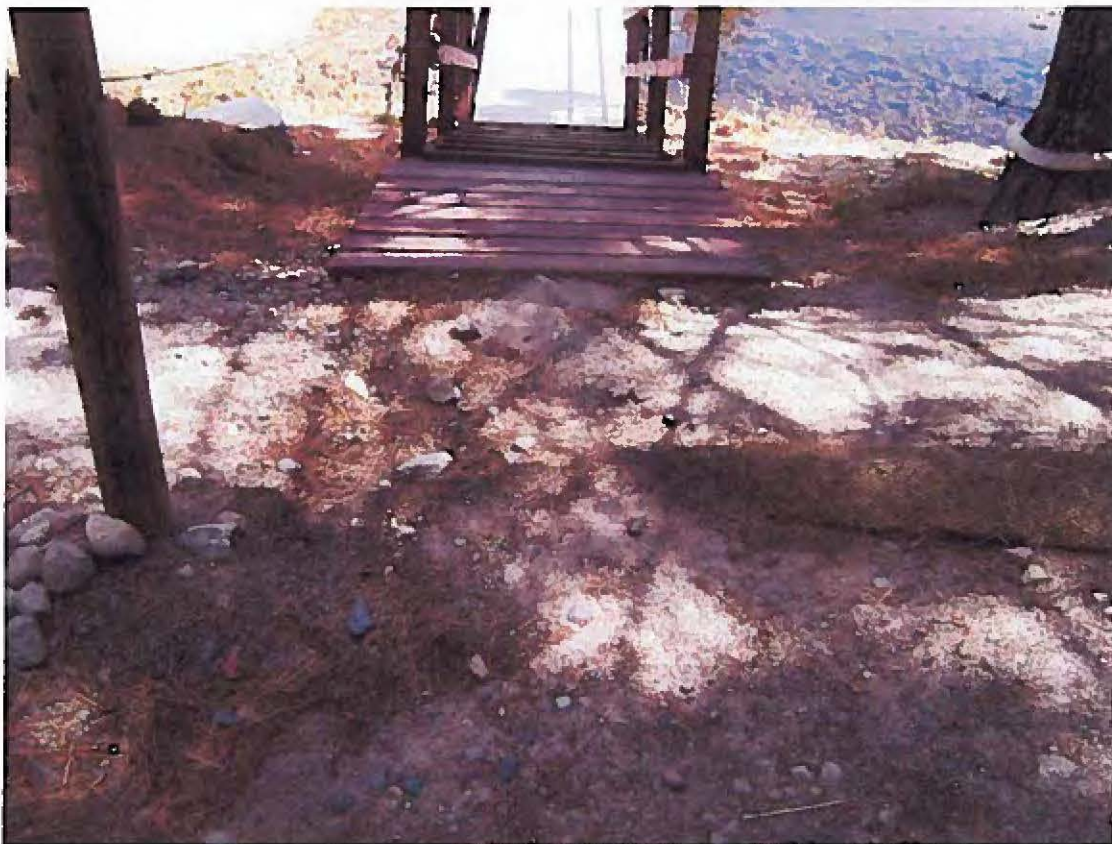
Photograph 22 - Close up of the sediment-inundated fiber roll shown in Photograph No. 20, also showing sediment deposits down along the embankment and into Lake Tahoe.
