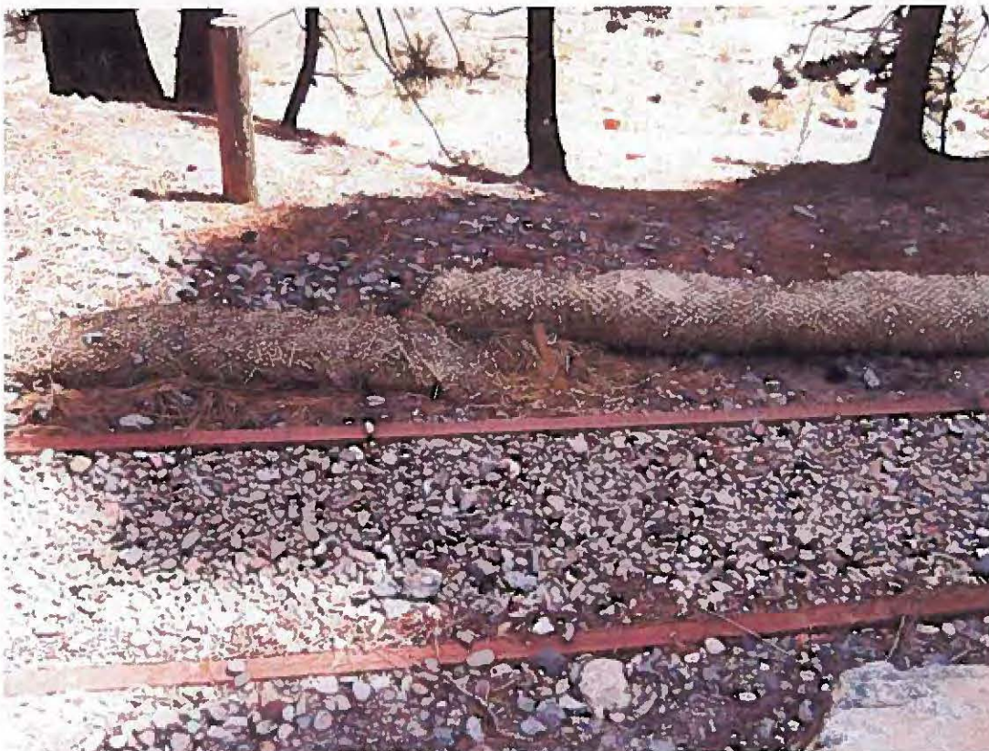
Photograph 18 - Midway between 3rd and 4th ramps west of office. The ends of the fiber rolls are degrading, and they are barely overlapped.
