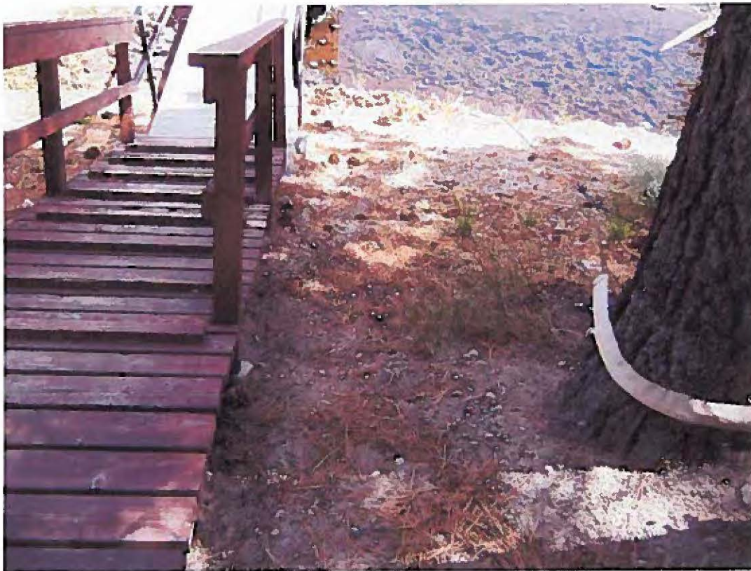
Photograph 24 - Close-up of the west side of the 4 th walkway shown in Photograph No. 20. Evidence of erosion can be observed.
