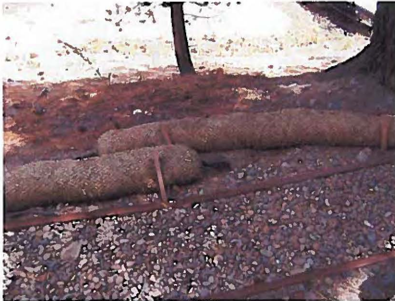
Photograph 19 - West of photo 18, between 3rd and 4th ramps west of office. In this area, the fiber rolls are adequately overlapped.
