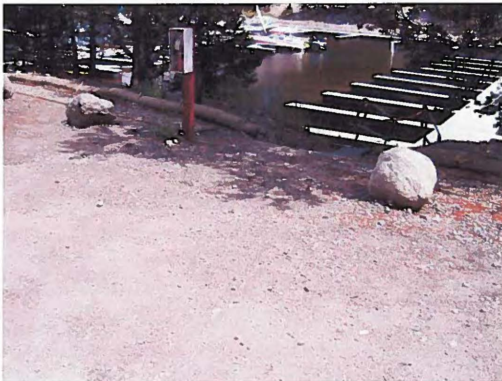
Photograph 08 - Second ramp west of office, facing southeast. Fiber rolls do not prevent runoff from going down ramp and into marina.
