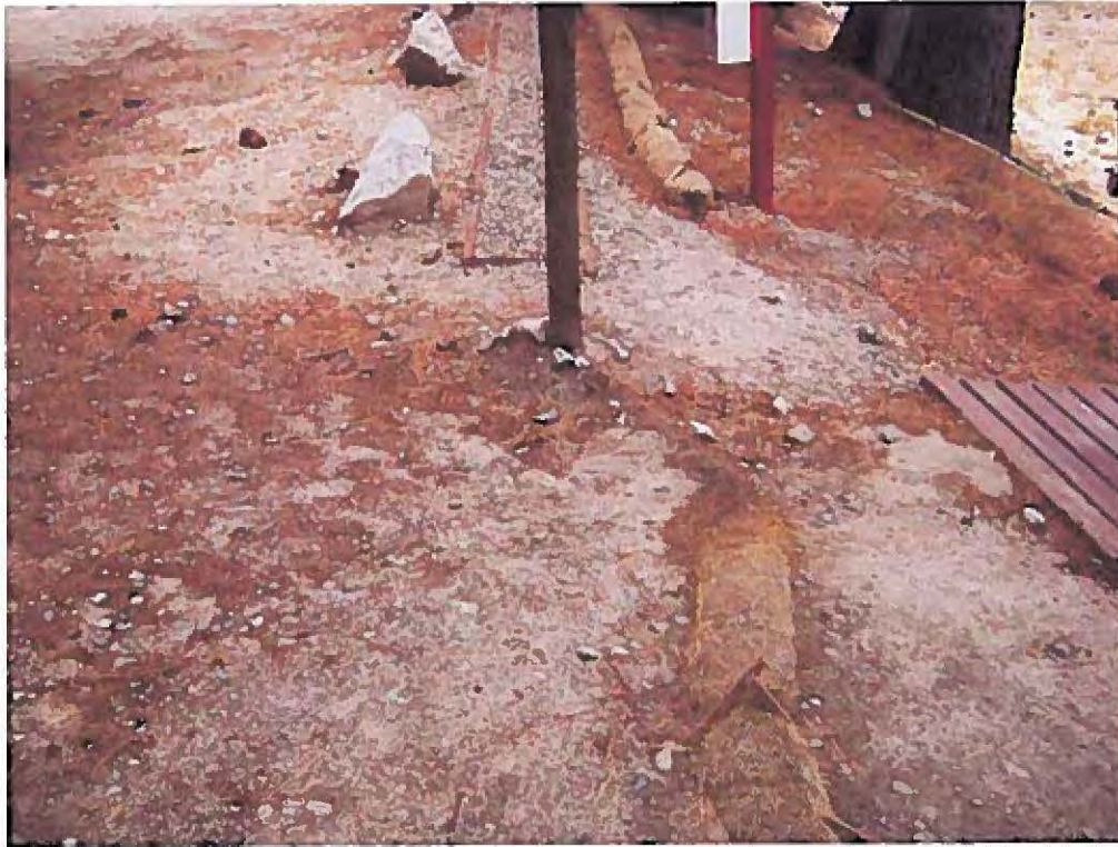
Photograph 23 - Close up of the sediment-inundated fiber roll shown in Photograph No. 20, facing east. The fiber roll end in the foreground was slightly J-Hooked to capture runoff and sediment, while the end of the fiber roll at the top of the photograph is not J-Hooked and allows runoff to flow down the embankment. Photograph taken by Will Chen.
