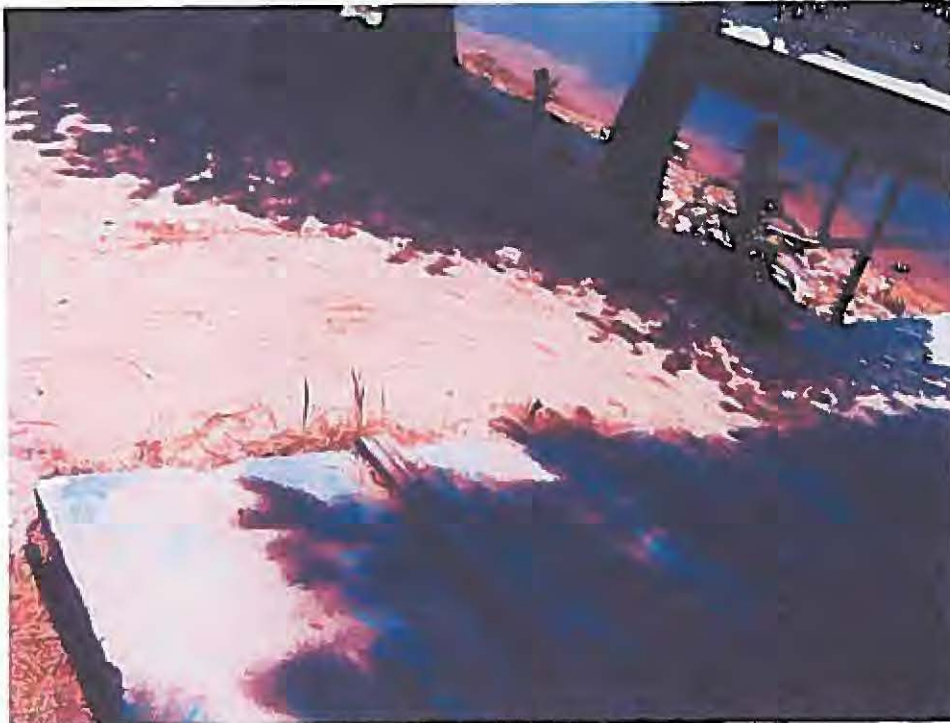
Picture 4: This is gangway number 1, closest to the lake. Due to the topography of the parking lot, a low spot forms at the top and runs down during significant rain events.
