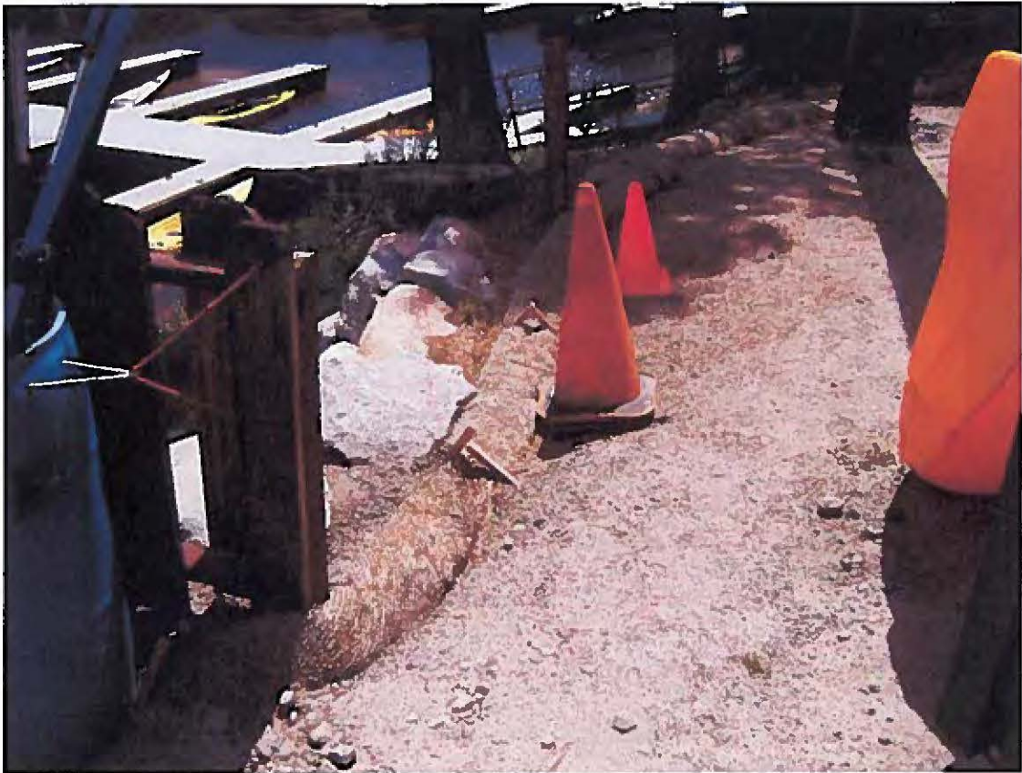
Photograph 05 - Flattened fiber roll adjacent to marina office, facing southwest. Also, the end of the fiber roll is installed perpendicular to the gradient, which will channelize storm water runoff.
