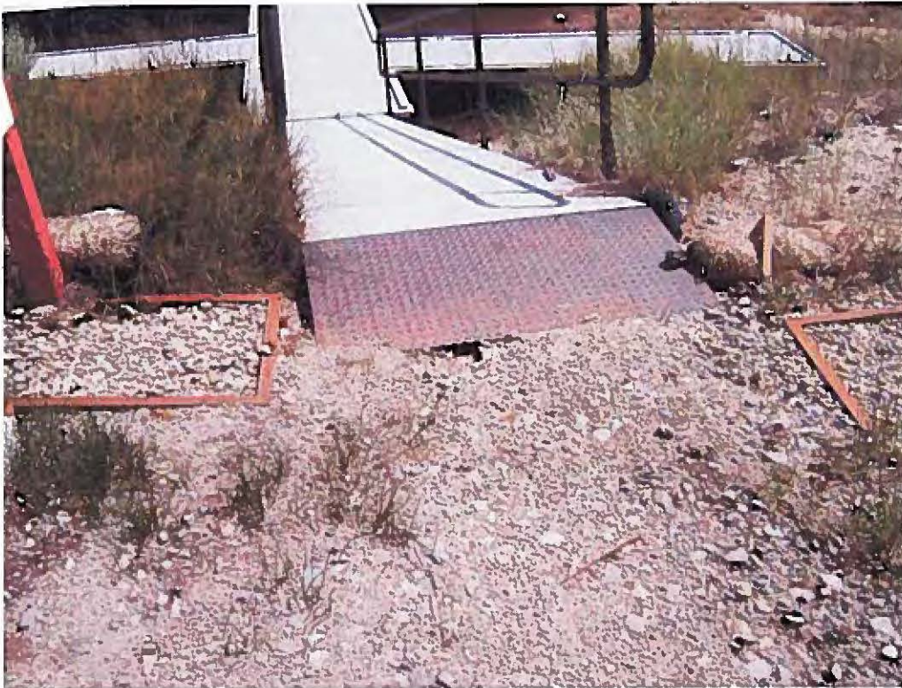
Photograph 17 - 3rd ramp west from office, facing south. A rill has formed beneath the metal plate, creating a threatened discharge of sediments into the marina. No fiber rolls or other BMP exists to prevent runoff from flowing down this area and causing bank erosion.
