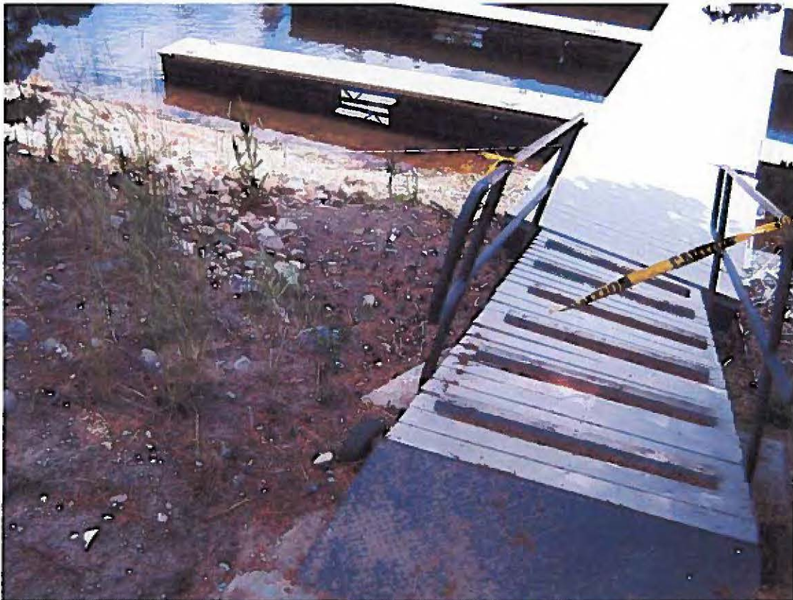
Photo 12 - Moving closer to the second ramp west of office to get a further close up within the marina area. Note that the fiber rolls were unable to prevent runoff from going down ramp and into marina, as evidenced by a sediment deposit in marina located on left (east) side of ramp.
