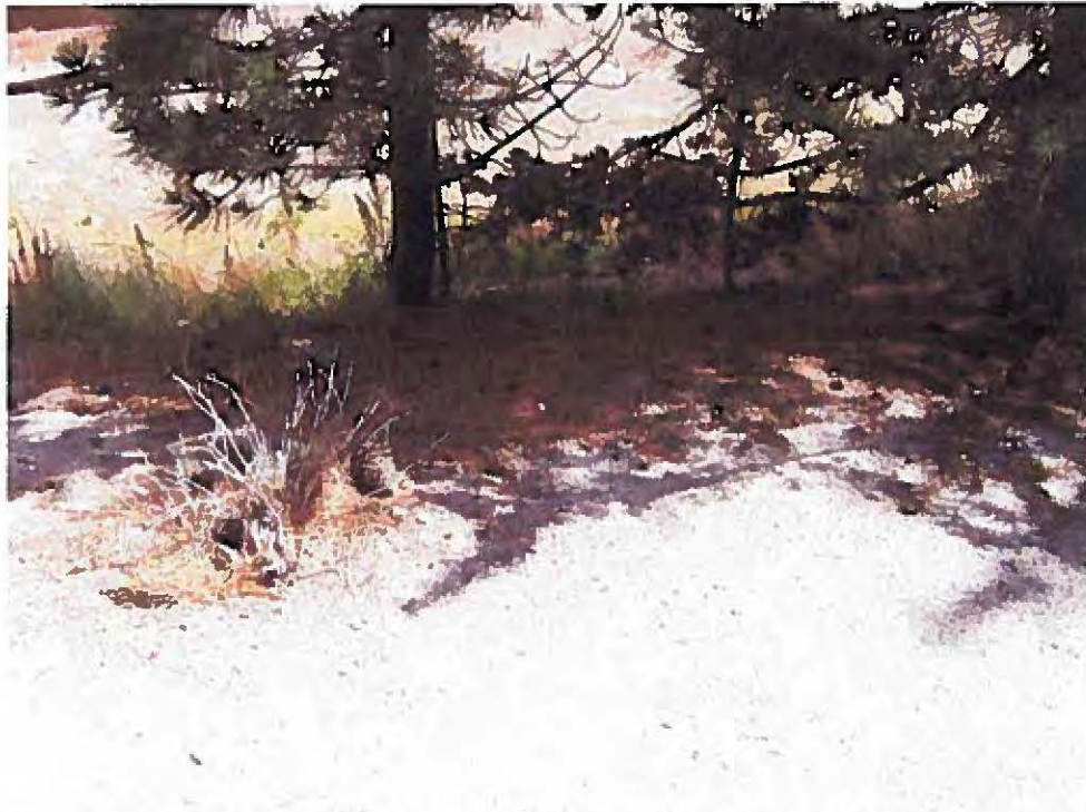
Photograph 29 - Standing at photo point 28, looking southwest. Fiber rolls have not been placed to collect potential stormwater runoff from the unpaved parking area.
