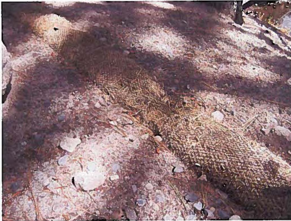
Photograph 25 - 10 feet west of the 4 th walkway west of the office. The fiber roll has degraded.
