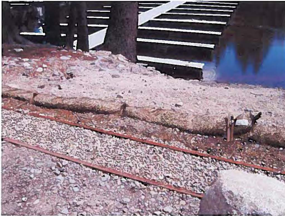
Photograph 15 - About 20 feet west of 2nd ramp west from office, looking south-southeast. The fiber roll has been degraded degraded and flattened.
