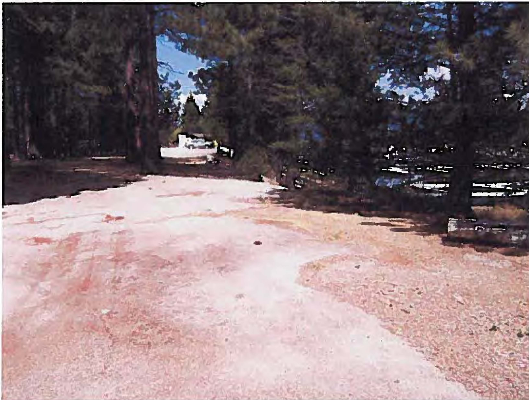
Photograph 32 - At west end of the marina boundary in the boat trailer parking area looking east. Fiber rolls were not installed at trailer parking area. Note the evidence of ponded water in the middle of the photograph, indicating fiber rolls may not be necessary in this area.
