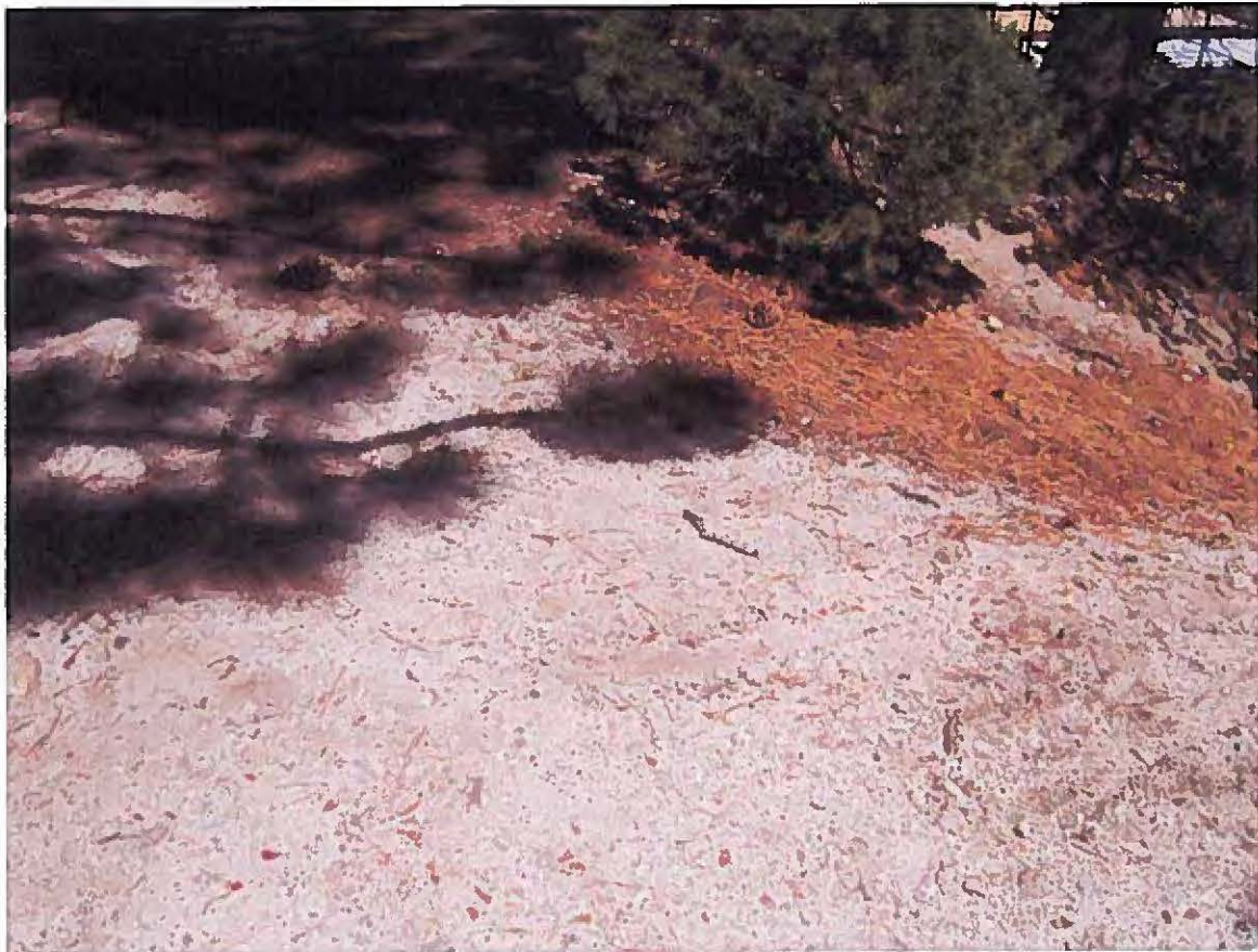
Photograph 26 - 20 feet west of 4th walkway ramp from office, facing east. No fiber roll has been installed, and a small gully erosion can be observed.
