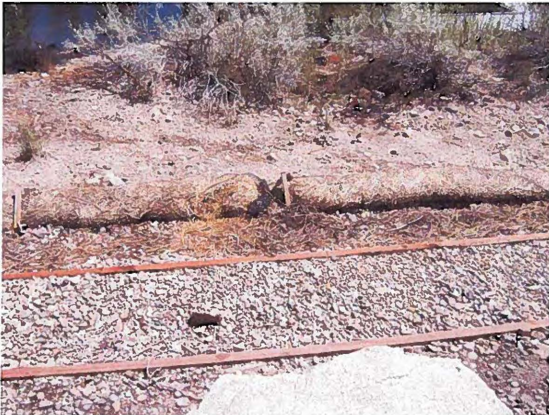
Photograph 16 - Mid-way between 2nd and 3rd ramps west from the office. The fiber rolls have been slightly flattened, and the ends have not been overlapped leaving a gap between the rolls where stormwater runoff can become concentrated.
