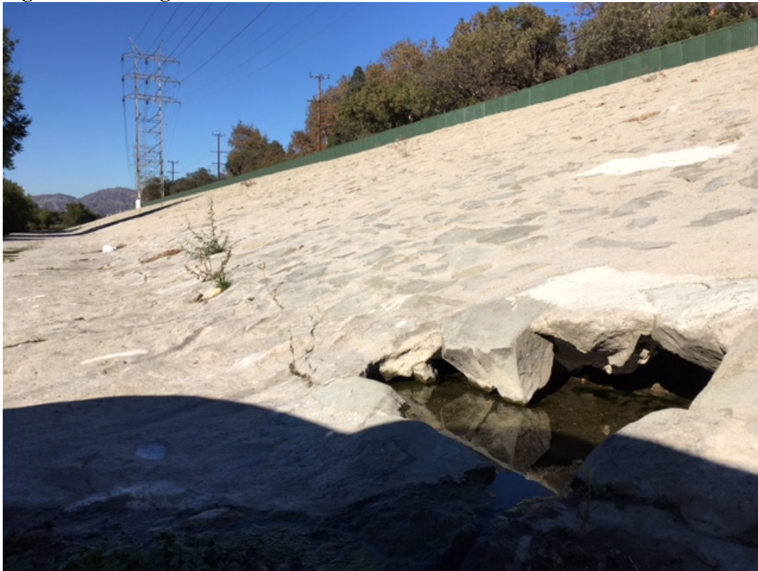
Figure 3. Los Angeles River – Hole in Levee Embankment
