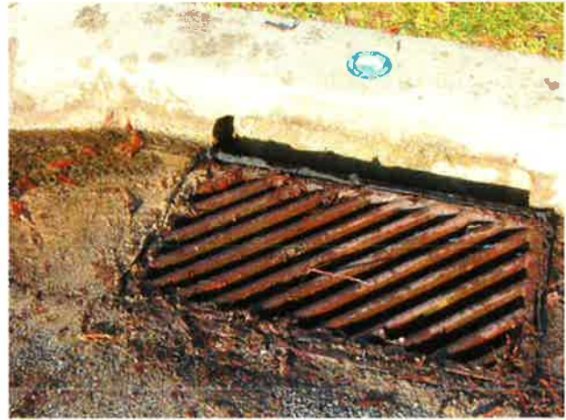
Figure 3. UltraDrainguard-protected inlet showing water flow bypassing the filter and entering the curb opening.
