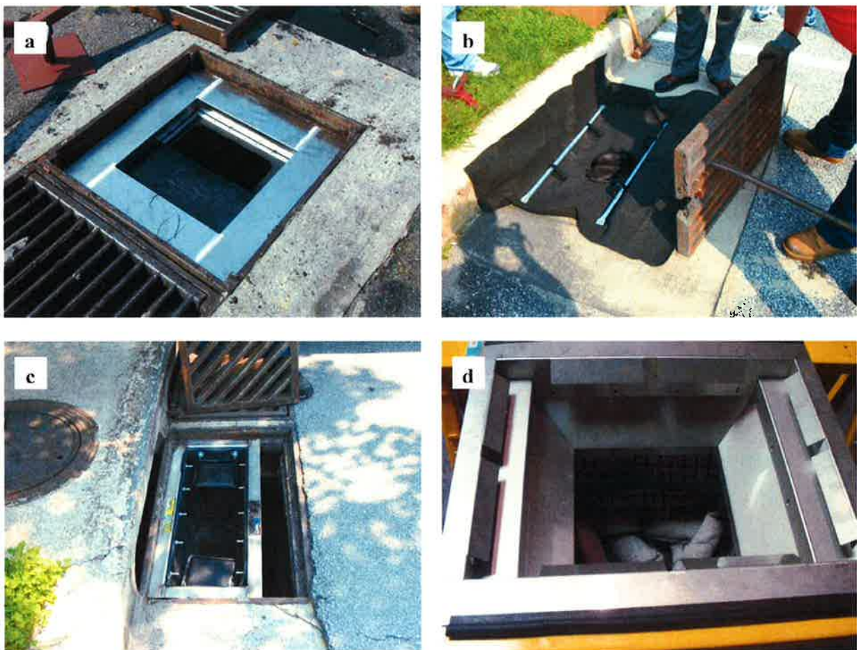
Figure 1. Photographs of installed catch basin inserts. (a) HydroKleen units at the I-95 service plaza; (b) UltraDrainguard filters at the service plaza; (c) DrainPac inserts in Drummond North subdivision; (d) FloGard Plus units at the Wilmington Riverfront.
