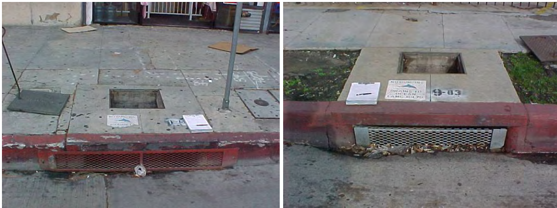
Figure 4-20. Curb inlet screens installed at two sites: FL003-F (left) and CC004-H (right).
