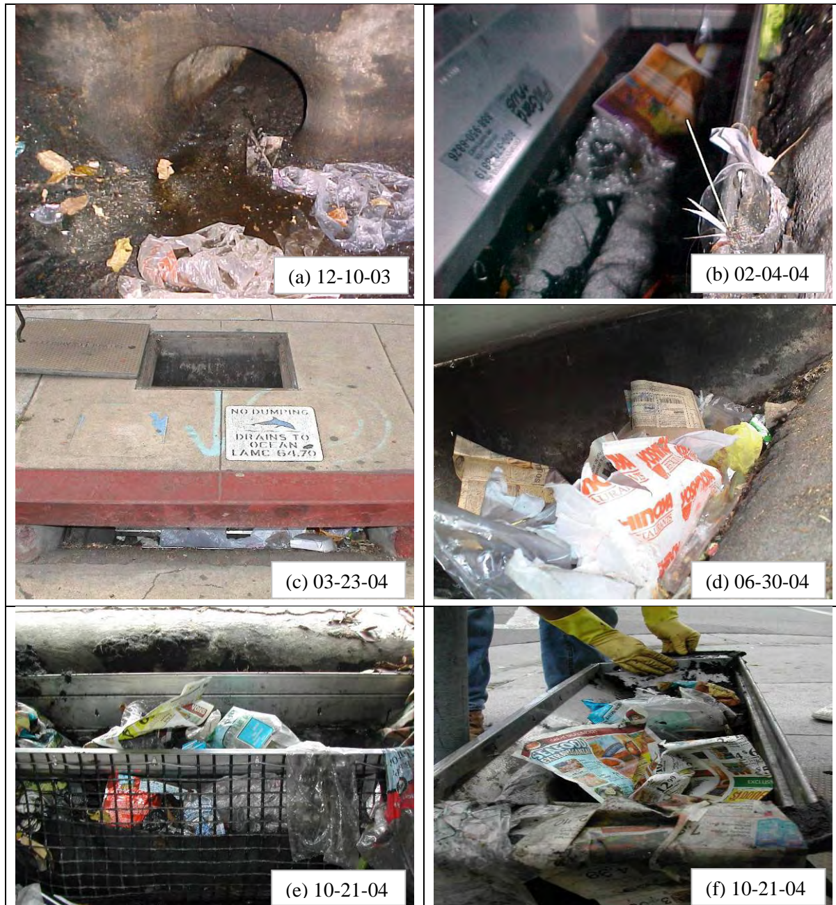
Figure 4-12. Field inspection photos showing the condition of FloGard Plus at the intersection of 18th St. and Flower St. (southwest corner).
