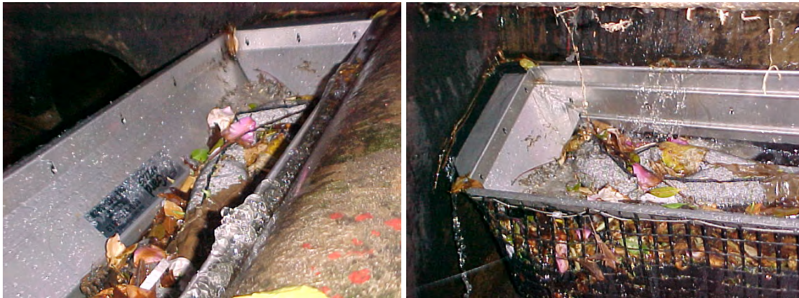
Figure 4-18. Improper installation of insert that caused bypass (CC-003-F, 2/4/04).
