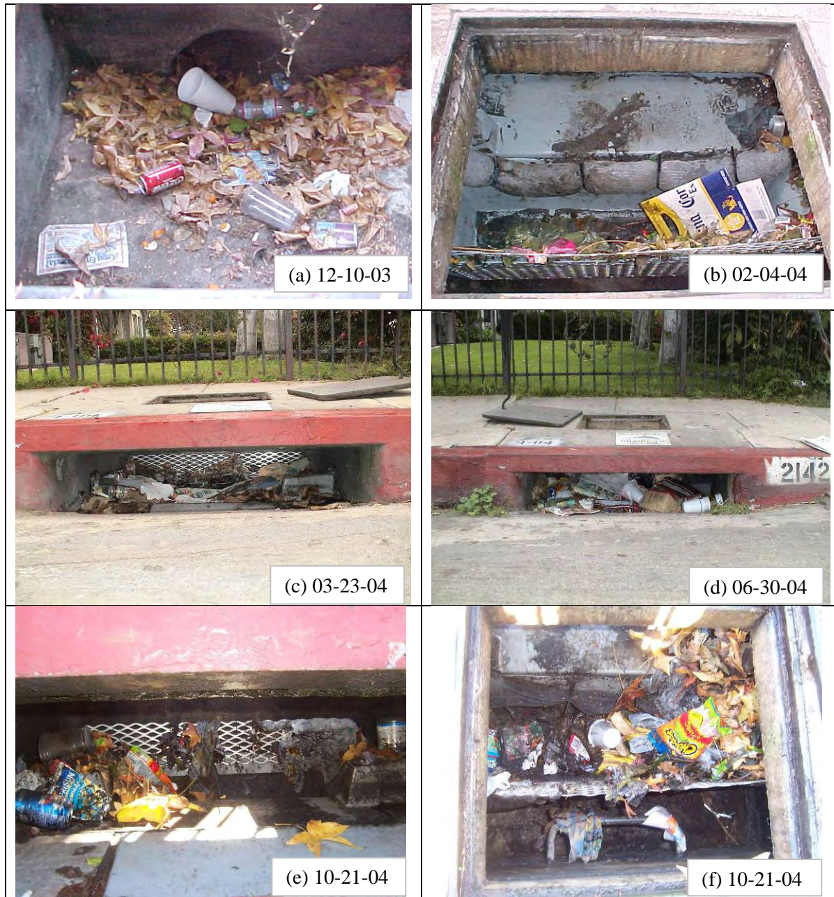
Figure 4-8. Field inspection photos showing the condition of Curb-Inlet Basket at the intersection of 23rd St. and Portland (east side).
