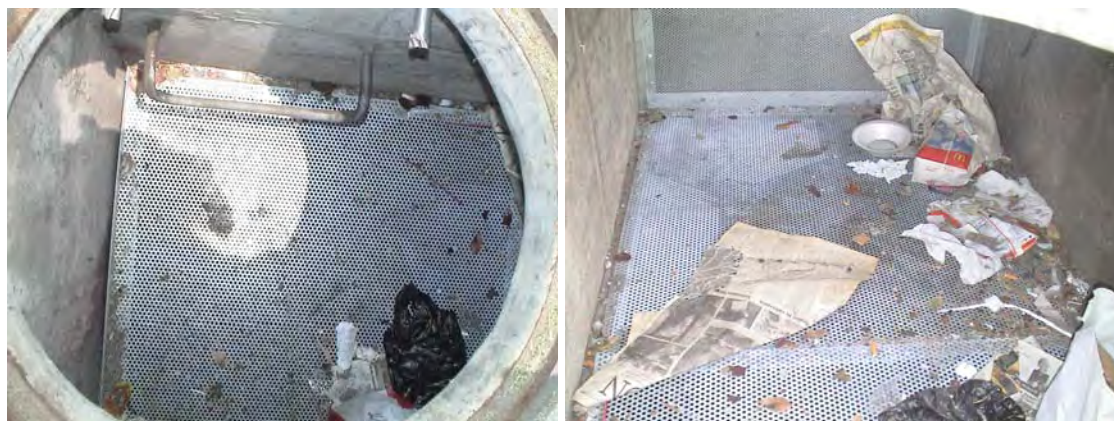
Figure 3-5. Alternative catch basin insert system installed by the City of Los Angeles.
