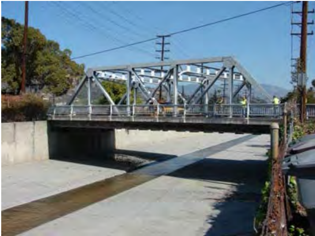
VW_CON Ground-Level View
