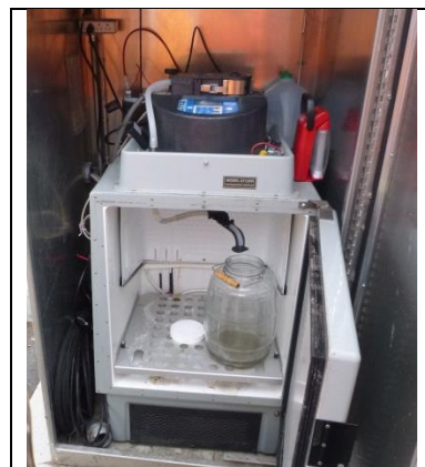
Figure 1. ISCO Type Automated Flow and Sampling Equipment Installed at Existing Monitoring Stations
