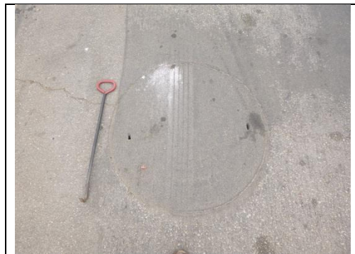
Figure 2-2. Currently No Safe Access to Former Watershed Station MdR-2
