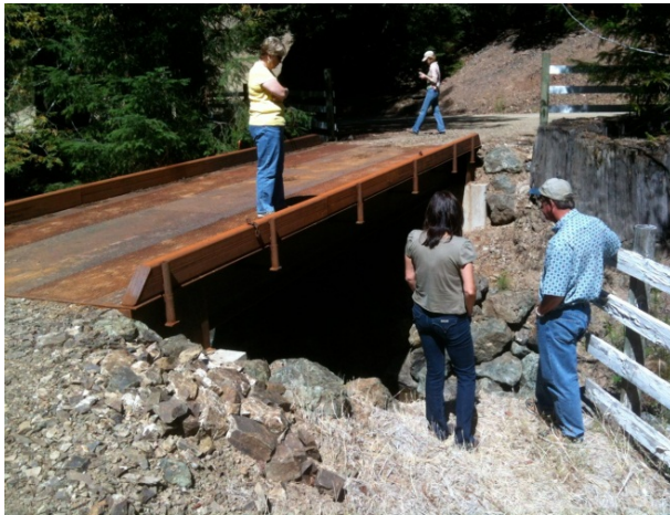
Mendocino RCD and Natural Resources Conservation Service partners inspect a new bridge installation to improve fish passage on Monahan Creek. Photo by Jonathan Warmerdam. August 2012
