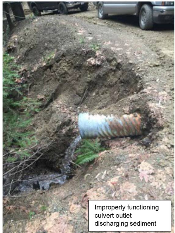
Image 2: An example of a stream crossing culvert outlet that needs to be replaced to repair scour and prevent erosion and sediment transport.
