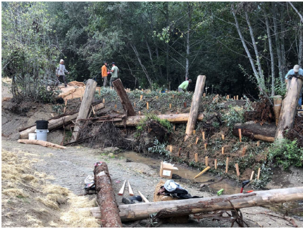
The Ten Mile River Restoration Project: crews installing brush mattress, willow poles, and final erosion control at the Island Head fill area. Photo courtesy of the The Nature Conservancy.
