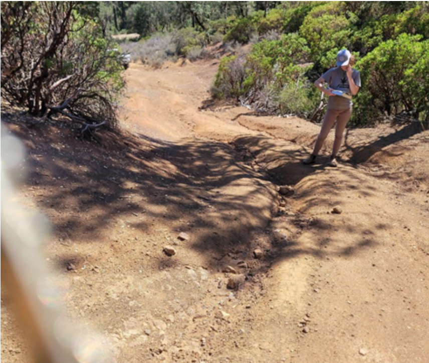
Figure 2: Typical deteriorated road in Post Mountain community
