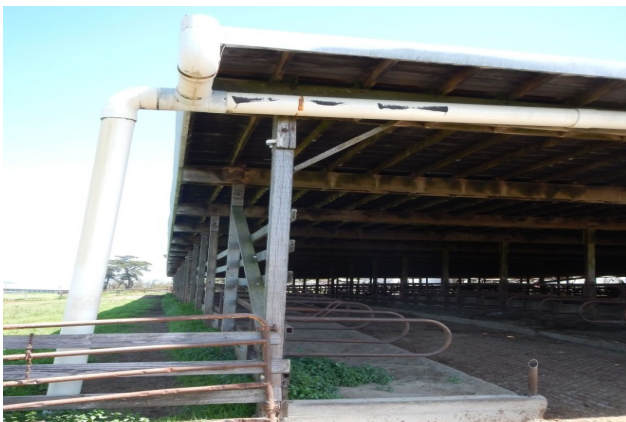
Roof gutter system diverts clean rain water away to optimize needed space in the manure ponds. Sonoma County. Photo by Cherie Blatt.
