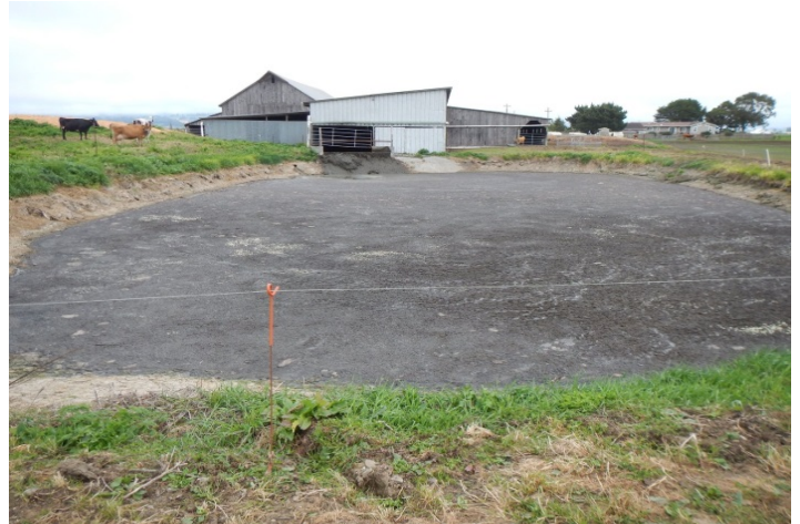
Keeping vegetation trimmed around manure ponds makes it easy to check for leaks or cracks. Humboldt County. Photo by Cherie Blatt
