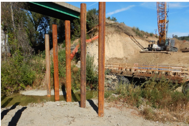
Photo 1: HWY 20 Calpella Bridge replacement project along the Russian River in Ukiah, October 2022
