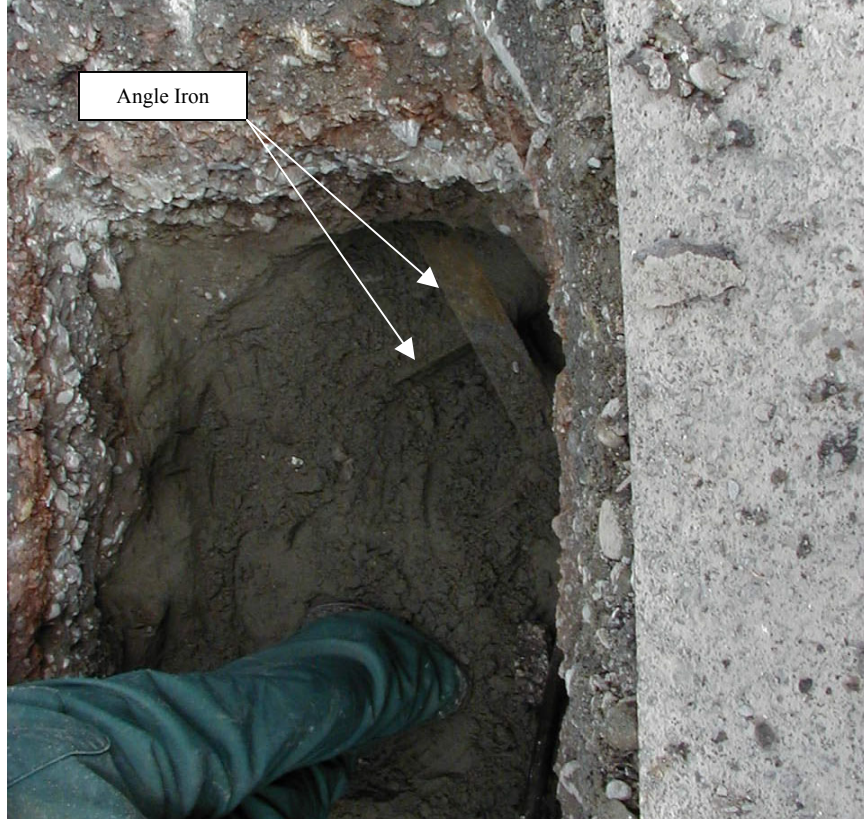
Photograph 7 – Shows angle iron along north (top) side of the excavation at Anomaly B.
