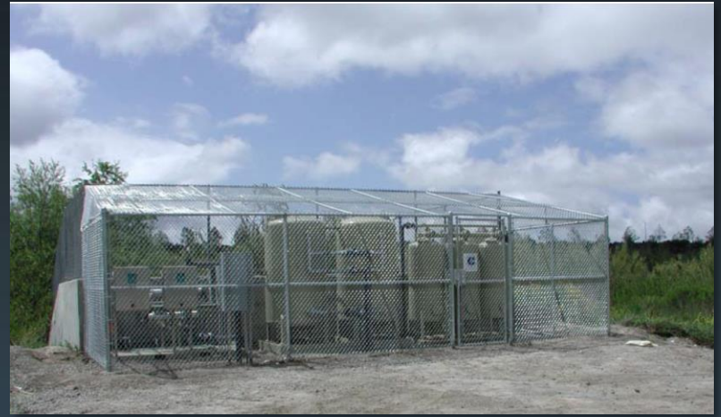
Source: Photo of Aliso Creek Bacteria Treatment Facility (County of Orange, 2005)
