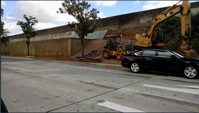
Source: Photo of Caltrans filter project, 210 Freeway in Pasadena (Paulsen, Dec 2014)
