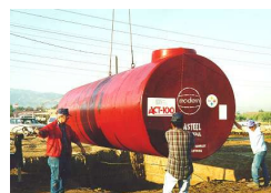
Underground storage tank
