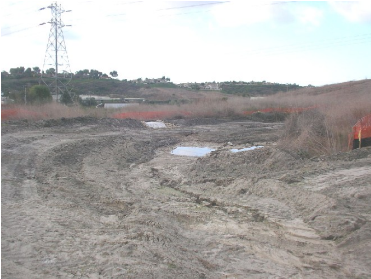
Photo 1 Example of Sediment Trap (Facing South)
