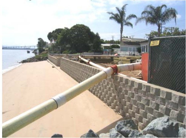
Figure 2. Post construction shoreline condition, with un-permitted seawall construction, and discharge of fill material (beach sand)
