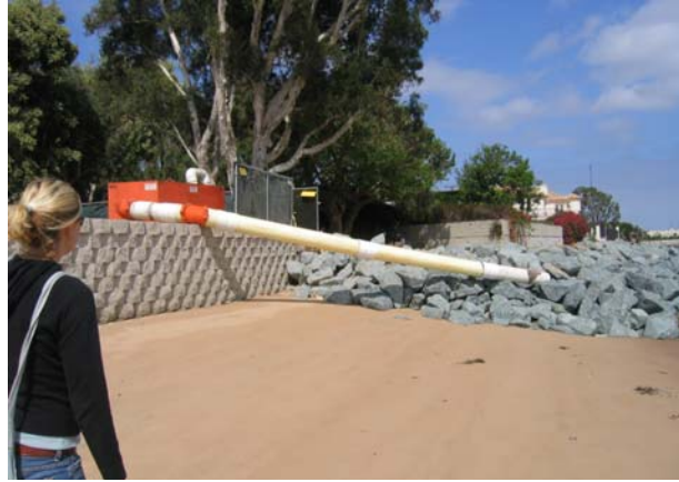
Figure 6. It is unknown what the pipe shown here is discharging offsite into City of Coronado Project footprint (possibly used to spread sand on constructed beach?)
