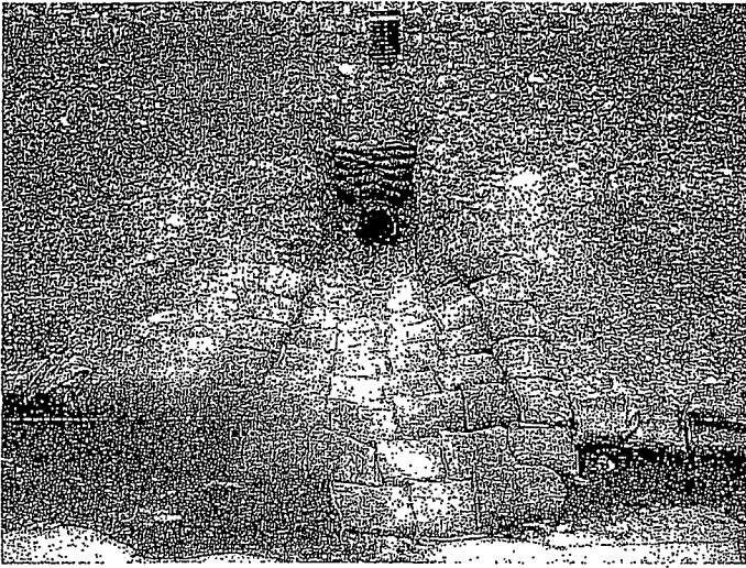
156. A runoff discharge point upstream to the east of the culvert in photo 153. Sediment-laden runoff flows out of the pipe across the gravel bags and into the plastic lined ditch.
