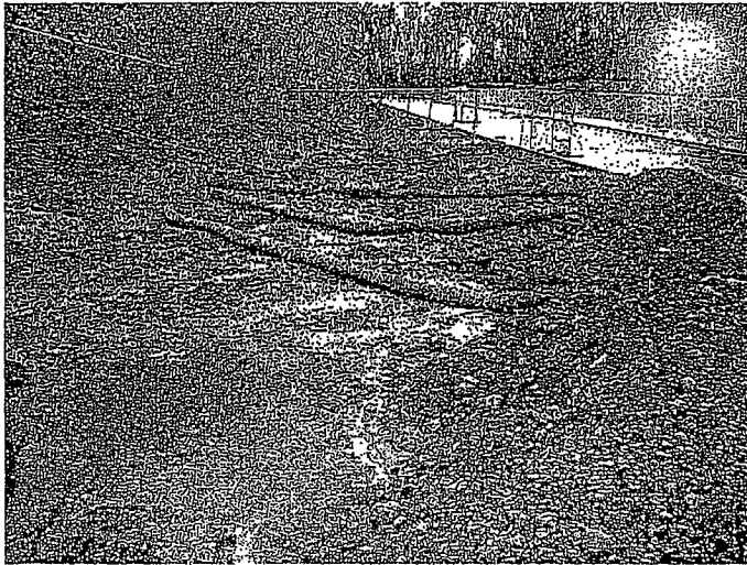
154. Upstream of the culvert entrance on the western side, no erosion controls have been implemented. Fiber rolls have not been trenched in and staked therefore they are doing little to stop the sediment flows.
