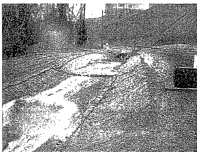
150. Photo is looking upstream of the discharge in photo 149. Sediment-laden runoff is flowing from a storm drain culvert outlet pointed out by the arrow.
