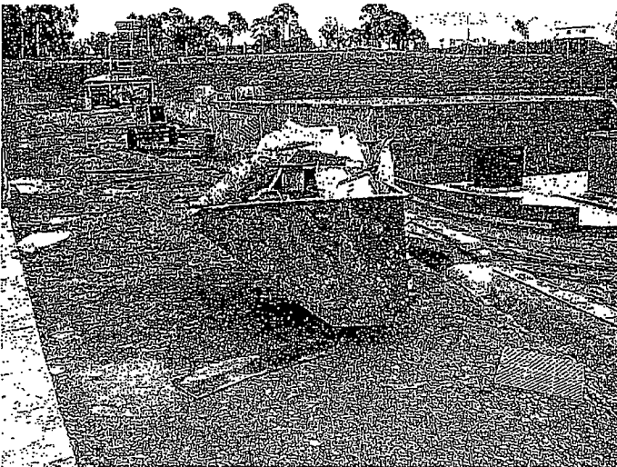
204. Construction trash is not covered to minimize contact with storm water.
