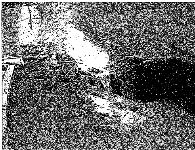
152. This is the culvert entrance to photo 151 on the south side of Avenue of Nations receiving sediment-laden runoff.
