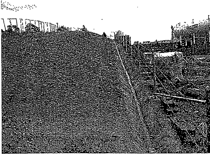
178. Upstream of the inlet in photo 177, the slope has no sediment controls along the toe of slope or in the concrete v-ditch.
