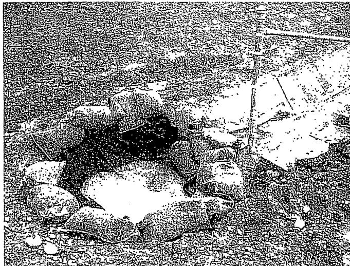
177. A storm drain inlet with sediment laden water.
