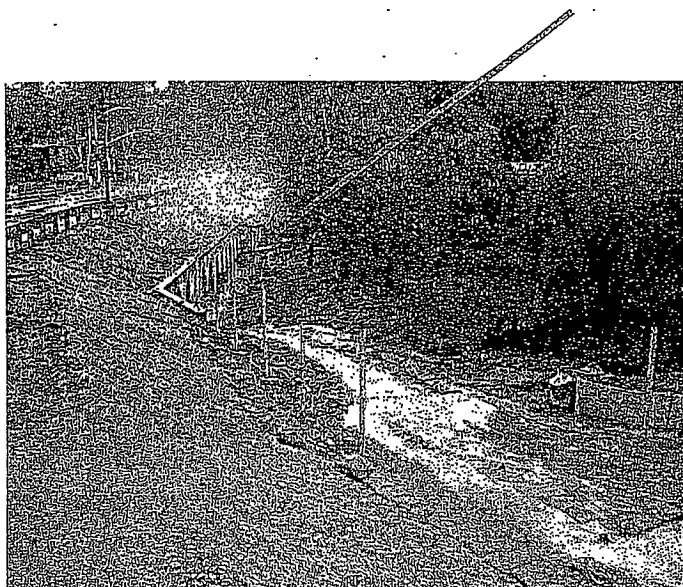
149. Sediment and sediment-laden water entering Carroll Canyon Creek. Arrow points to the culverts for Carroll Canyon Creek going under Avenue of Nations.
