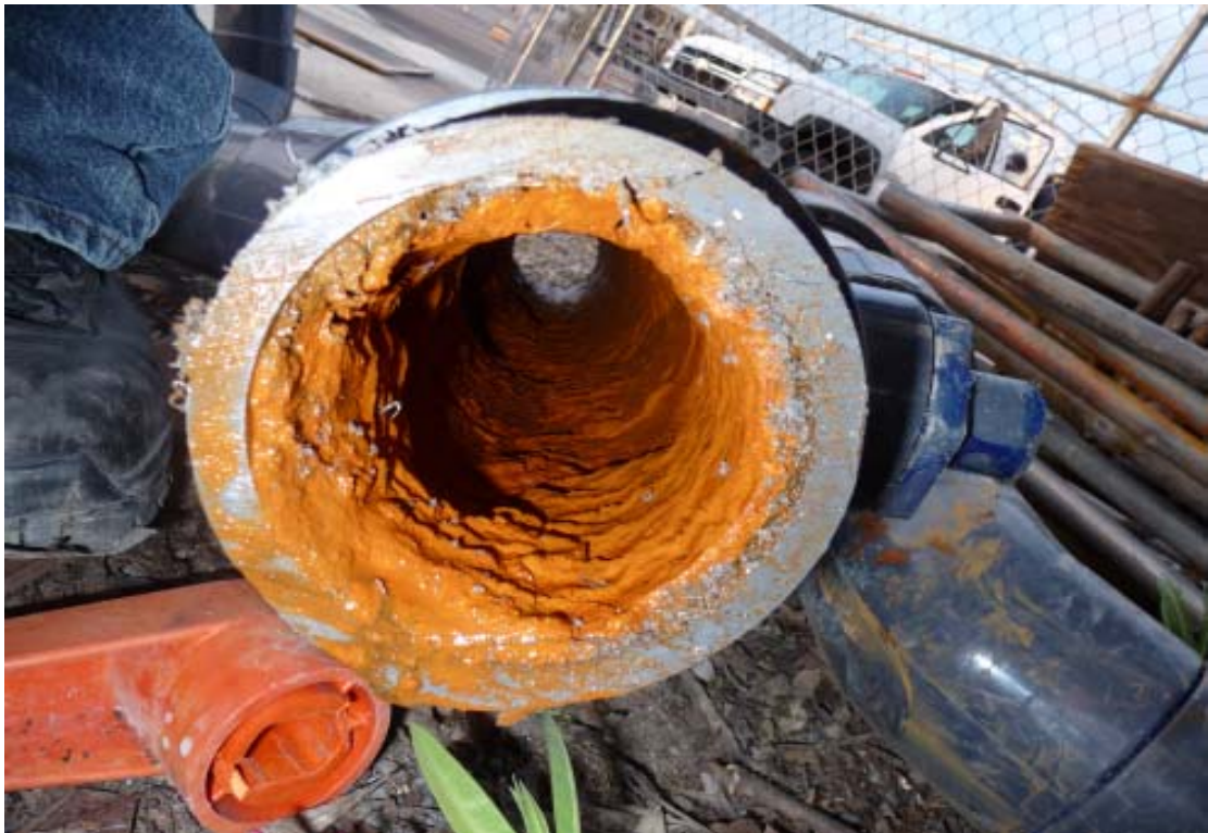
2. Fouling on Extracted Water Conveyance 2.
