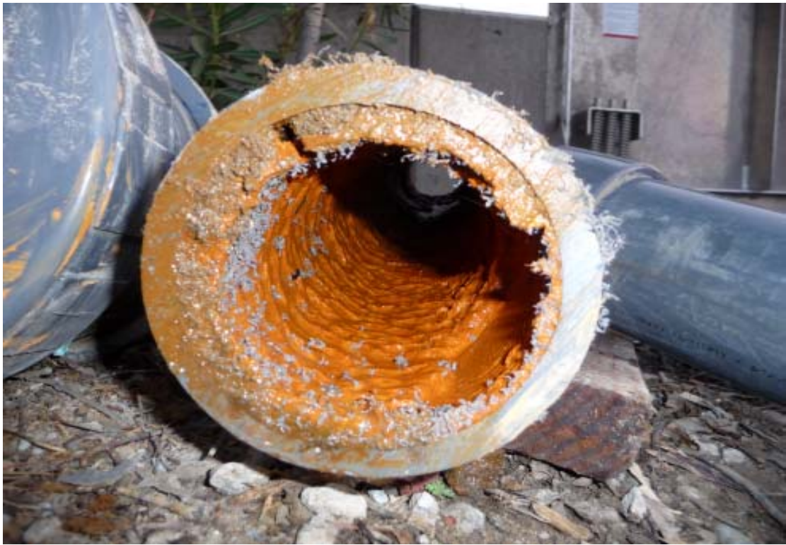
1. Fouling on Extracted Water Conveyance 1.
