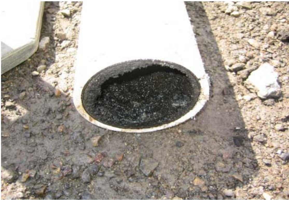
3. Mineral Fouling on Treated Discharge Pipe 1.
