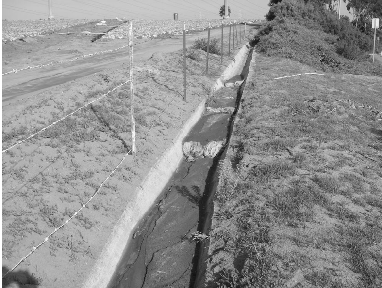
Figure R-5. Use of Sandbags near Strawberry Fields, Cannon Rd. near Interstate 5, Carlsbad Watershed.
