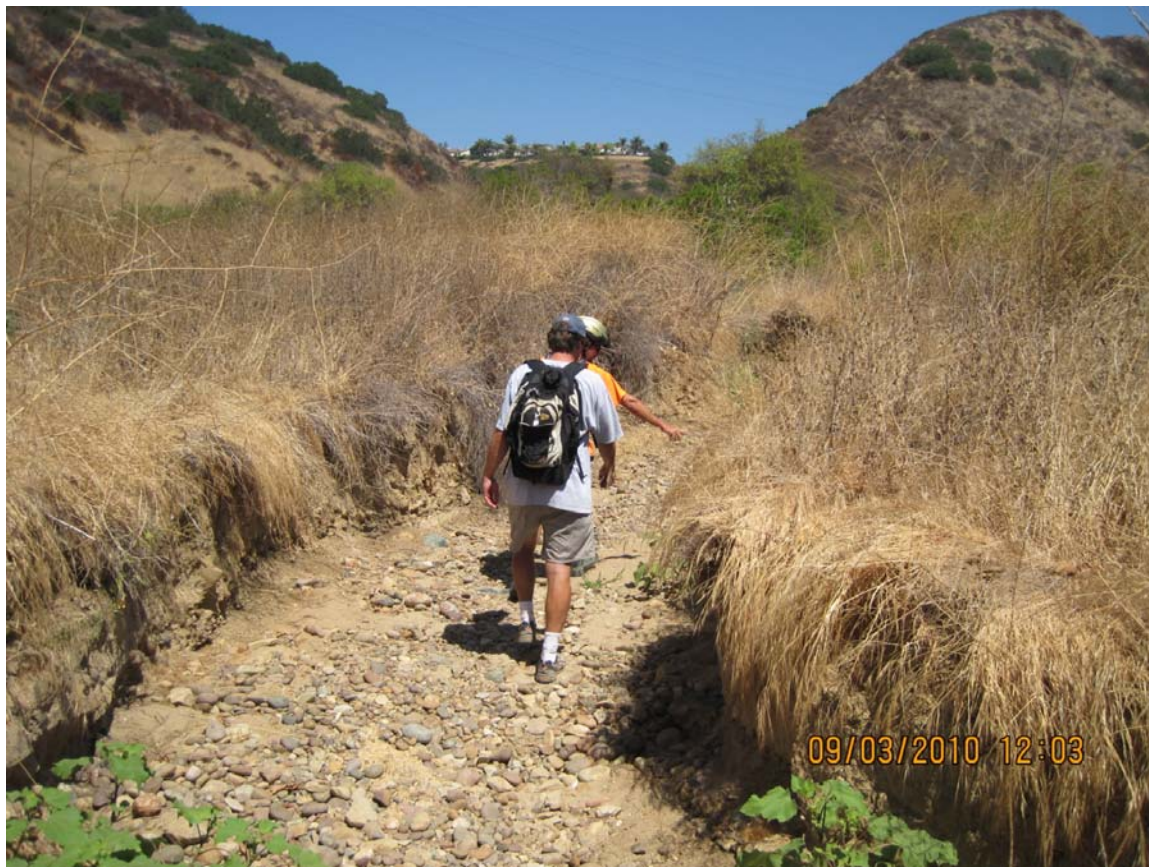
Figure 16. Erosion of canyon walls below storm drain outfall in the Los Peñasquitos Creek watershed (Garrity and Collison, 2011).
