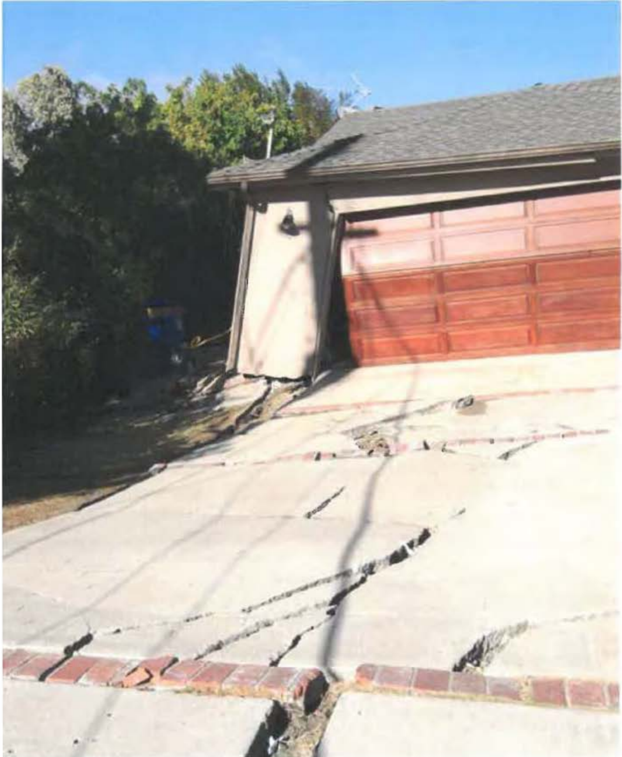
Photo 2 – La Jolla landslide (Ardath Shale Formation, Claystone, Hydrologic D)
