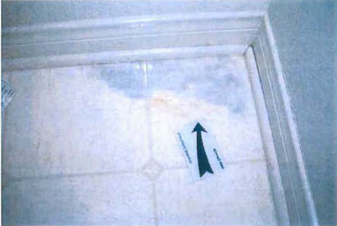
Photo 5 – water migration through slab (mold under vinyl flooring)
