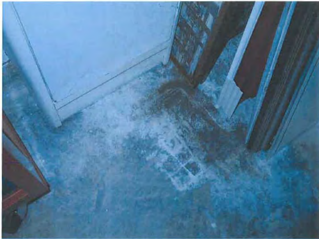
Photo 6 – water migration through slab (white coating is efflorescence)
