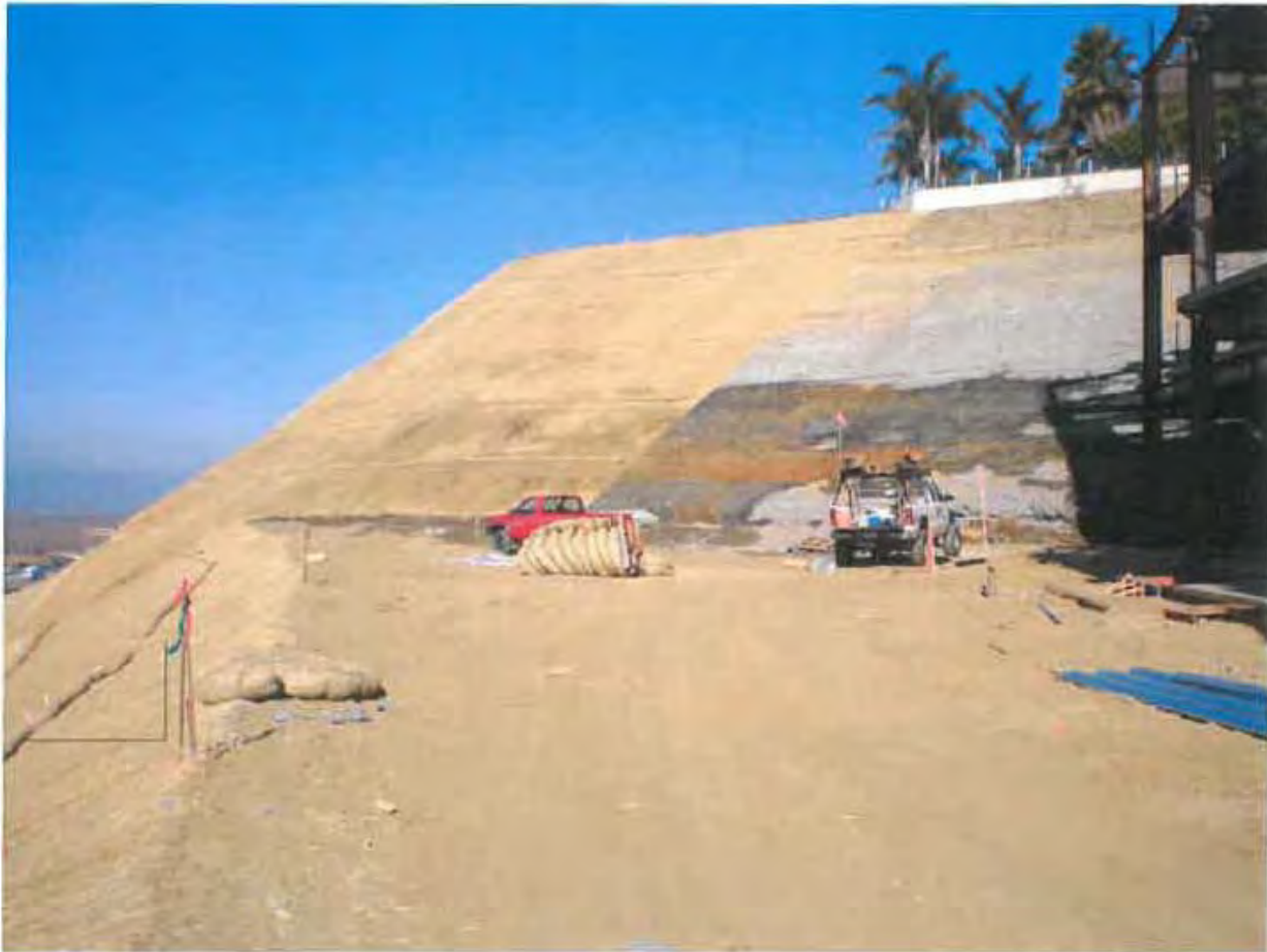
Photo 3 – Perched water visible on lower half of hillside (water migration)
