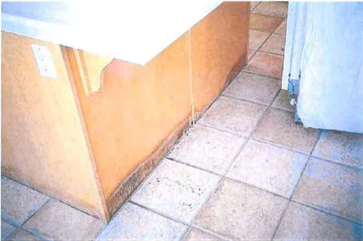
Photo 4- water migration through slab into cabinetry
