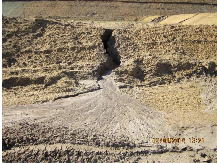
Photo 3. Evidence of erosion at edge of a lot
