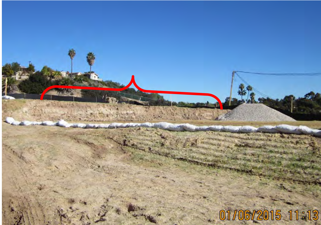
Photo 5. Sidewall without adequate erosion control
