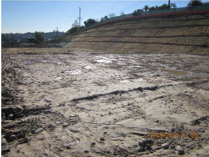
Photo 1. Lot lacking erosion control BMPs
