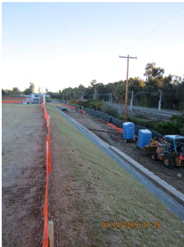
Photo 4. Rills filled in, area re-hydroseeded, silt fence added to perimeter of lot.
