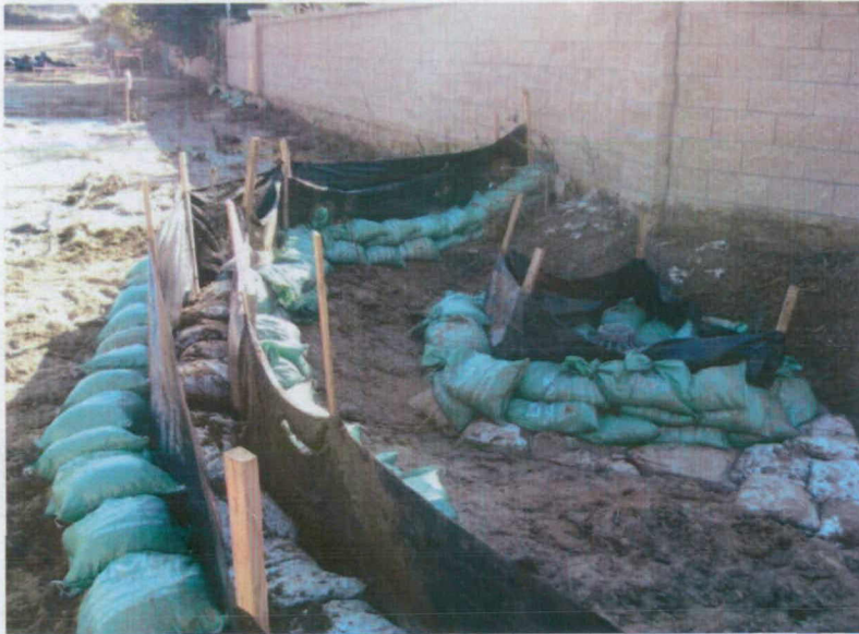
Photo 7: Inundated storm drain inlet. Green gravel bags and two outer silt fences were installed after the December 13, 2012 discharges.
