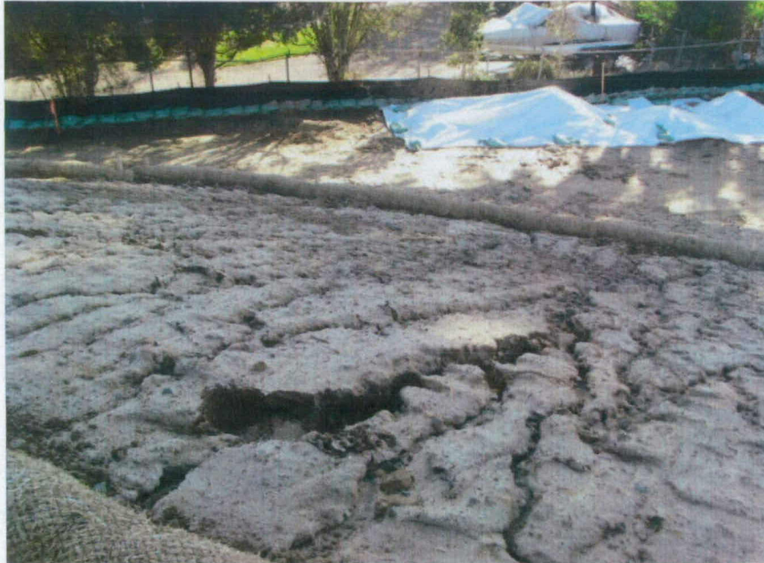
Photo 5: Significant erosion rills leading toward property boundary along Carretta Way.
