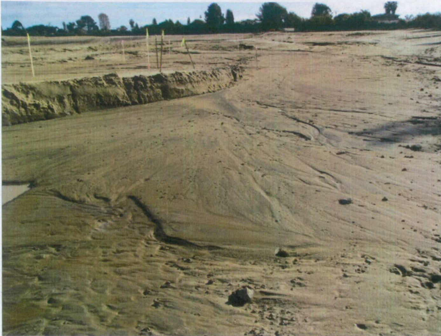
Photo 1: Large graded area with no erosion or sediment controls. Looking south towards Caretta Way.
