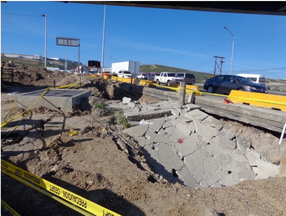
Figure 10 Additional damage along roadway due to collector collapse downstream of junction box- Blvd Lazaro Cardenas, Colonia Los Pirules, Tijuana, B.C. - March 9, 2017
