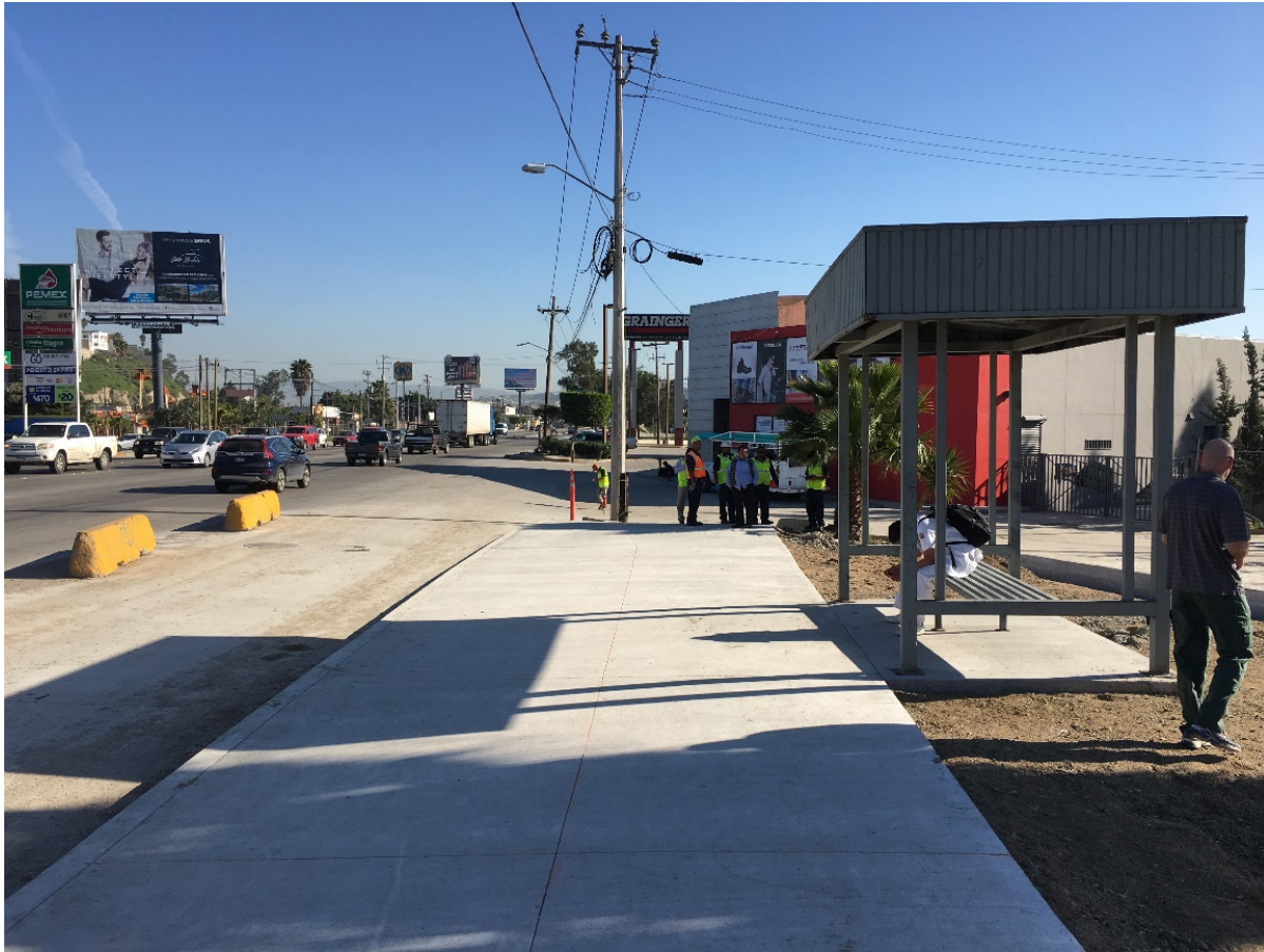
Figure 11 Final repairs to road and bus stop and location of Insurgentes/Oriente collector repair- - Blvd Lazaro Cardenas, Colonia Los Pirules, Tijuana, B.C. - March 9, 2017
