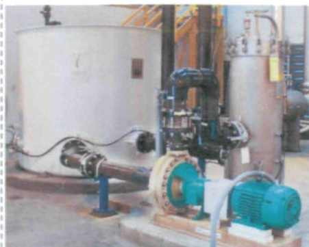
Groundwater demineralization facility
