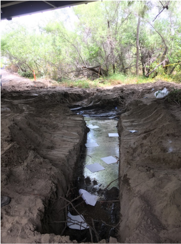
Figure 4: Excavation to remove diesel-impacted soil. Groundwater and diesel fuel are both present in the trench. Absorbent pads in the trench repel water and absorb only the diesel fuel for disposal.
