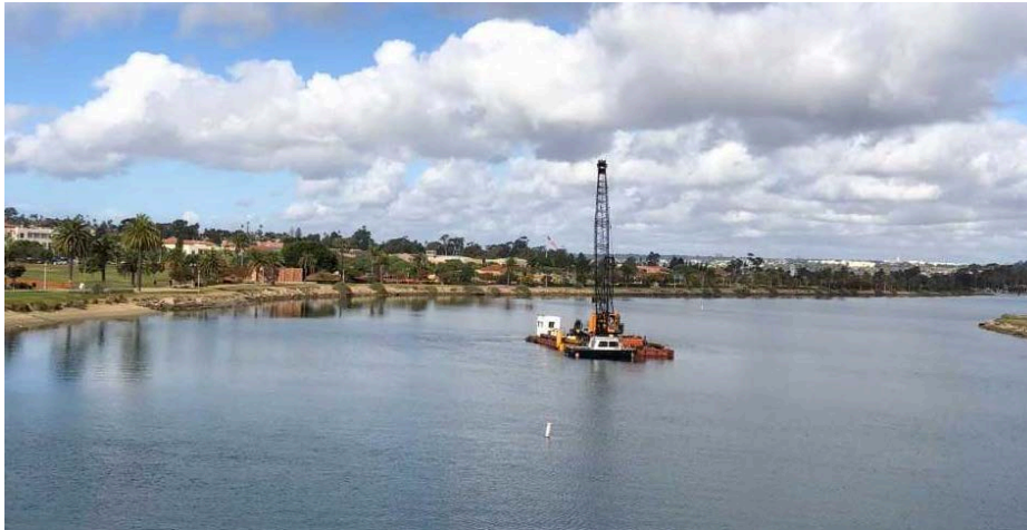
Figure 1: Dredge barge being moved into position in the Former Naval Training Center Boat Channel. (Photo provided by Lynn Dowling)
