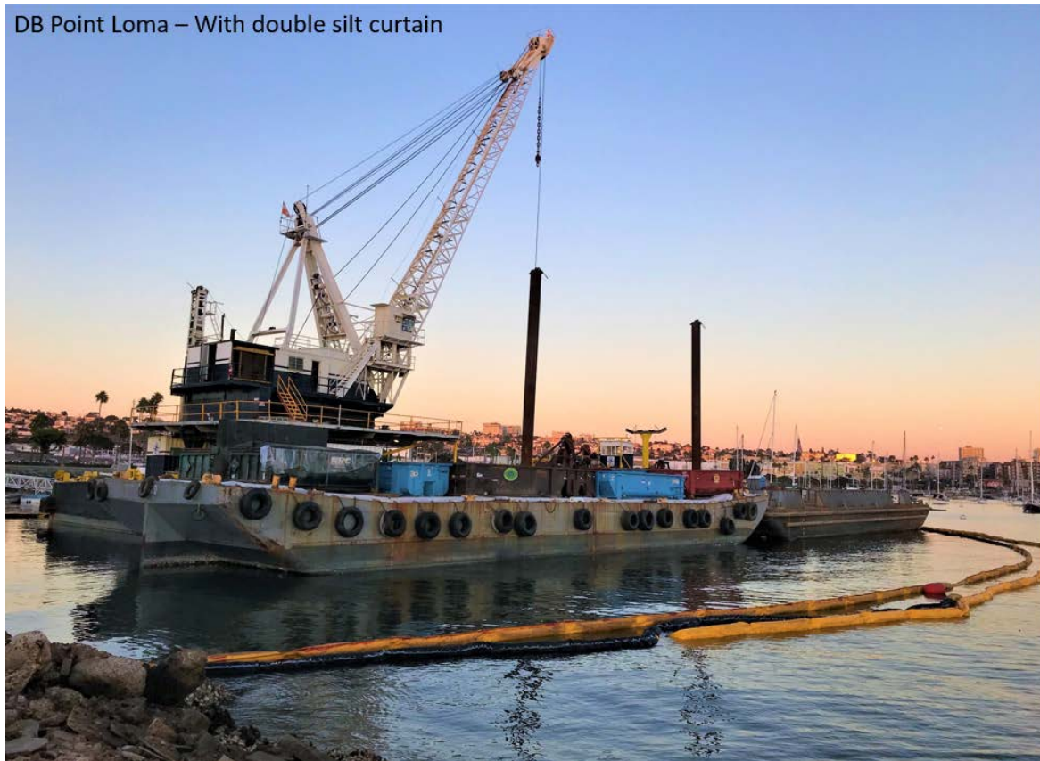
TDY completed dredging the targeted PCB hot spot in the project area. The dredge barge scooped up bay sediment, placed the sediment on the barge to be dewatered and then loaded it into dump trucks to be taken to the Otay Landfill for disposal
