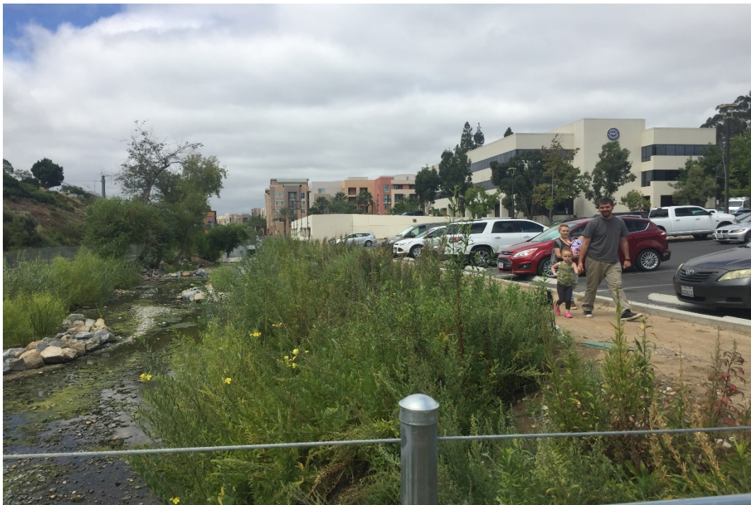
Post-project photo looking downstream- Channel morphology has been redesigned, and non-native vegetation has been replaced with native vegetation.
