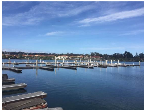
Figure 3: Reinstallation of piles on dock at Marine Corps Recruit Depot. (Photo provided by Department of Navy)
