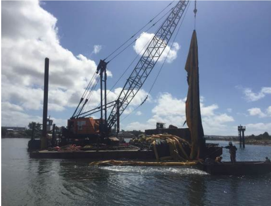
Figure 4: Silt Curtain removal from the Boat Channel (Photo provided by Department of Navy)
