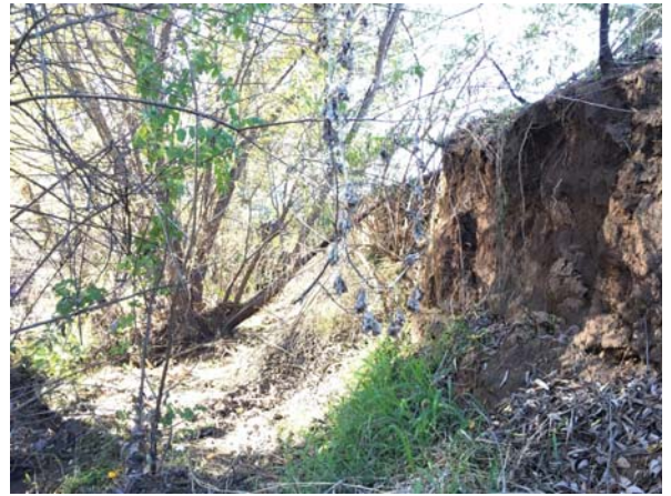
Figure 3. View of right bank at XS2 looking downstream showing highly erodible streambanks typical of the assessment reach.
