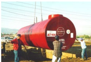
Underground storage tank
